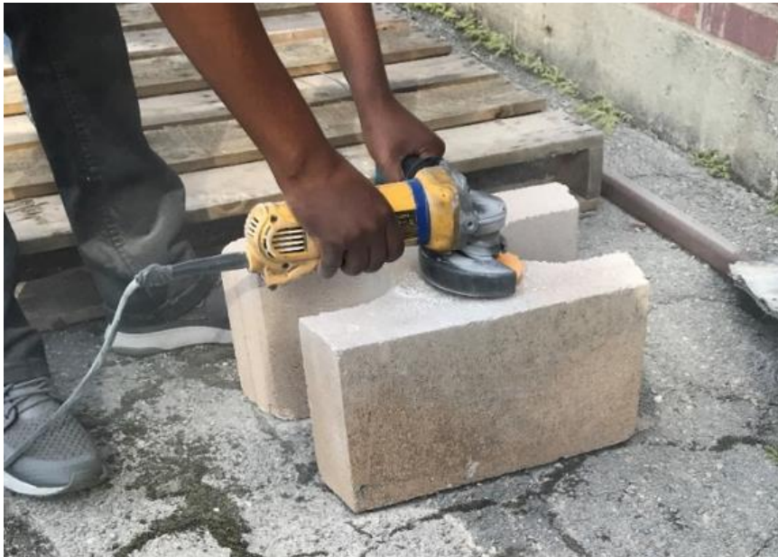
Grinding the lug off the tops of the Vertica straight face block
