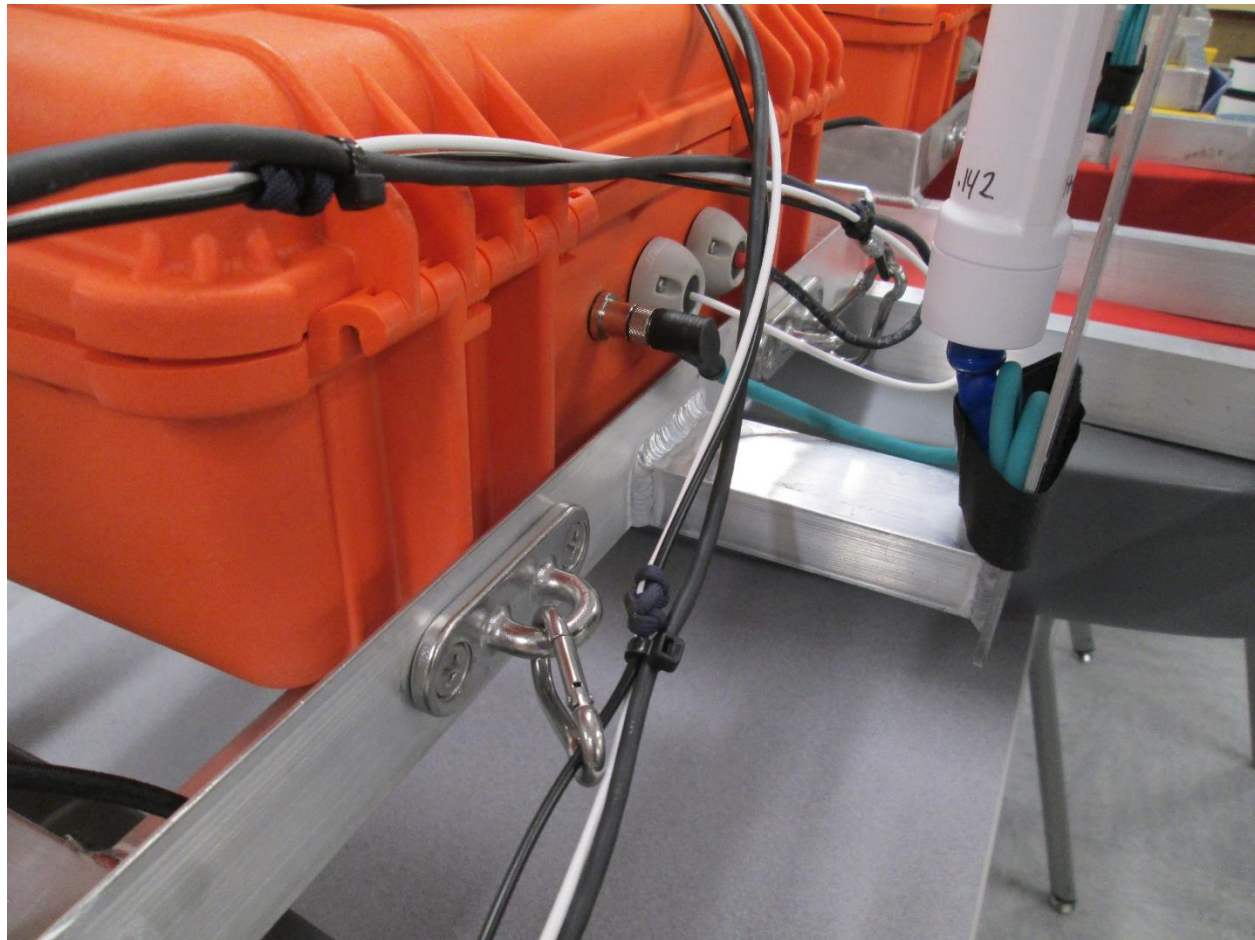
Bulkhead connections through box and strain relief
