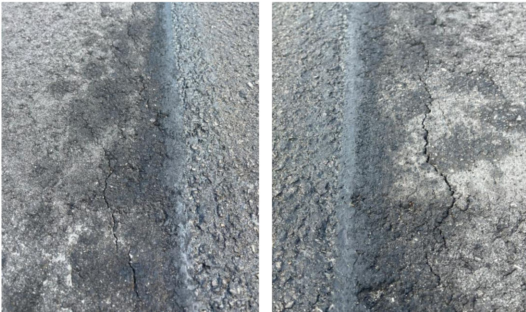
Figure 10. Longitudinal cracks along the edge of HVS wheel-path on scabbing section
