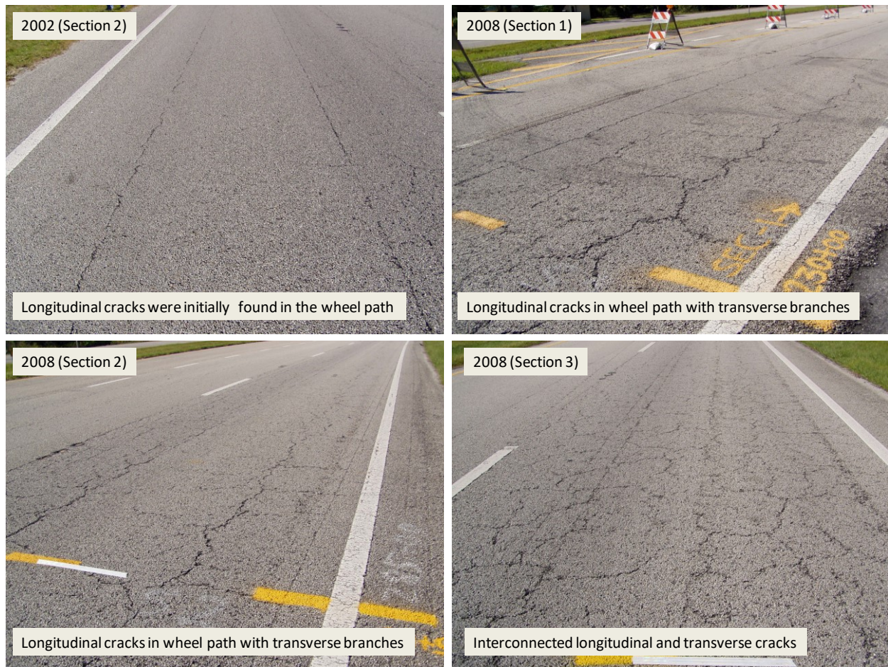
FIGURE 8 Pavement cracking trends: longitudinal crack in the wheel path initially.
