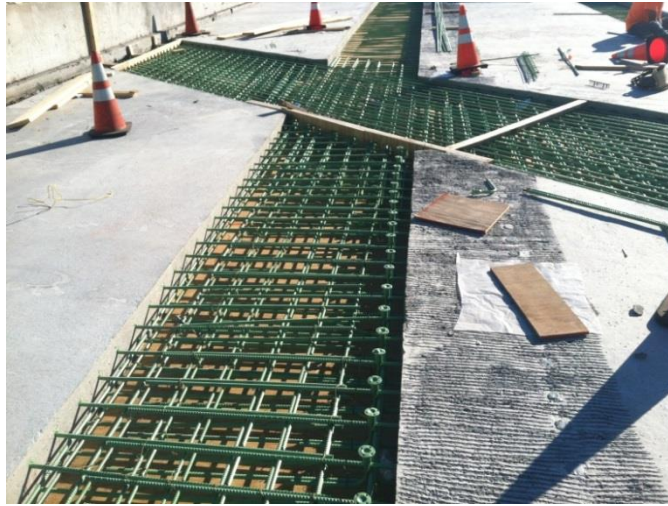
Figure 8.42 Link Slab Construction Showing New Slab Over the Pier and Link Slab Over the Girders
