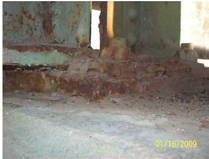
Figure 8.14 Damage to Bearings – Major Deterioration
