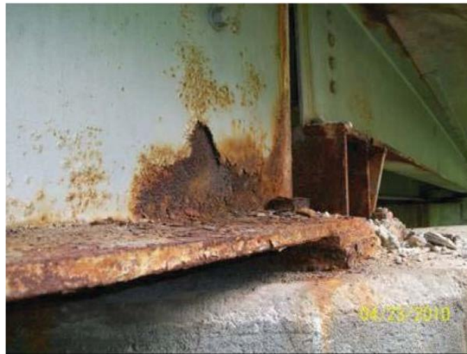
Figure 8.15 Damage to Steel Beam Ends – Major Deterioration
