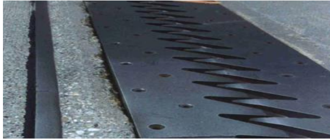
Figure 8.31 Damaged Finger Joint
