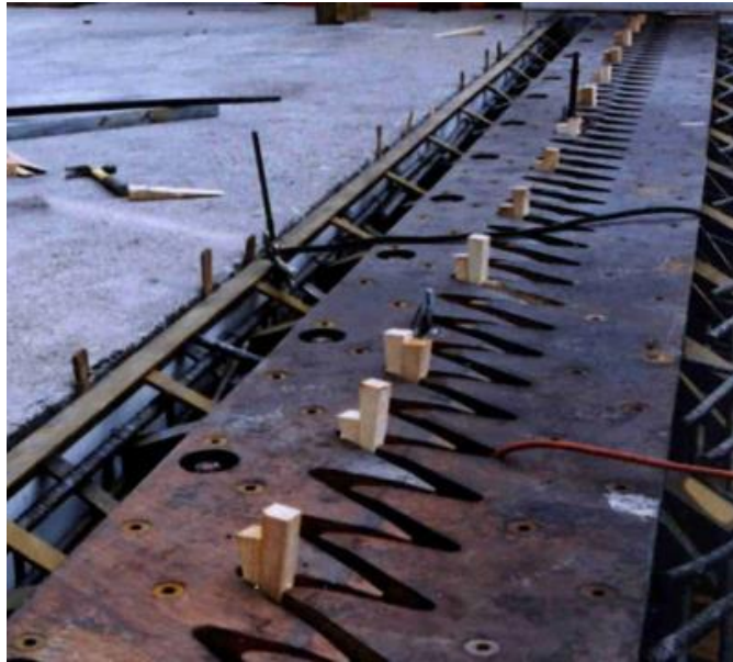
Figure 8.34 Shims Used to Provide Proper Joint Spacing Prior to Casting the Joint
