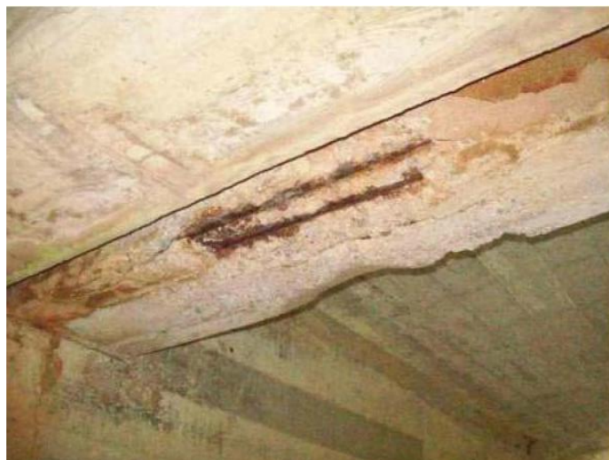
Figure 8.16 Damage to Concrete End Diaphragms – Major Deterioration
