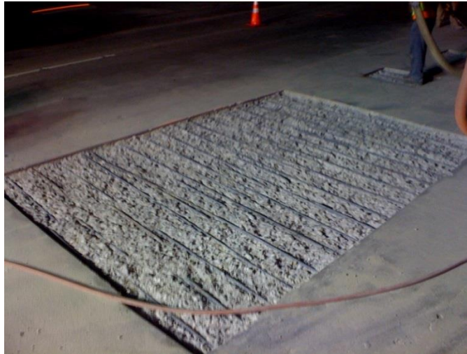
Figure 7.28 Sawcut, Chipped Out and Cleaned (Courtesy of Truesdell Construction) Concrete Removal Shown to the Top Mat Only
