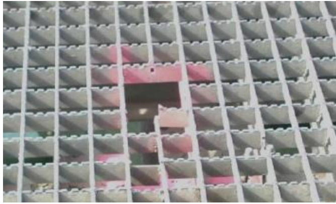
Figure 7.44 Typical Broken Grid Section
