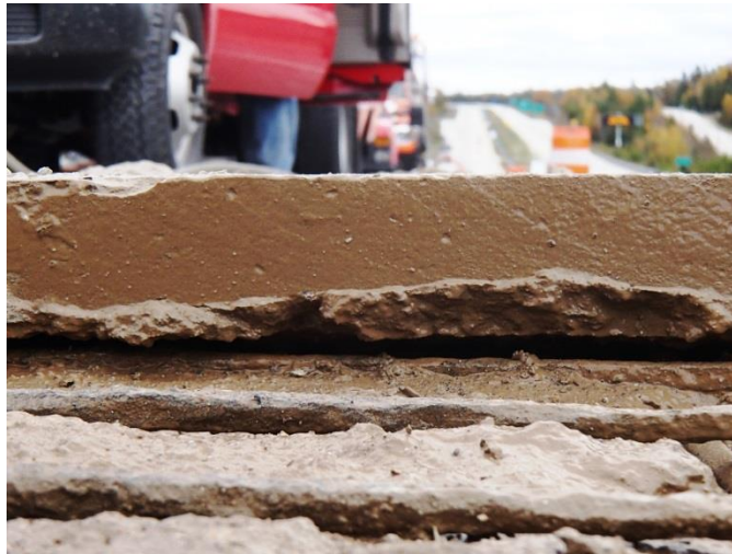
Figure 7.20 Delamination at Edge of Patch (Courtesy of MDOT)
