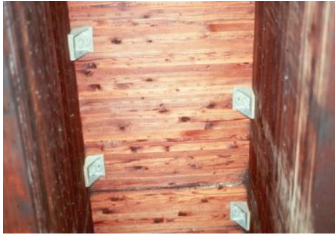
Figure 7.47 Glulam Members Attached with Metal Clips
