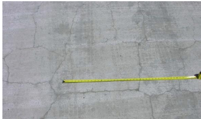
Figure 7.7 Typical Widespread Cracking Pattern on a Bridge Deck (Courtesy of Virginia DOT)
