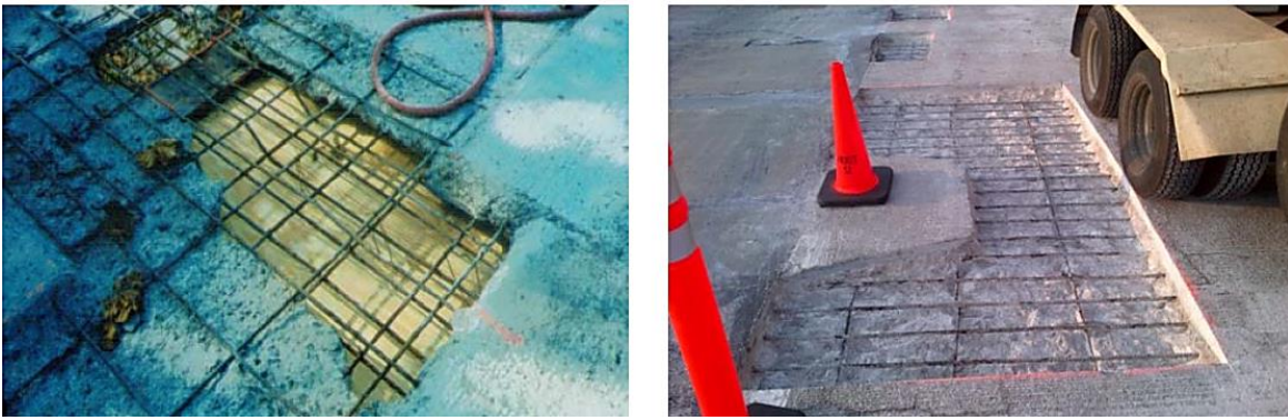
Figure 7.16 Concrete Repair Photos. Full Depth Repair (left) and Partial Depth Repair (right)
