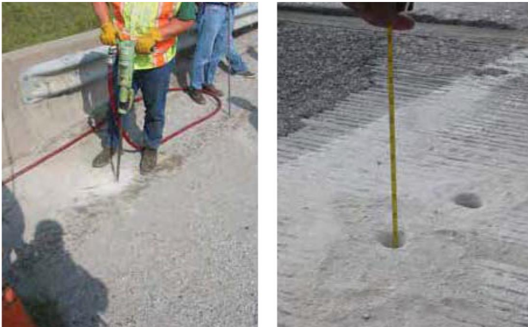
Figure 6.6 Drilling through the Approach Slab (left). Measuring the Depth of the Void (right). (Courtesy of Iowa DOT)
