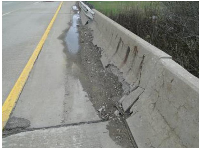
Figure 6.15 Crushed Barrier due to Approach Pavement Growth (Courtesy of MDOT)
