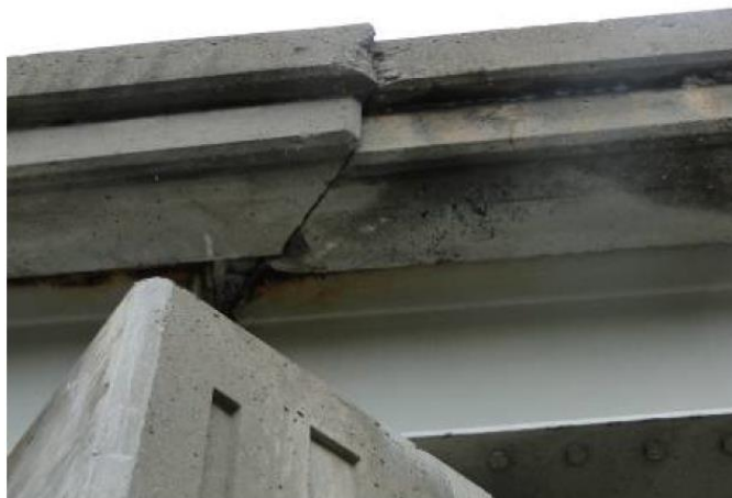
Figure 6.14 Expansion Joint Permanently Closed due to Approach Pavement Growth (Courtesy of MDOT)
