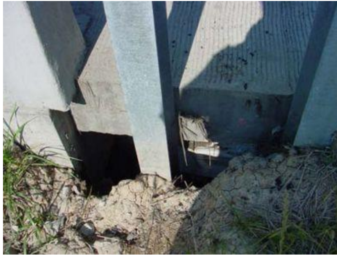
Figure 6.5 Void under Approach Slab (Courtesy of Missouri DOT)
