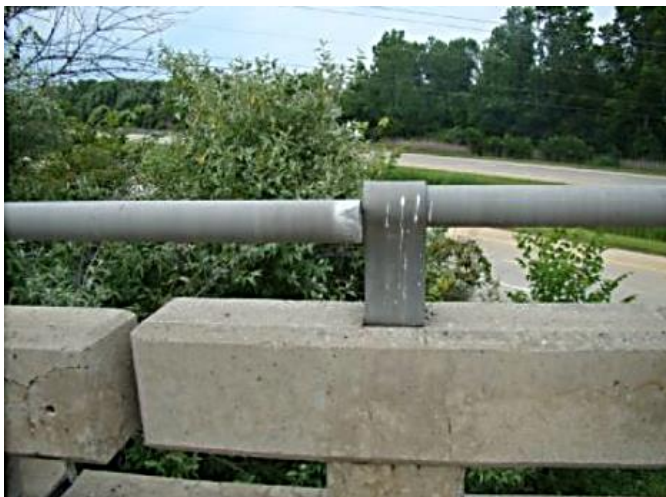
Figure 6.16 Aluminum Tube Rail Separation, a Possible Sign of Approach Pavement Growth (Courtesy of MDOT)
