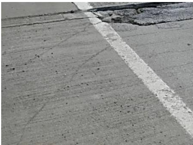
Figure 6.17 Diagonal Deck Cracking May be a Sign of Approach Pavement Growth (Courtesy of MDOT)
