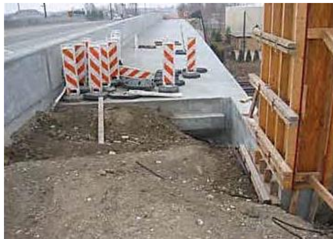
Figure 6.3 Non-Compacted Granular Backfill Behind a Bridge Abutment (Courtesy of Iowa DOT)
