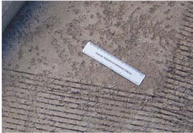
Figure 5.6 Scaling on a Bridge Deck (Courtesy of Iowa State University)
