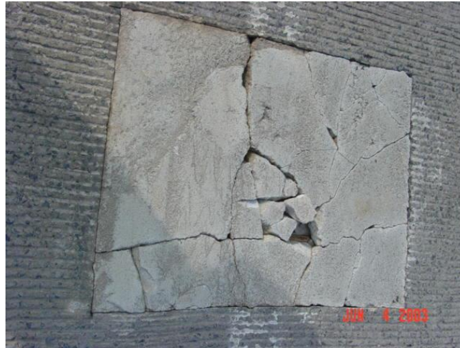
Figure 5.54 Failure of Rapid-Setting Mix
