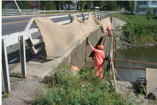
Figure 5.71 Preparing for the Cure of the Repair of a Concrete Fascia Beam Repair
