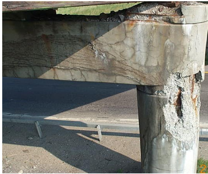
Figure 5.35 Severely Deteriorated Concrete Pier
