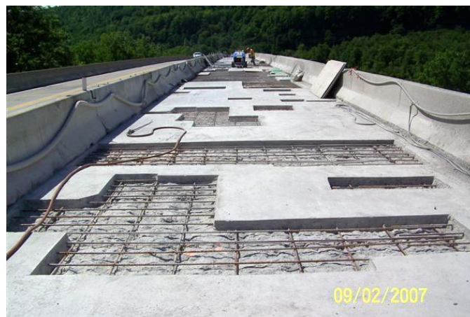
Figure 5.43 Extensive Patching on a Bridge Deck
