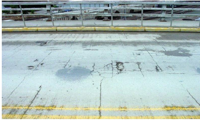
Figure 5.10 Spalls and Cracking
