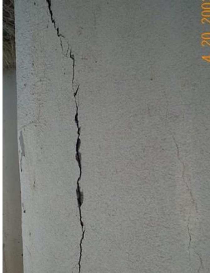
Figure 5.3 Vertical Crack on a Pier Column
