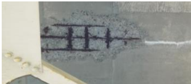
Figure 5.11 Spalled Concrete and Efflorescence on the Underside of a Bridge Deck
