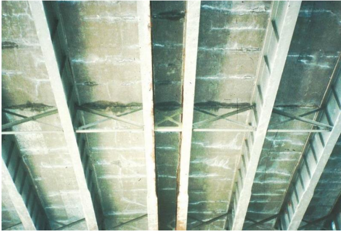
Figure 5.8 Cracking from Thermal Effects
