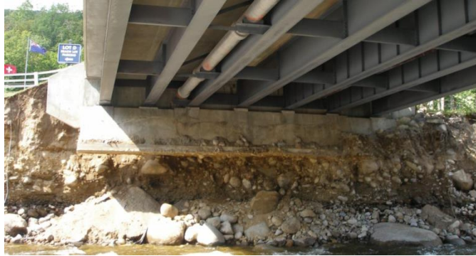
Figure 4.27 Example of Severe Scour (Courtesy New Hampshire DOT)
