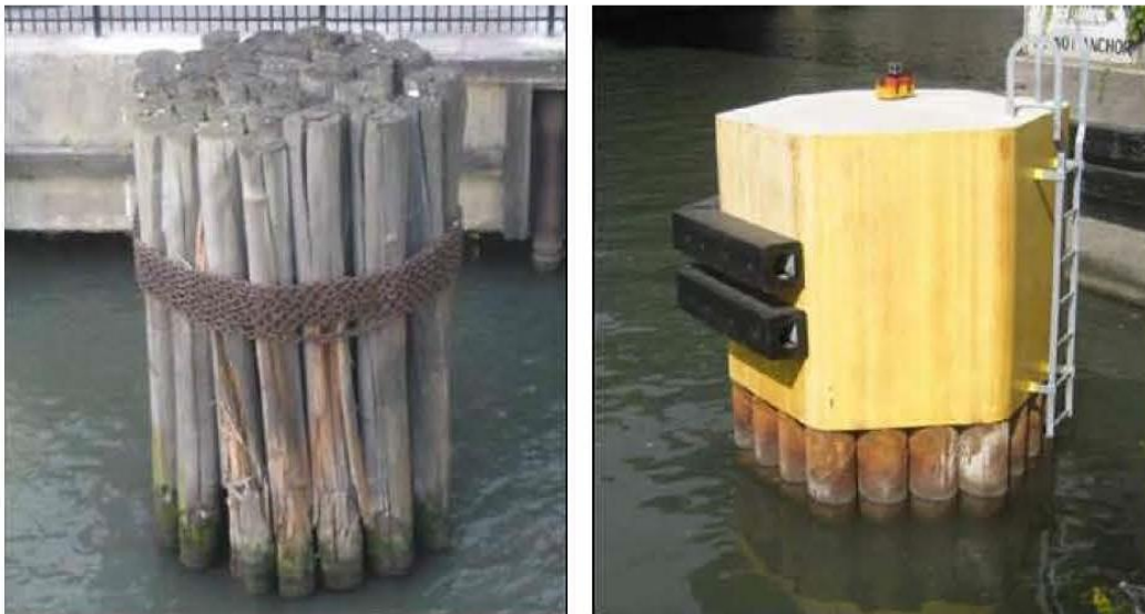
Figure 3.46 Examples of Dolphins. Timber Dolphin (left) and Steel Pipe Pile Dolphin with Concrete Cap (right).
