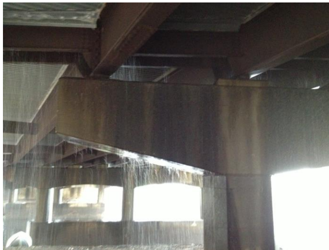
Figure 3.8 Leaky Joints Lead to Problems at Bearings and Pier Caps
