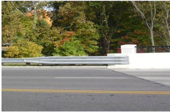
Figure 3.11 Approach Guardrail Transition
