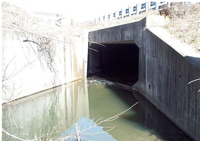
Figure 3.63 Culvert Skewed End
