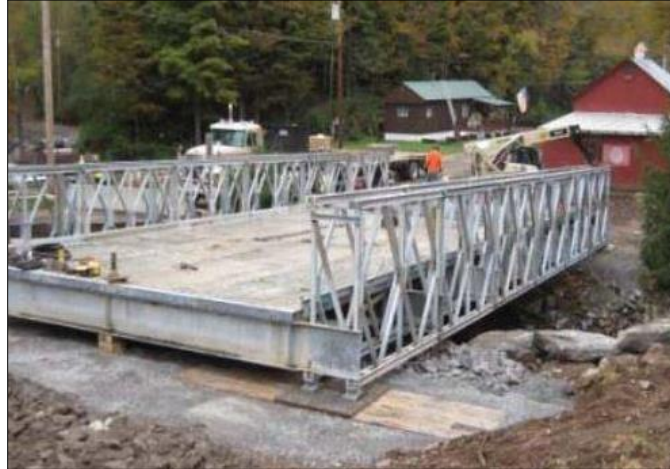
Figure 21.2 Panelized Truss Temporary Bridge with Two Trusses on Each Side of Roadway
