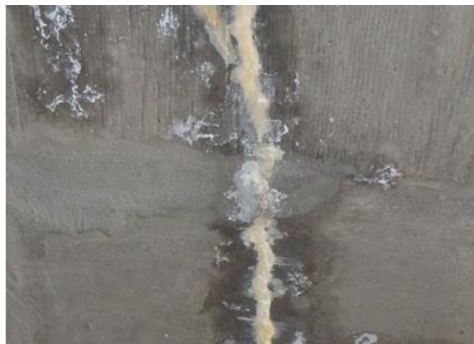
Figure 20.10 Typical Soffit Crack with Efflorescence
