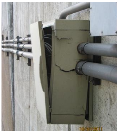
Figure 19.14 Signs of Damage Should Be Fixed to Prevent Electrical Shock
