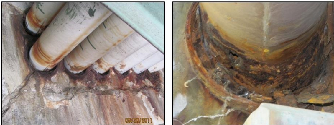
Figure 19.12 Examples of Corrosion at Exposed Gas Pipe
