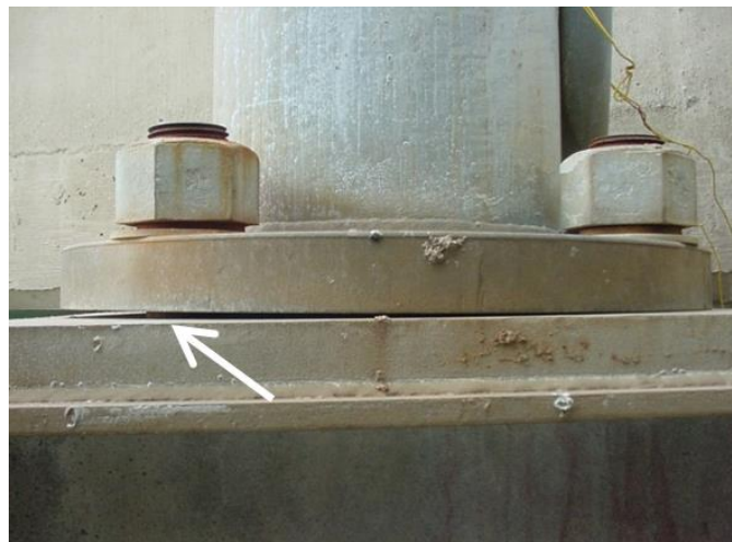
Figure 19.24 Loose Anchor Bolts Revealed by Gap Under the Base Plate
