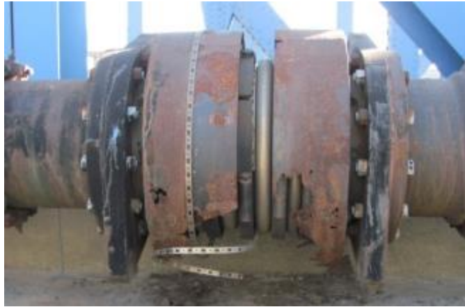
Figure 19.16 Example of Damaged Supports Requiring Attention
