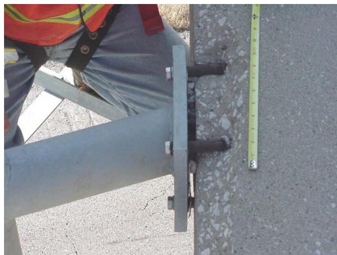
Figure 19.27 Epoxy Anchorage Failure
