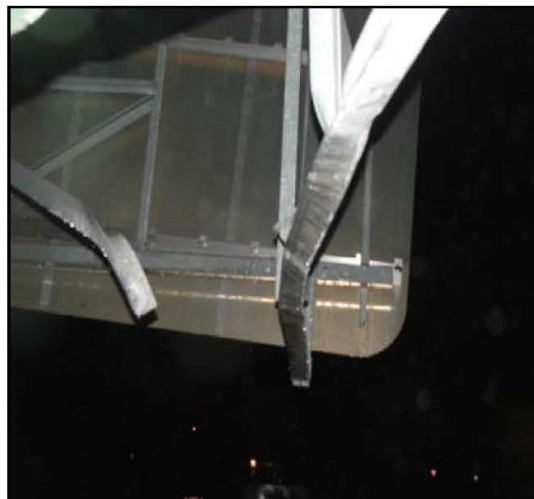
Figure 19.30 Examples of Impact Damage to Sign System Elements
