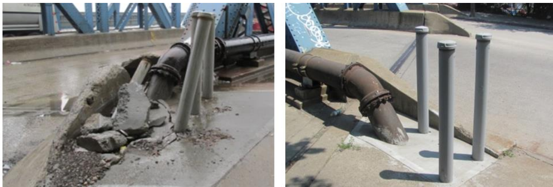
Figure 19.18 Example of Incidental Damage (left) and Resultant Repair (right)
