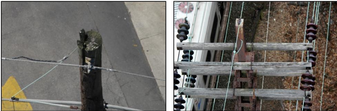
Figure 19.17 Examples of Cracked and Splintered Wood Poles (left) and Supports (right)
