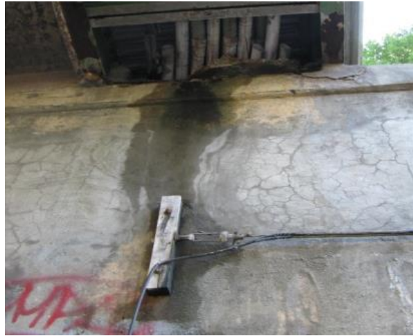
Figure 19.13 Water Leakage under Bridge Structure
