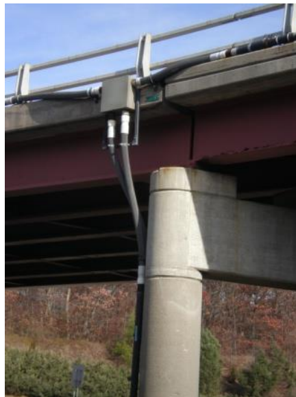
Figure 19.3 Communication Lines Encased in Protective Conduit
