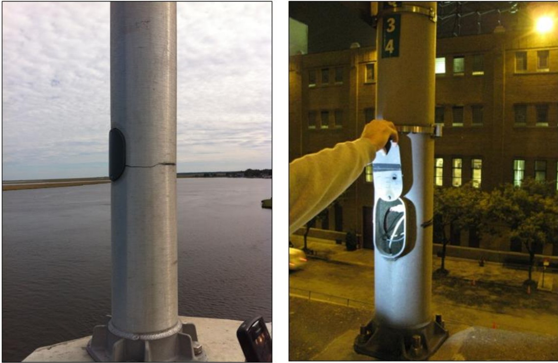
Figure 19.29 Examples of Potential Areas for Fatigue Cracking in Aluminum Light Poles
