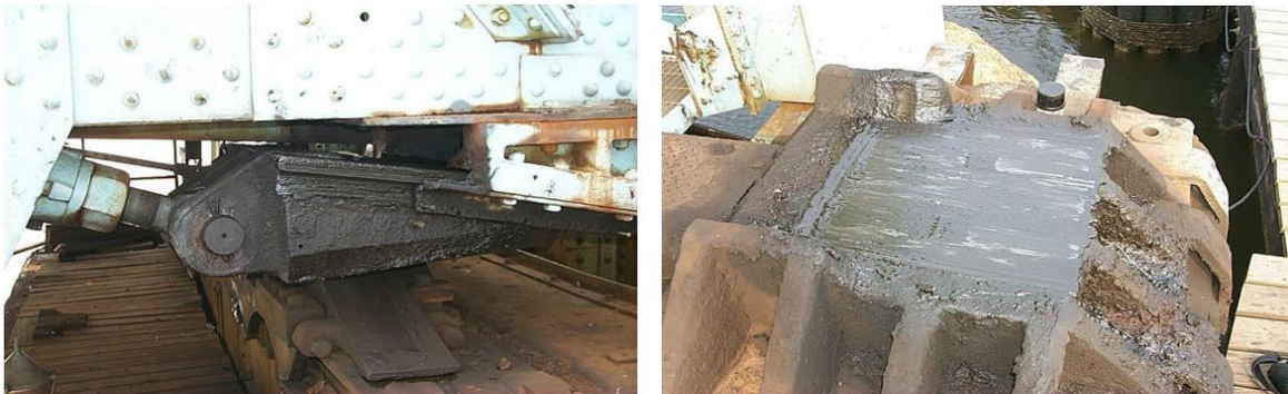
Figure 17.14 Live Load Wedges and Shoes Closed Position with Wedge (left). Live Load Shoe (right).
