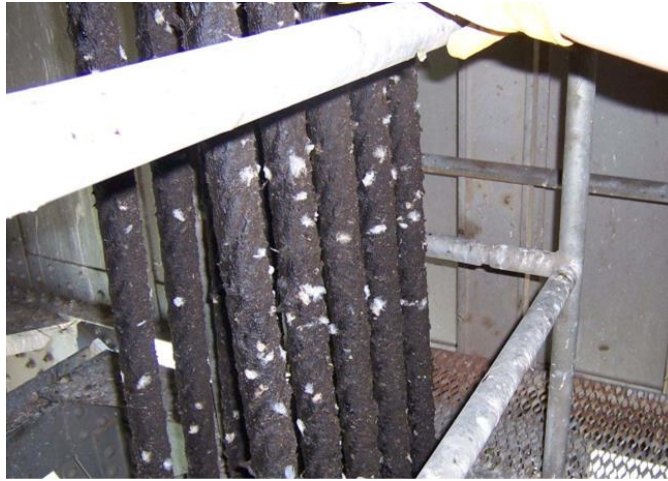
Figure 17.102 Fouled Wire Ropes (Courtesy of California Department of Transportation)
