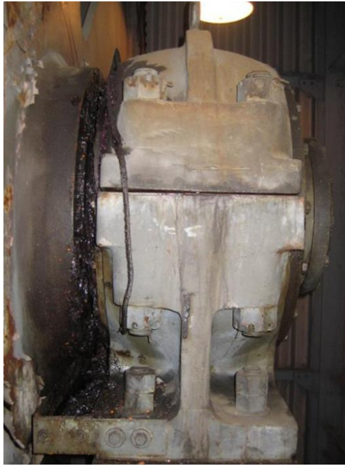
Figure 17.98 Trunnion Bearing with Broken Seal Due to Excessive Lubrication
