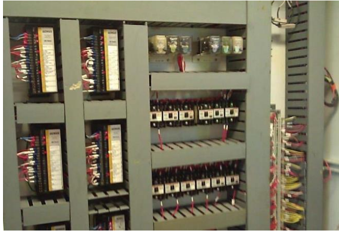
Figure 17.59 I/O Blocks Controlled by the PLC (Courtesy of NHDOT)
