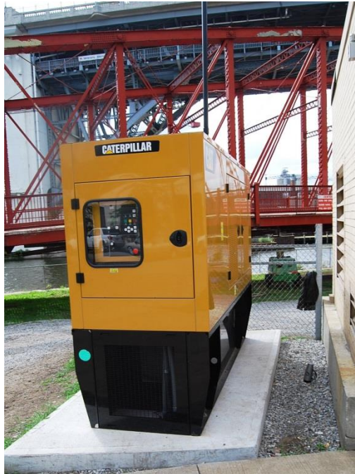
Figure 17.95 Exterior Grade Auxiliary Generator
