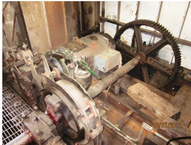
Figure 17.20 Open Gearing Operating Machinery
