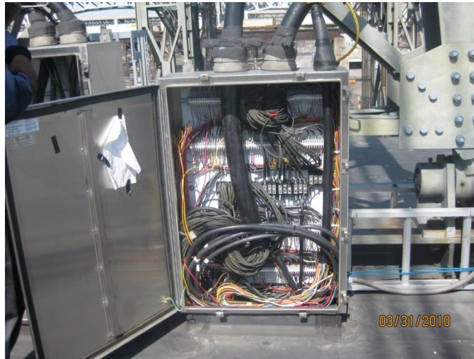
Figure 17.93 Aerial Cable Junction Box Where the Aerial Cables have Slipped
