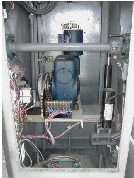
Figure 17.63 Drive Motor Cabinet for Resistance Gate (Courtesy of MaineDOT)
