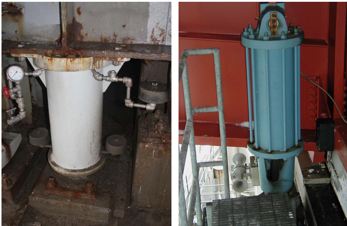
Figure 17.25 Air Buffers in the Retracted (left) and Not Retracted (right) Positions (right - Courtesy of MaineDOT)
