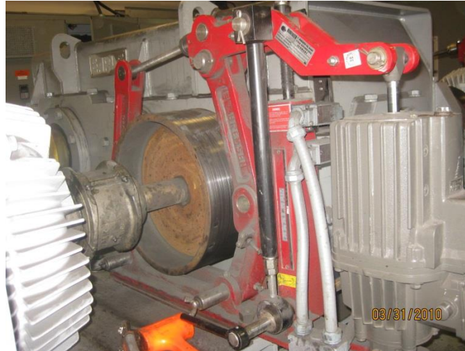
Figure 17.79 Brake Assembly Exhibiting Moderate Brake Dust Accumulation
