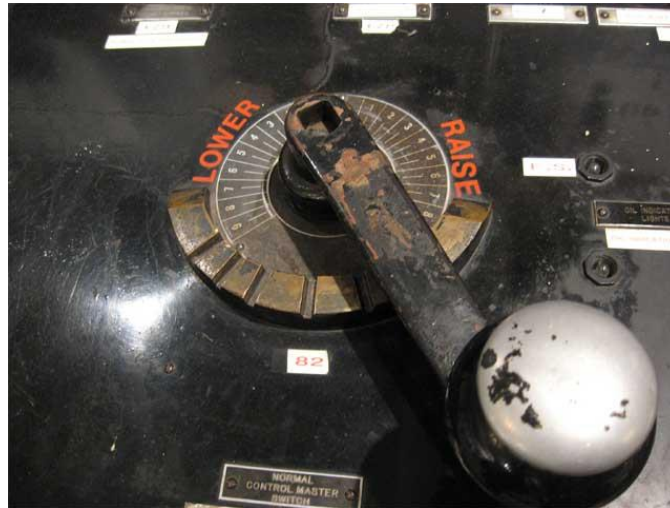
Figure 17.57 Drum Switch to Control Motor Speed and Direction (Courtesy of Brian D. Luster)
