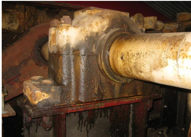
Figure 17.77 Leaking Sleeve Bearing
