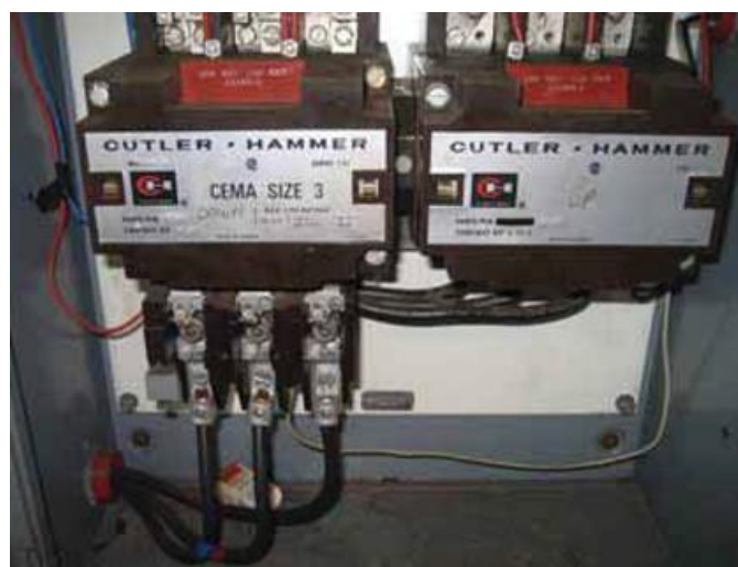
Figure 17.56 Drive Motor Contactor
