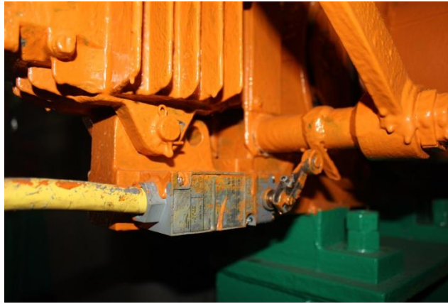
Figure 17.70 Painted Over Limit Switch on Brake Assembly
