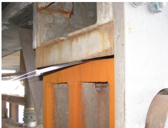
Figure 17.83 Fixed Live Load Support Bearing Not Fully Engaged in Seated Position
