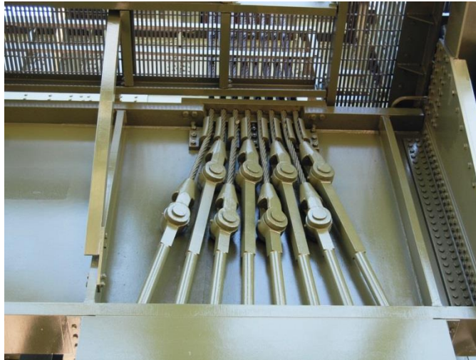
Figure 17.100 Wire Rope Sockets and Fittings at Lifting Girder
