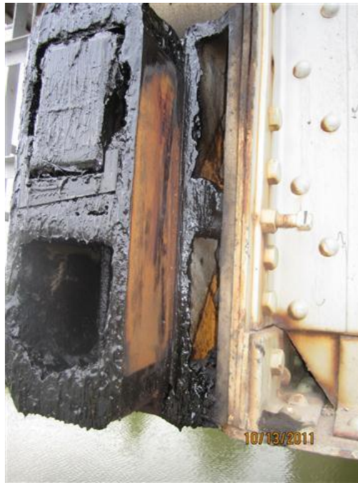
Figure 17.81 Span Lock Rusting due to Aged and Contaminated Lubrication
