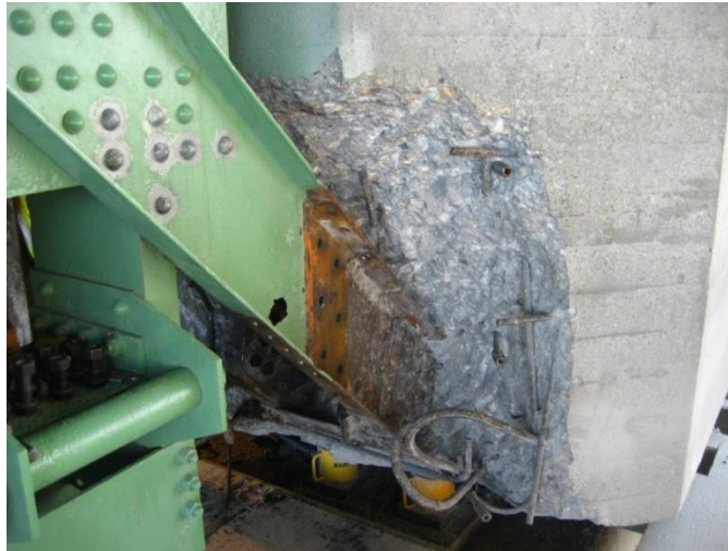
Figure 17.82 Section Loss Repair of Steel Frame Connection with the Counterweight
