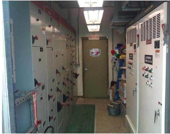
Figure 17.52 Motor Control Center (MCC) (Courtesy of NHDOT)
