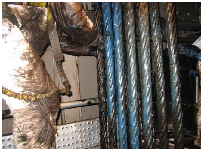
Figure 17.101 Lubricating Wire Ropes (Courtesy of California Department of Transportation)
