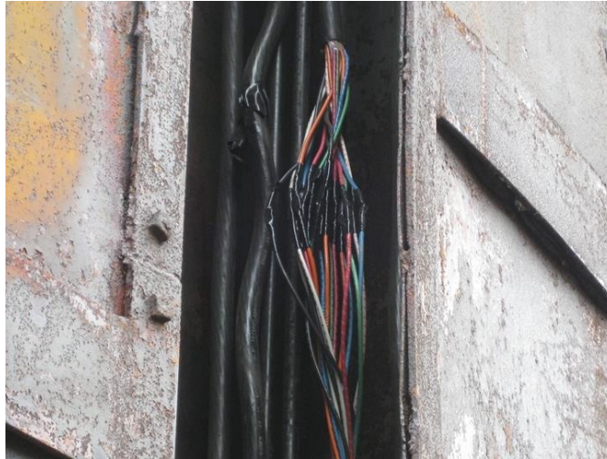
Figure 17.90 Twisted Droop Cable with Exposed Wiring
