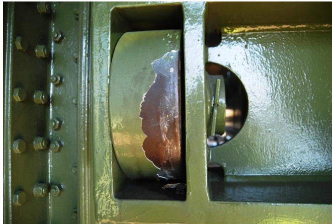
Figure 17.86 Painted Over Span Guide Roller Impeding Free Rotation
