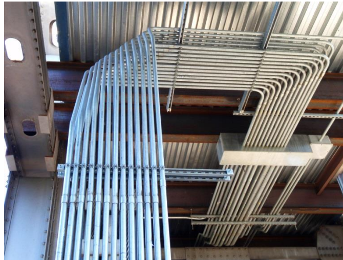
Figure 17.53 Example of Electrical Conduit Work Under a Bridge (Courtesy of Kyle Asfahl)
