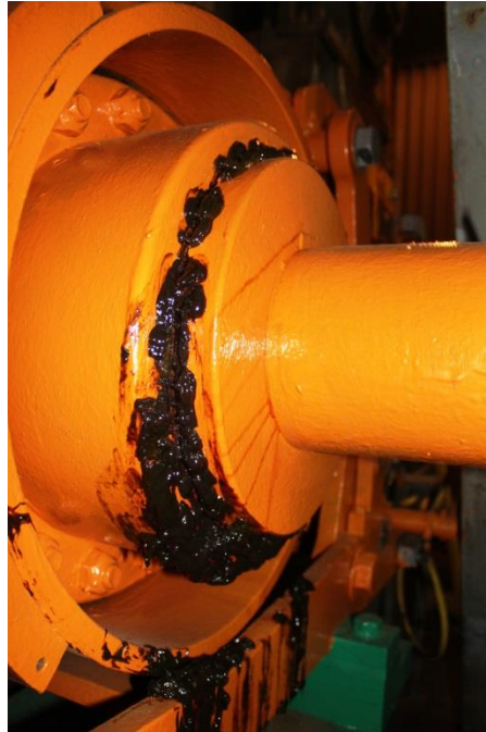
Figure 17.75 Leaking Gear Coupling
