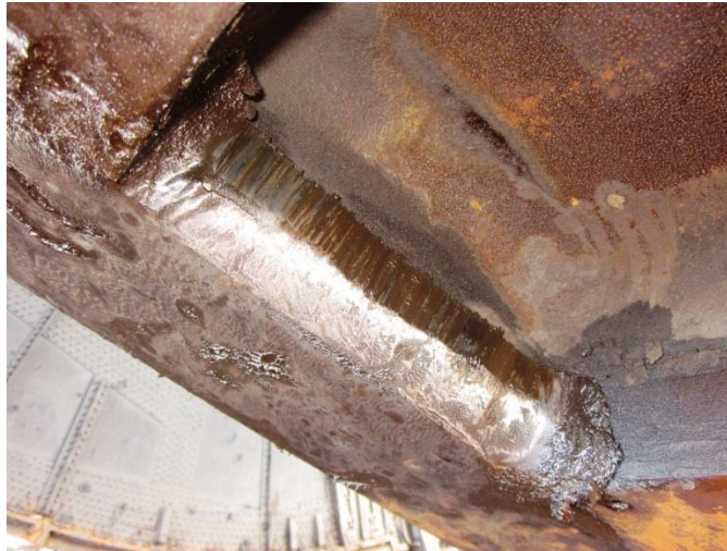
Figure 17.88 Excessive Wear of Curved Tread Plate Pocket
