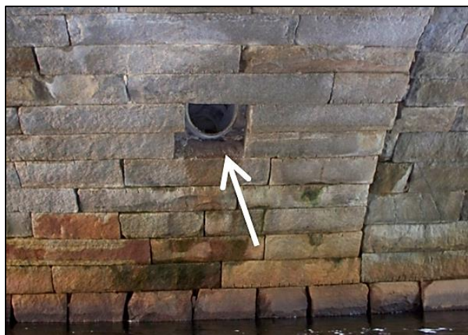
Figure 16.17 Missing Stones in a Masonry Arch
