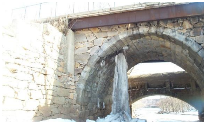
Figure 16.26 Evidence of Water Infiltration
