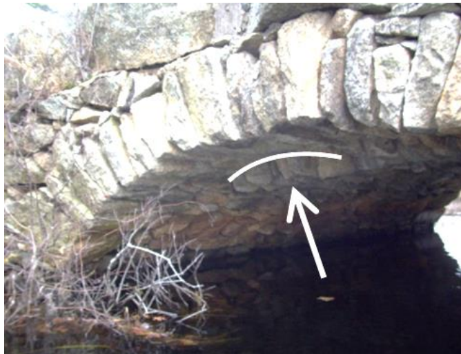
Figure 16.15 Multiple Slipped Stones
