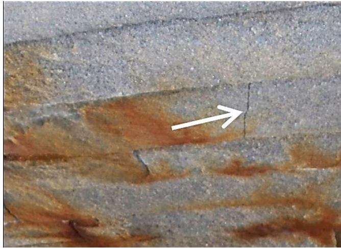
Figure 16.14 Transverse Crack in Stone Arch
