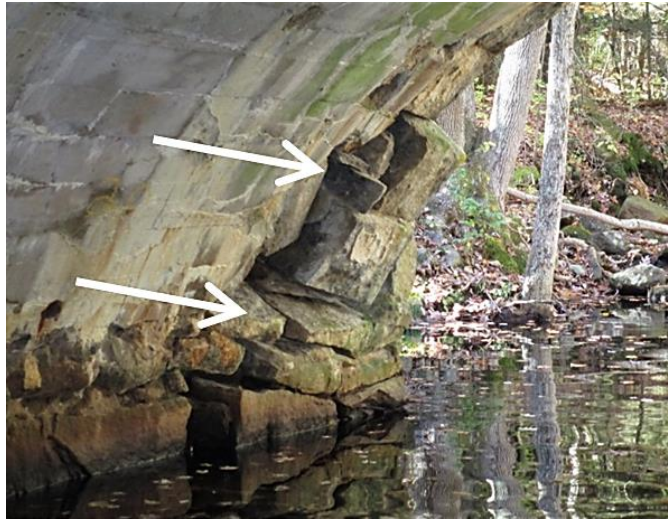
Figure 16.18 Arch Deformation caused by Masonry Displacement
