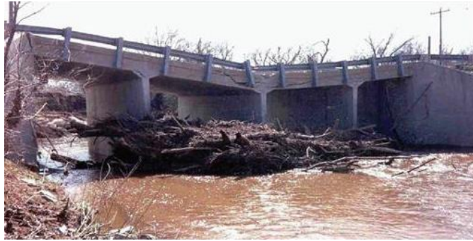
Figure 15.6 Increased Scour at Bridge Piers as a Result of Debris
