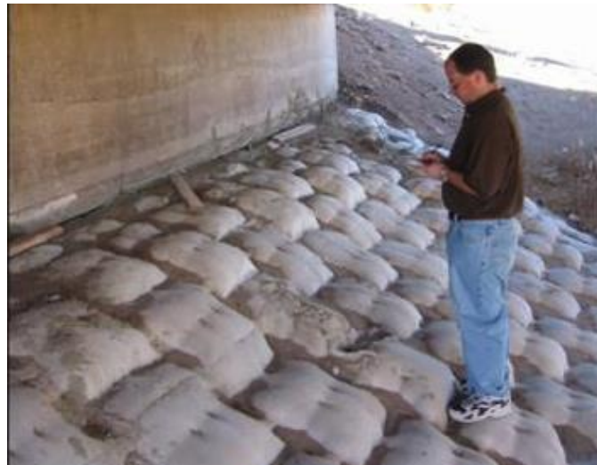
Figure 15.26 Grout-Filled Mat Used for Scour Protection at a Bridge Abutment
