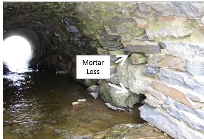
Figure 14.11 Mortar Loss in Bottomless Masonry Arch
