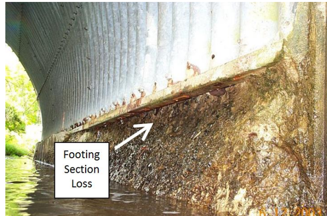
Figure 14.12 Footing Section Loss in Bottomless Culvert
