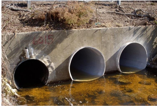
Figure 14.22 A Completed Installation of Cured in Place Pipe (Courtesy of Insituform USA)
