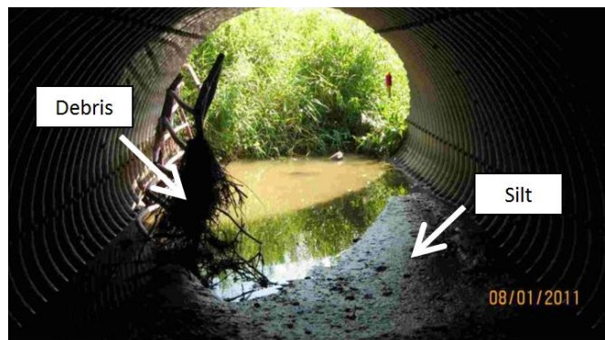
Figure 14.6 Debris and Silt in Corrugated Culvert
