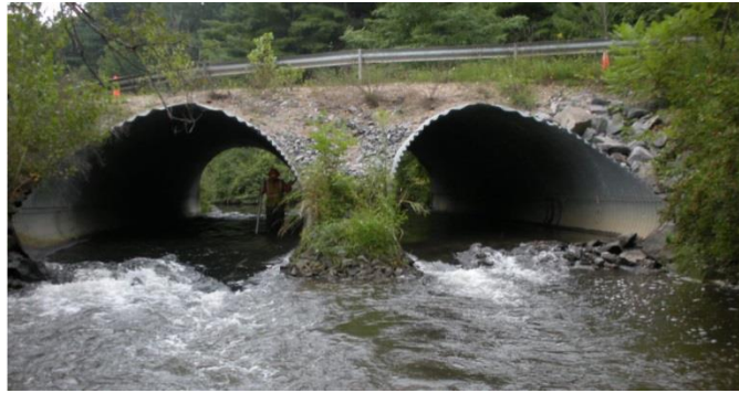
Figure 14.1 Twin Corrugated Metal Plate Pipe Arches
