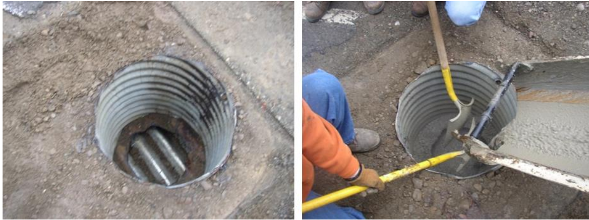
Figure 14.17 Grout Placement Hole Excavated in Road Surface (Courtesy of Washington County NY DPW)
