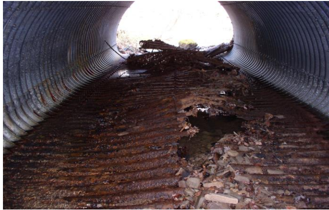
Figure 14.9 Corrosion Failure of Culvert Invert
