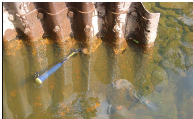
Figure 14.8 Corrosion in Plate Arch
