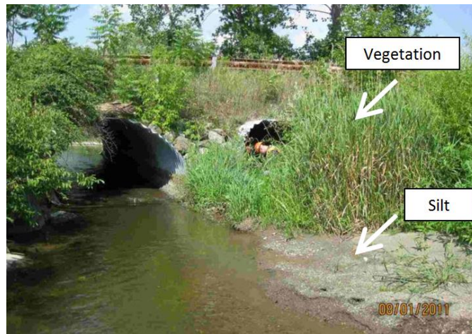
Figure 14.7 Silt and Vegetation Blocking Corrugated Metal Culvert
