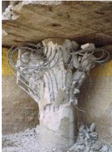
Figure 13.86 Inadequately Confined Column
