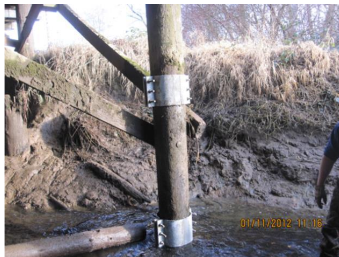
Figure 13.63 Repair to Split Timber Pile Using Steel Clamps (Courtesy of Washington DOT)
