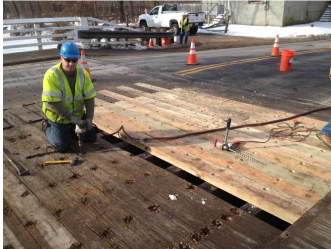
Figure 13.19 New Bridge Replacement Elements Need Surface Treatment
