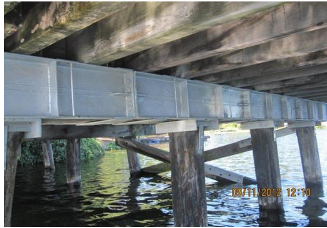
Figure 13.69 Steel Cladding Used to Repair Deteriorated Timber Cap (Courtesy of Washington DOT)
