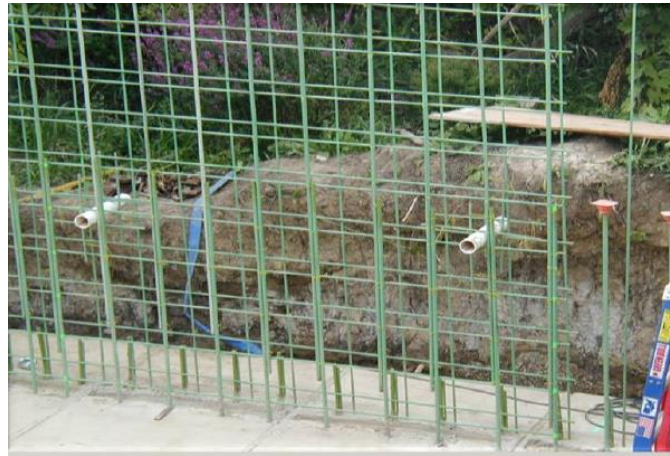
Figure 13.6 Weepholes Consisting of PVC Pipe
