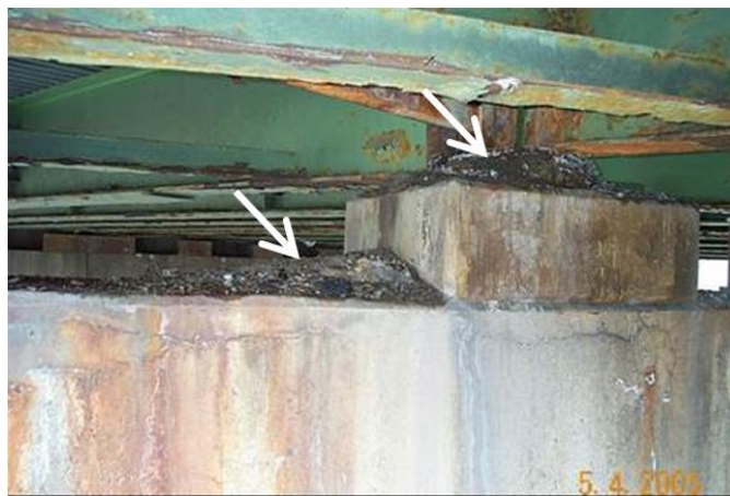
Figure 13.3 Debris on Pedestal and Pier Cap
