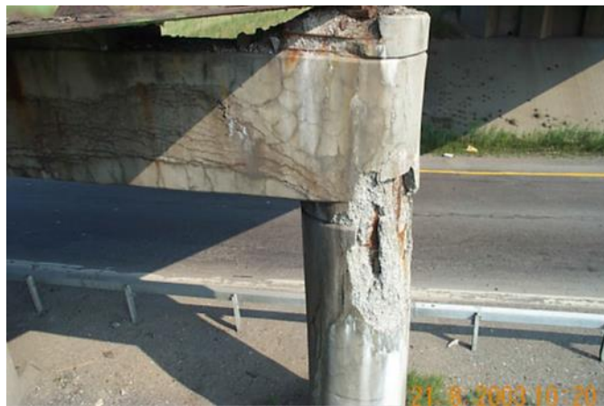
Figure 13.28 Pier Cap and Column in Need of Structural Rehabilitation
