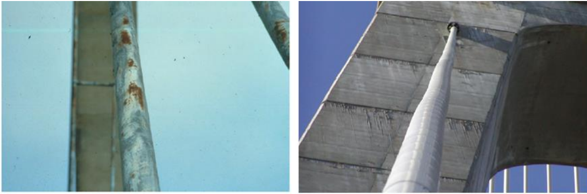
Figure 12.33 Example of Steel Sheathing Deterioration. Corrosion (left) and Bulging (right).
