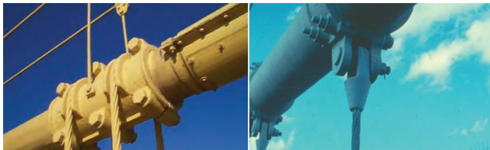
Figure 12.28 Suspender Cable Looped over Cable Band (left) and Suspender Cable with Open Socket Connection (right).
