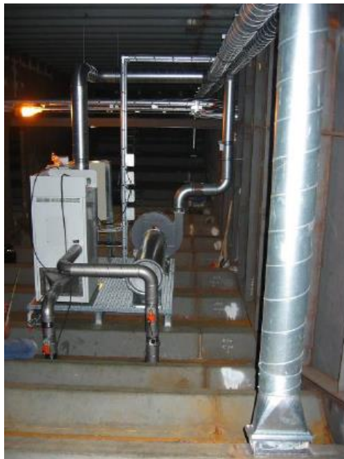
Figure 12.35 Dehumidification Plant (Courtesy of COWI A/S)
