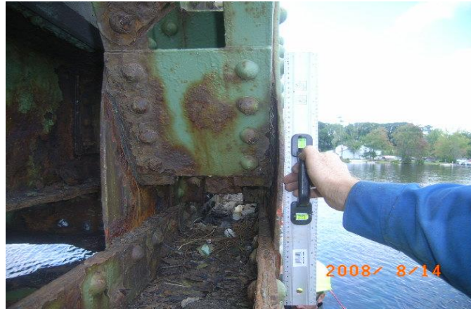
Figure 12.18 Example of Gusset Plate Buckling
