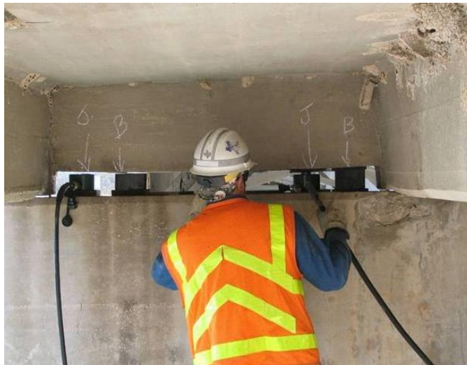
Figure 12.12 Lifted or “Jacked” Superstructure
