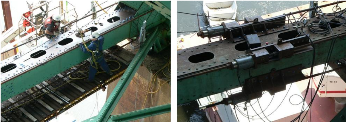
Figure 11.41 Repair of Bottom Chord Plate (left) Utilizing Thread Bars and Jacks (right)
