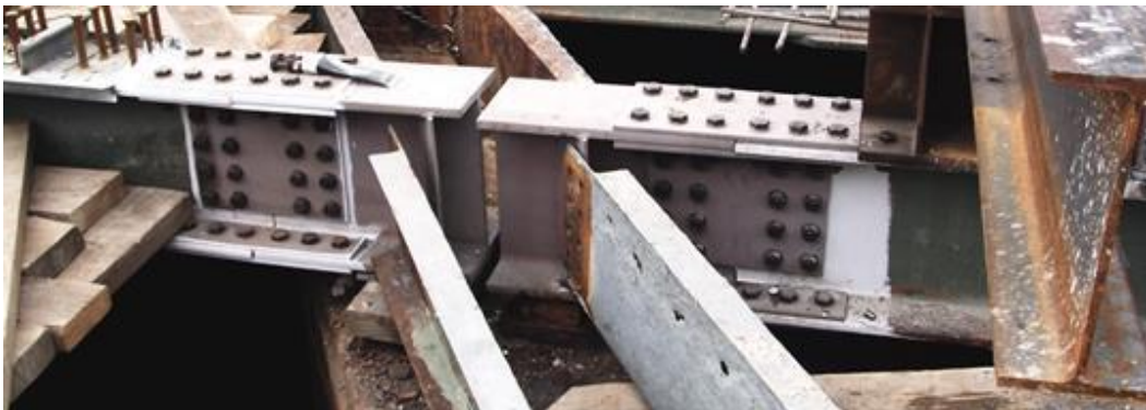
Figure 11.34 Example of a Girder End Repair Utilizing Bolted Splice of a New Full Section
