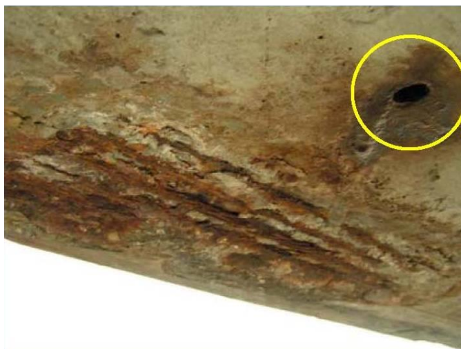
Figure 11.32 Clogged Drains are an Issue
