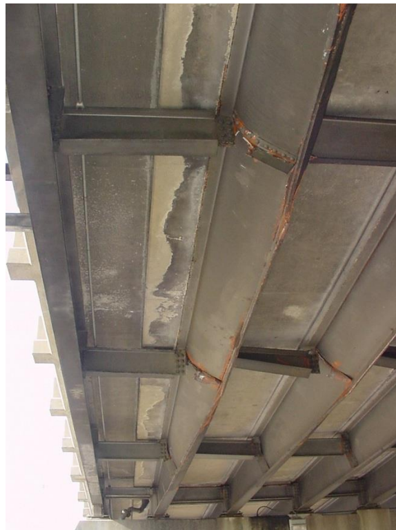
Figure 11.58 Impact Damage to Fascia and First Interior Girder (Courtesy of VDOT)
