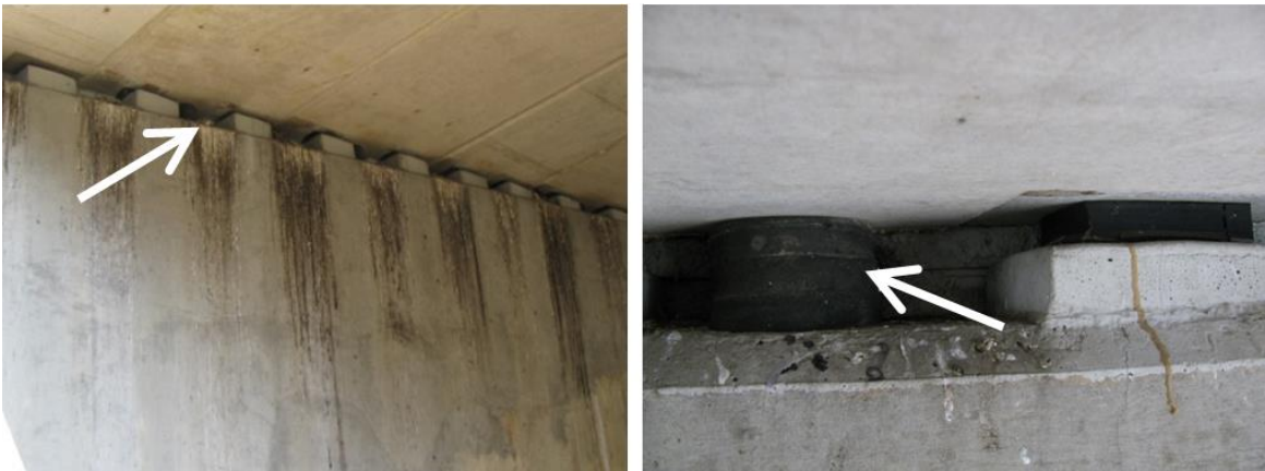
Figure 11.2 Evidence of Bird Nesting (left) and a Rubber Cylinder Deterrent (right)
