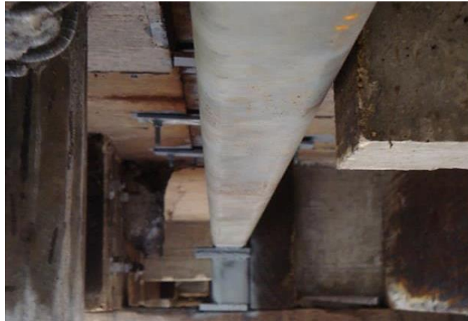
Figure 11.66 Rectangular Steel Section Replacement for Rotten Timber Girder (Courtesy of Washington DOT)
