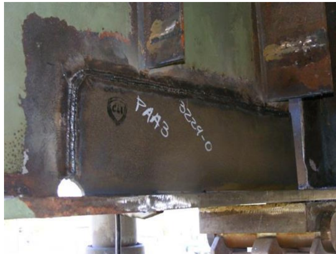
Figure 11.35 Repair in Progress using Tee – Section Cut Out From a Matching W Section
