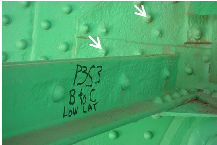
Figure 11.49 Rivet Heads Exhibiting Various Degrees of Corrosion
