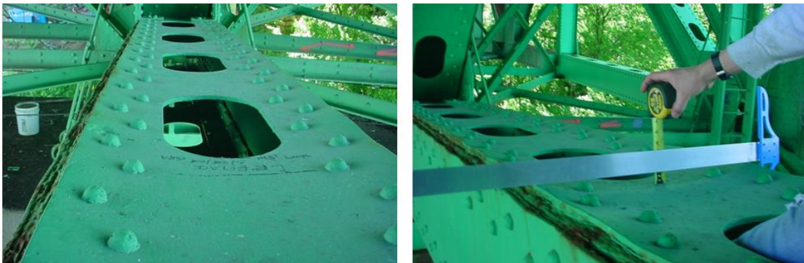
Figure 11.40 Built Up Box Member Corrosion
