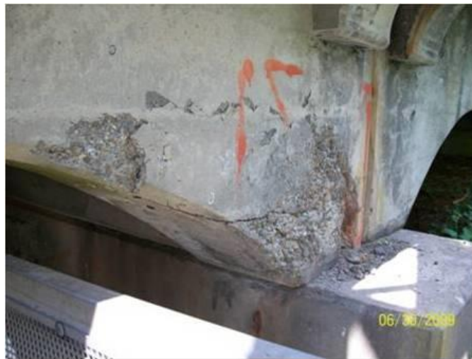
Figure 11.22 Beam End Deterioration
