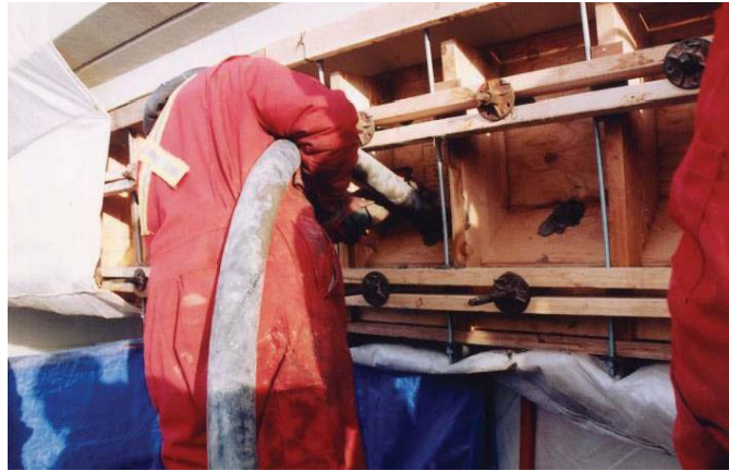
Figure 11.17 Forming Repair. Pumping Concrete into the Form (Courtesy of the Alberta Ministry of Transportation)
