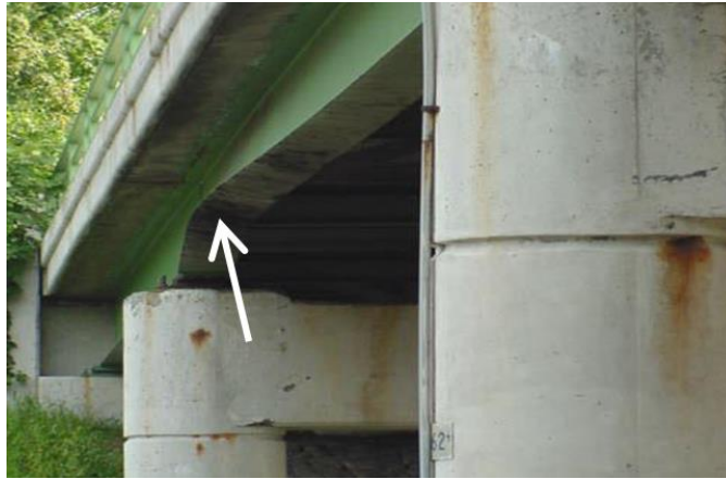
Figure 11.57 Bridge Fascia Girder Damage Caused by Under Passing Vehicle (Courtesy of the New York State Thruway Authority)
