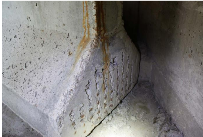
Figure 11.1 Exposed Strands on End of Precast Prestressed Concrete Girder
