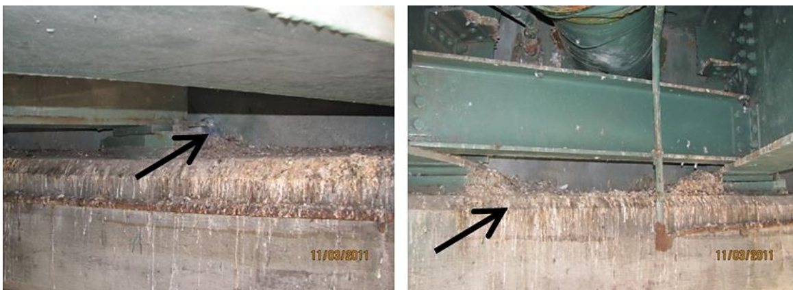
Figure 11.5 Bird Nesting Signs on Steel Superstructure (left) and Behind Steel Girder (right)
