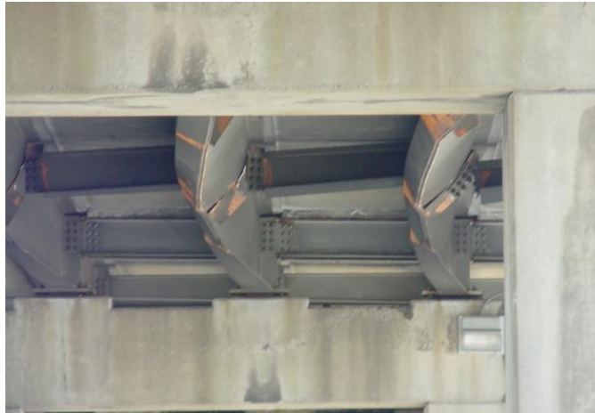
Figure 11.59 Impact Damage that can be Repaired with Heat Straightening (Courtesy of VDOT)
