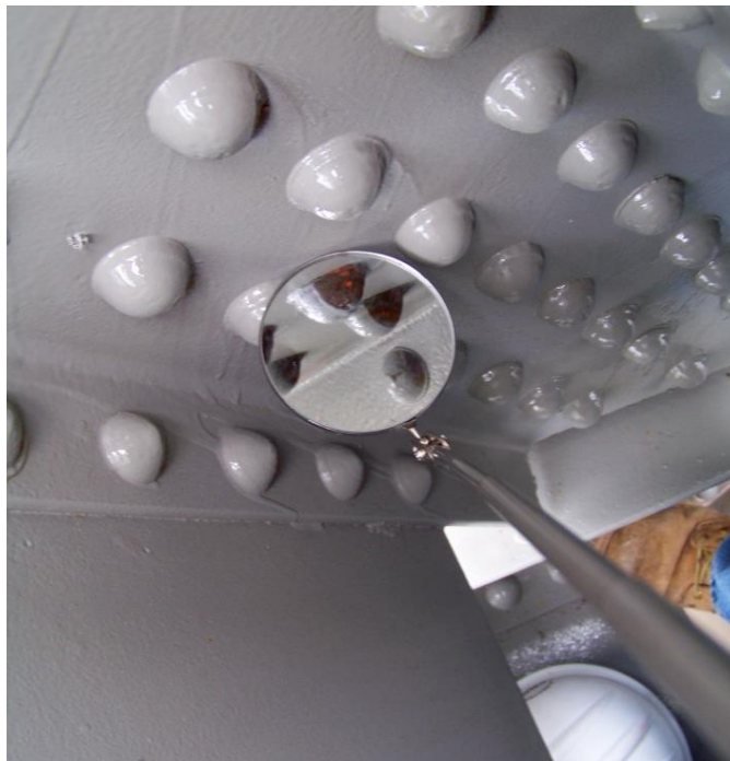
Figure 18.11 Obstructed Side of Rivet Pattern is Difficult to Paint
