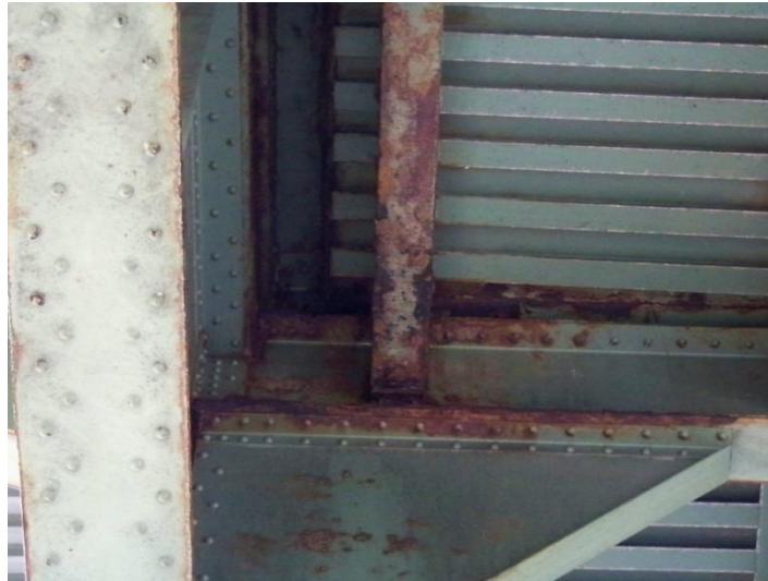
Figure 18.18 Corrosion Accelerated by Water Leaking at the Edges of a Roadway Deck
