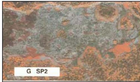
(a) Condition G cleaned using hand tools
