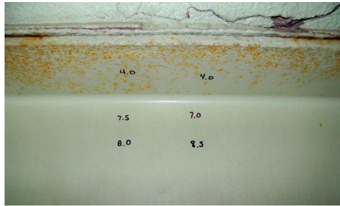
Figure 18.7 Corrosion Due to Low Dry Film Thickness (DFT)
