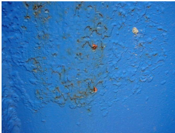
Figure 18.43 Close-Up Area on Bridge Showing Degradation from Poor Painting Practice
