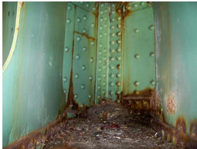
Figure 18.2 Inside Truss Bracing - Debris Collection and Accelerated Areas of Corrosion
