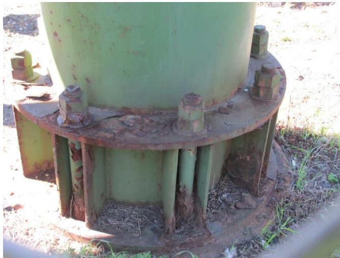
Figure 18.3 Corrosion on Irregular Surfaces of a Steel Pier Column Base
