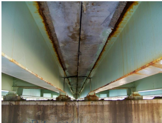
Figure 18.4 Corrosion on Beam Edges
