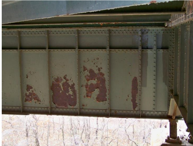
Figure 18.5 Aged Coating Exhibiting Peeling
