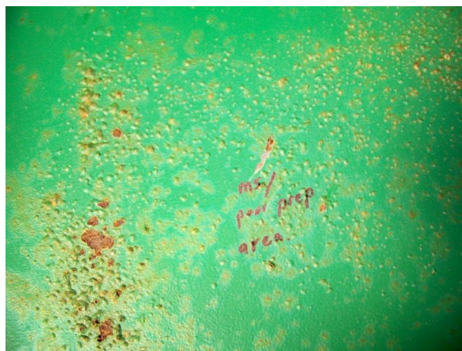
Figure 18.9 Coating Undercutting and Peeling
