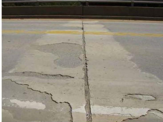
Photo-1 Shows delamination of the epoxy overlay/repair typical at Pier-3 and 4.
