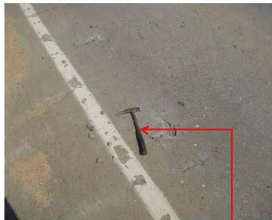
Photo-2 Shows delamination and shallow spalling to the deck in Span-2.
