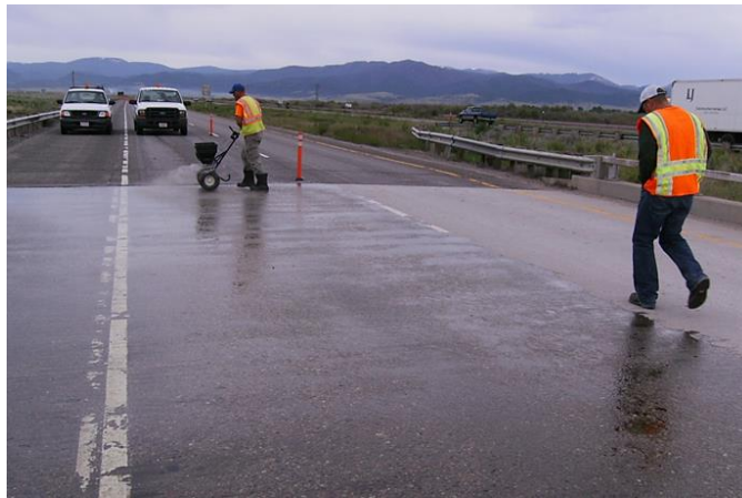
Figure A.31 Broadcasting Aggregate with Hand Operated Spreader (Courtesy of Kwikbond Polymers)
