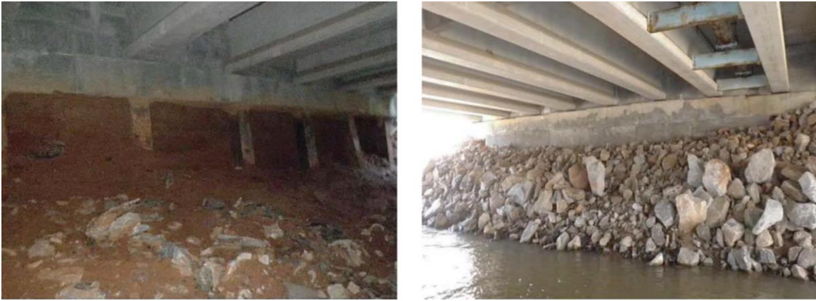
Figure A.39 Stone Abutment Slope Repair. Before Repair (left) and After (right). (Courtesy of Georgia DOT)
