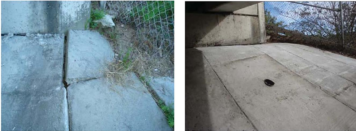
Figure A.38 Paved Abutment Slope Repair. Before repair (left) and After (right). (Courtesy of Georgia DOT)
