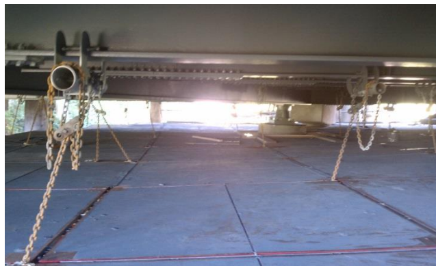
Figure A.10 Interior of the Dust Containment System
