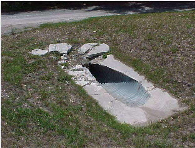
Side drainpipe with damaged concrete.
