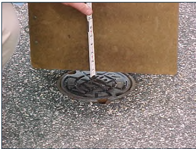
Depression at a water valve in pavement.
