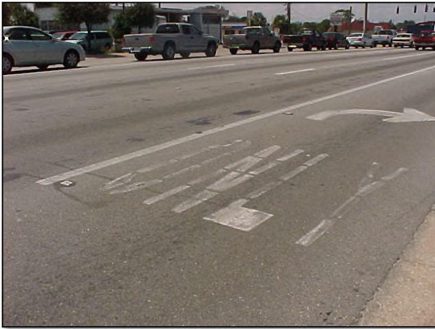
Worn and faded pavement symbol may not meet MRP standards.
