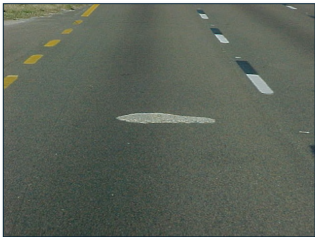
Concrete spill, rate as a bump.
