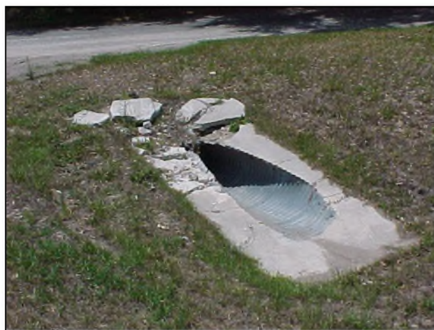
Side/cross drainpipe with damaged concrete. This does not meet MRP standards.
