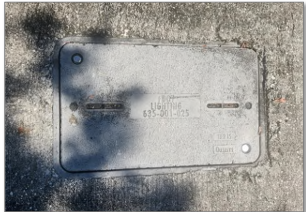
Pull box is properly secured. This meets conditions.
