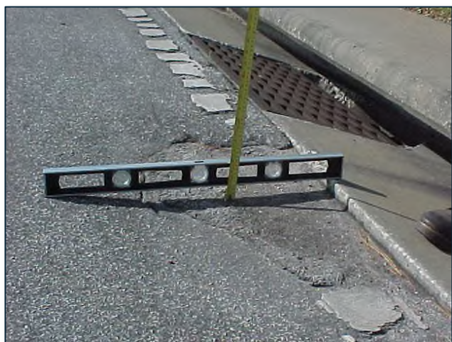
Depression next to a curb inlet.
