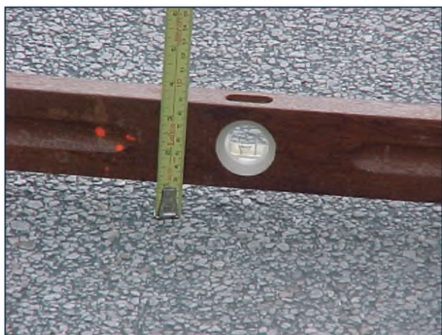
Measuring the depth of a depression.
