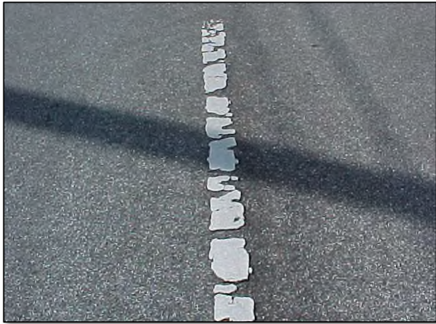
Edge line does not meet MRP standards.
