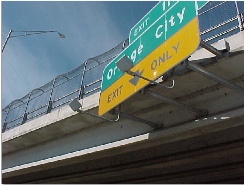
Overhead sign lighting.
