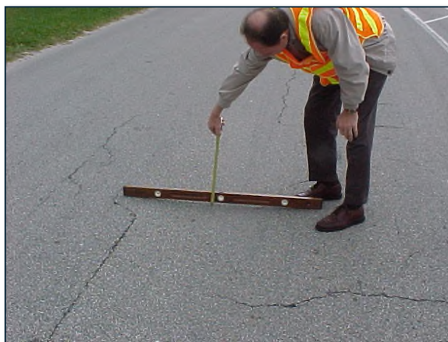
Measuring the depth of a depression.
