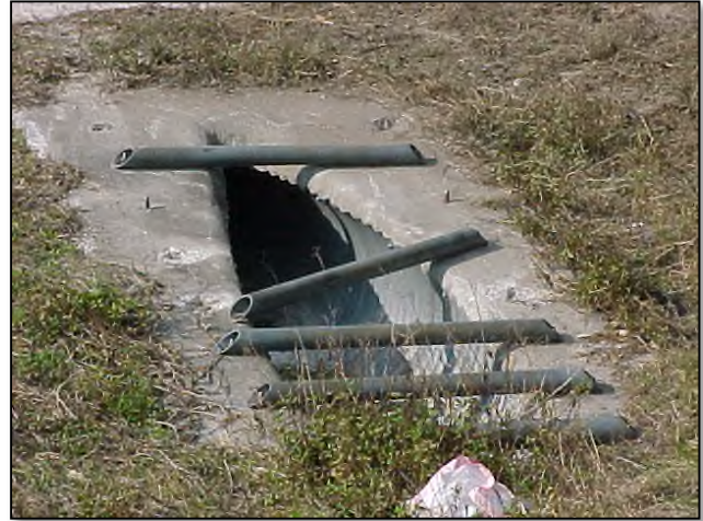
This is a side drainpipe with missing and damaged grates. This does not meet MRP standards.
