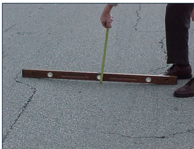
Measuring the depth of a depression.
