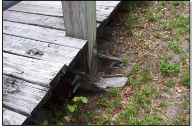
Deterioration of supports.
