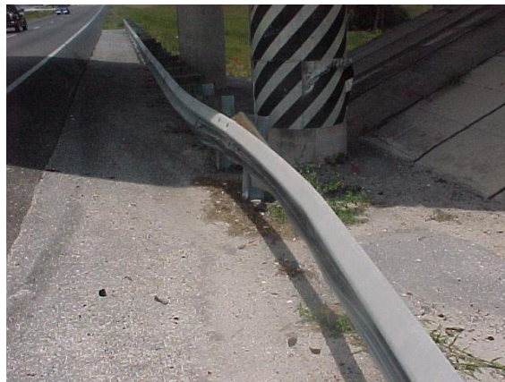
This guardrail has been hit and several posts are missing. This guardrail does not meet MRP standards.
