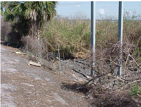
This fence has been damaged and is not the correct height. This does not meet MRP standards.
