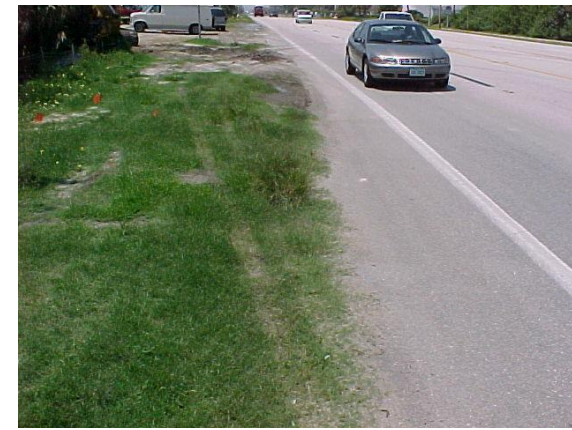
Build-up of sand, soil, and vegetation of unpaved shoulder onto outside paved shoulder.
