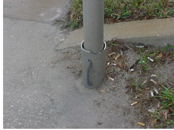
This sign foundation is non-standard and, therefore, does not meet MRP standards.
