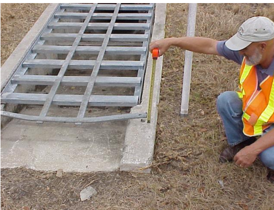
Broken bolt, grate bent. Does not meet conditions.
