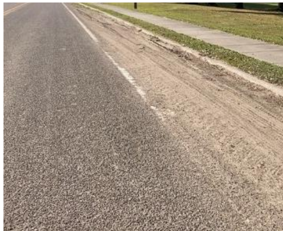
Edge line obscured by soil or other debris does not meet MRP standards
