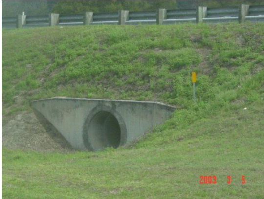
This object marker was installed but is not needed because the headwall is behind guardrail. Since the object marker is installed, it will be rated. The object marker is installed 2 feet 6 inches from the ground to the bottom of the marker. It should be installed no less than 4 feet plus or minus 1 foot from the ground to the bottom of the marker. This marker does not meet MRP standards.
