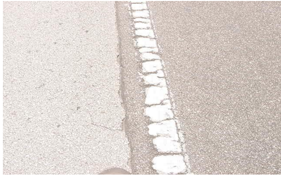
Worn out edge line does not meet MRP standards
