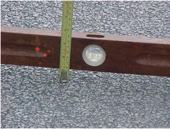
Measuring the depth of a depression.
