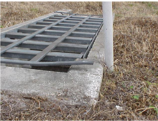
Broken/missing bolts, grate bent. Does not meet conditions.
