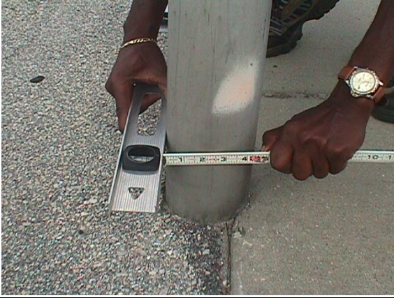
Measuring a sign post. This post is 4 inches and should be installed with a concrete foundation and breakaway assembly. This sign installation does not meet MRP standards.
