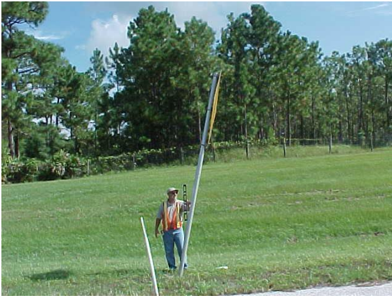
This sign is leaning more than 1 inch per foot and does not meet MRP standards.
