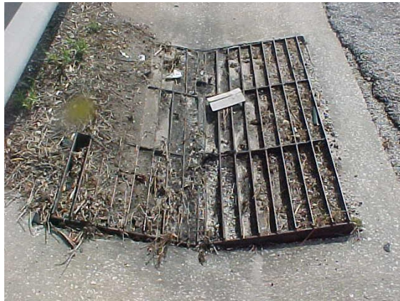
Blocked inlet grate. Does not meet MRP standards.
