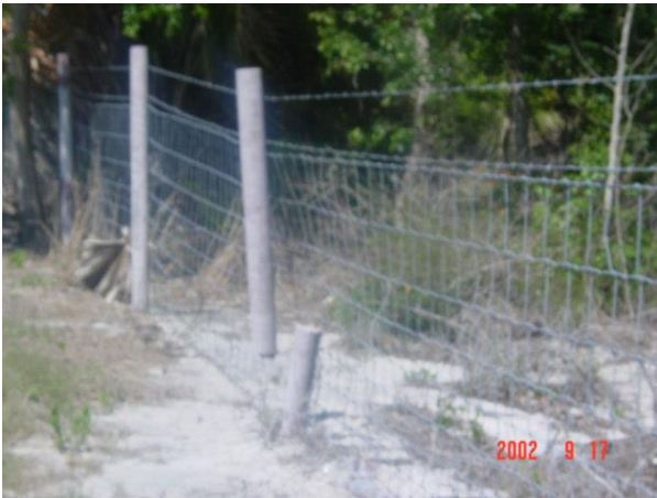
If two consecutive fence posts are missing or broken this would not meet MRP standards
