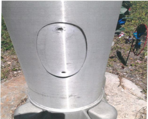
Inspection cover missing screws this would not meet conditions as properly secured.
