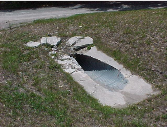
Side drain pipe with damaged concrete.
