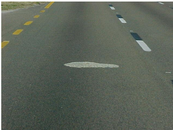
Concrete spill, rate as a bump.
