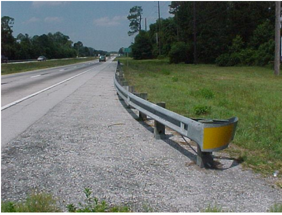
This end section has been hit and does not meet MRP standards.
