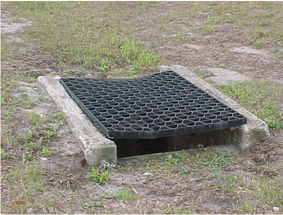
This inlet grate is not seated correctly in the design cradle. This does not meet MRP.
