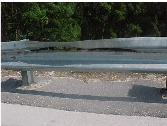
This guardrail section has been penetrated due to a crash. This does not meet MRP standards.
