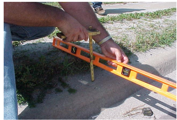
This is a soil buildup greater than 4 inches in the utility strip. It is built up more than 10 continuous feet and, therefore, does not meet MRP standards.
