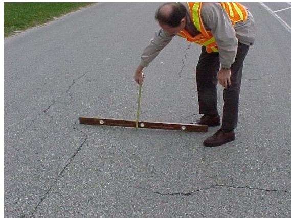
Measuring the depth of a depression.
