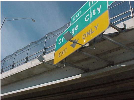
Overhead sign lighting
