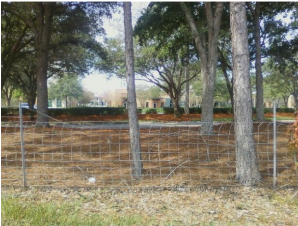
Both strands of barb wire are missing along top of fence, this would not meet desired maintenance conditions.
