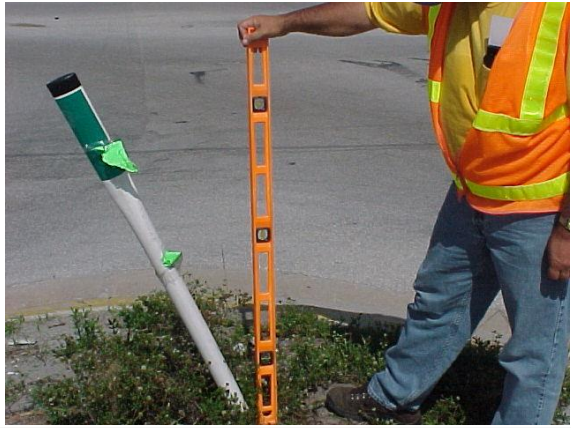
This post mounted delineator is leaning more than 1 inch per foot and does not meet MRP standards.
