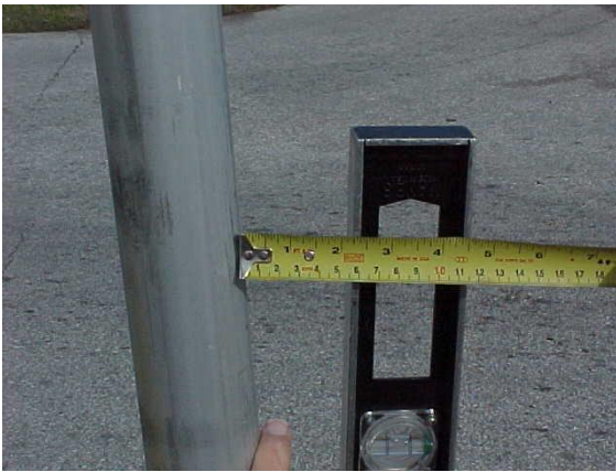
Measuring a sign that is leaning more than 1 inch per foot. Using a 2ft. level this sign does not meet desired maintenance conditions.
