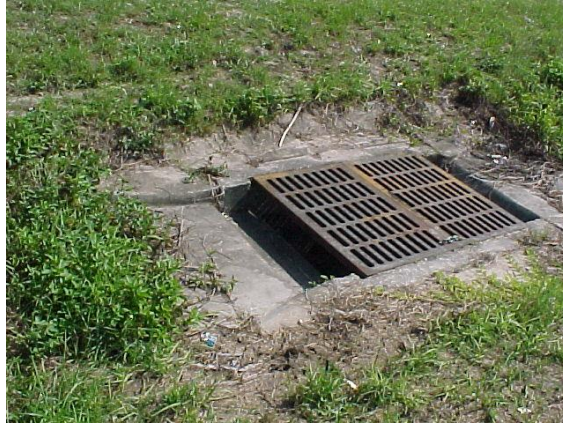
Ditch bottom inlet in good condition. This meets MRP standards.
