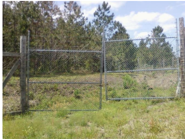
Misaligned gates, measure opening to ensure it is not greater than 6-inches.
