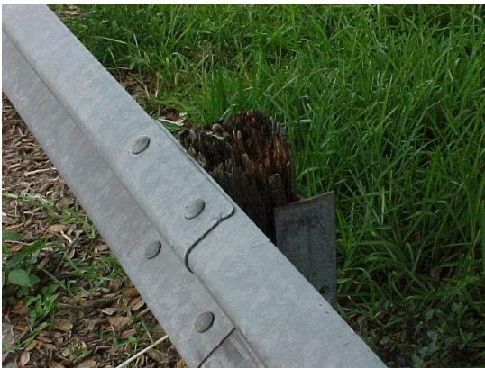
This guardrail section has several problems. The offset block is deteriorated and the rail is lapped incorrectly. This does not meet MRP standards.
