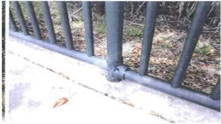
Cracked or broken hardware would not meet desired maintenance conditions.
