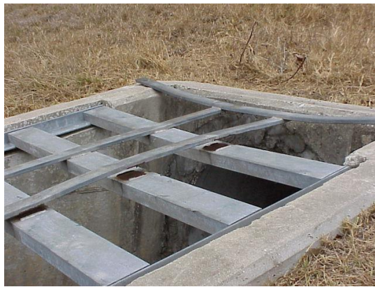
Broken welds on grate. Does not meet conditions.
