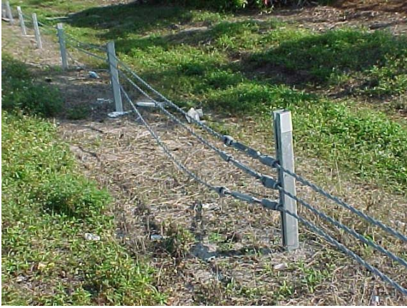
Loose cables on GIBRALTAR would not meet MRP standards.
