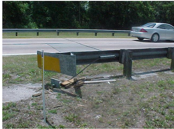
Damaged guardrail end section. This site does not meet MRP standards.
