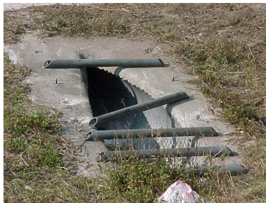
This is a side drain pipe with missing and damaged grates. This does not meet MRP standards.
