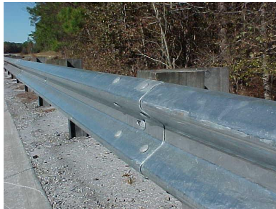
This guardrail section is lapped incorrectly. If hit by a vehicle, the rail would not function as designed. This does not meet MRP standards.
