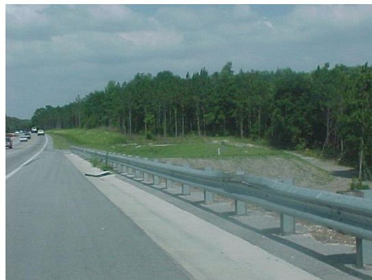
Penetrated guardrail does not meet MRP standards.
