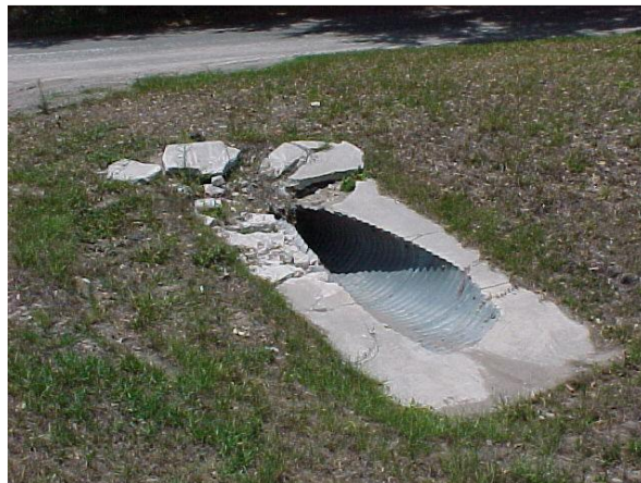
Side/cross drain pipe with damaged concrete. This does not meet MRP standards.
