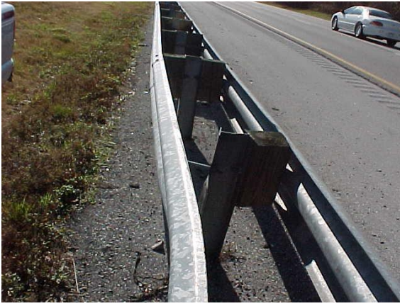
This guardrail has minor damage to the rail and a missing offset block. This would not meet MRP standards.
