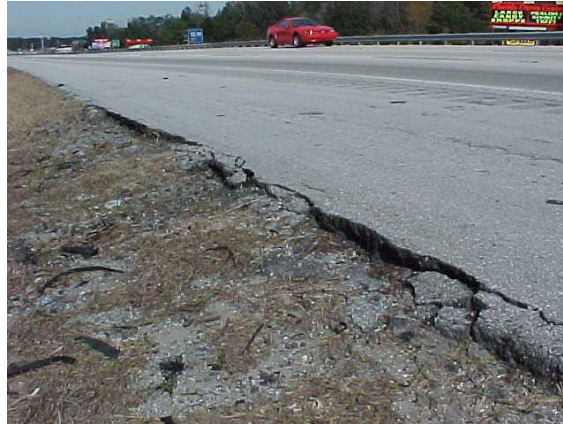
Edge raveling on paved shoulder. Measurements should be taken to determine if this meets MRP Standards.
