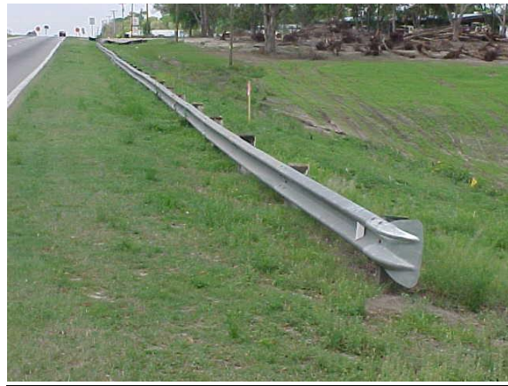
This guardrail section is low and should be measured to determine if it meets MRP standards.
