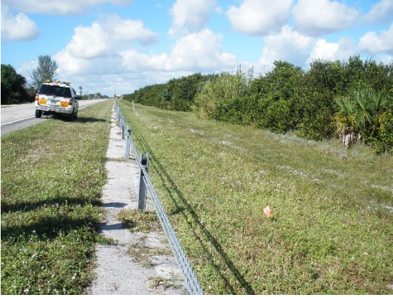
Misaligned cable would not meet desired maintenance conditions.
