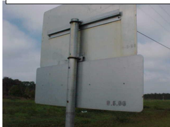
Incorrect bracket installation.
