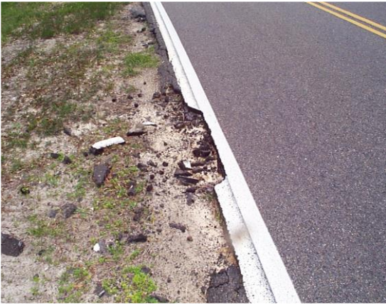
A roadway without paved shoulders would be rated for edge ravel.
