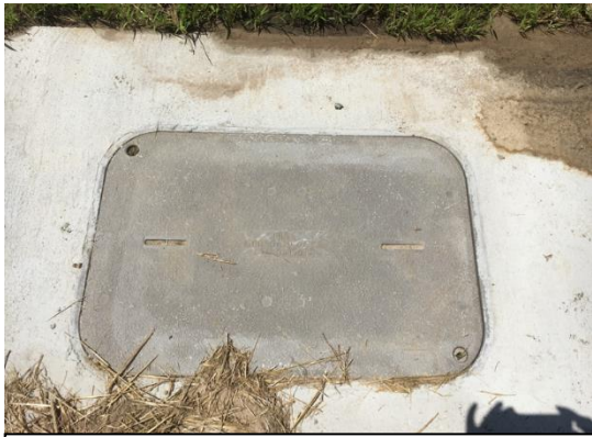
Pull box missing bolts. This would not meet conditions.
