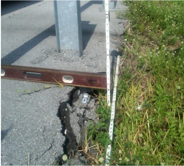
The asphalt is broken with a deviation greater than 5 inches and would not meet desired maintenance conditions for unpaved shoulder
