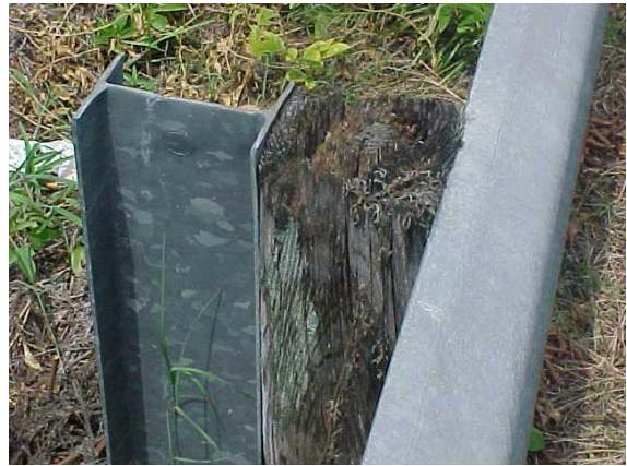
This is a rotten and deteriorated guardrail offset block. It does not meet MRP standards if more than 10% of the blocks are rotten and deteriorated.
