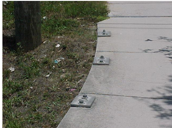
Missing handrail, this does not meet MRP standards.
