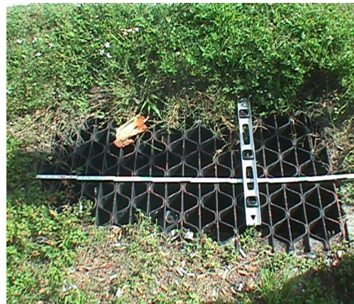
This is an obstructed inlet grate. If the opening is obstructed more than 85% , then it would not meet MRP standard for inlets.
