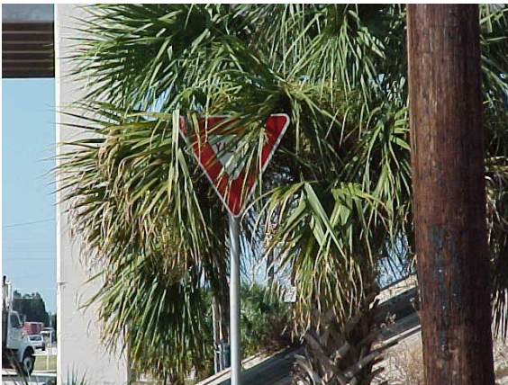
This sign is in good condition but cannot be seen because of a palm tree. The sign meets MRP standards, however tree trimming would not meet MRP standards.
