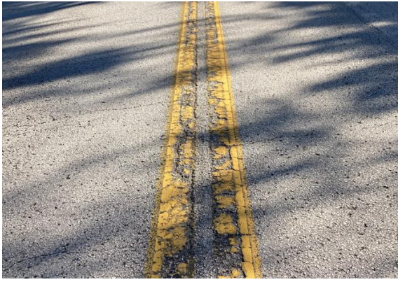
Worn out striping does not meet MRP standards.
