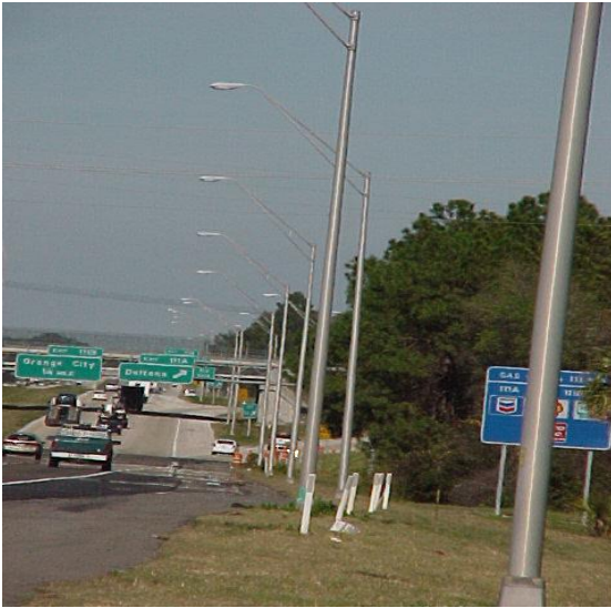
Standard roadway lighting. Count the number of luminaries within the sample.
