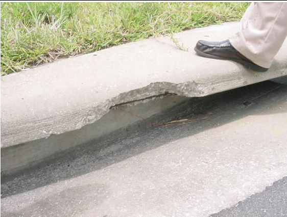
Exposed steel with spalling in this curb inlet. This does not meet MRP standards for inlets.
