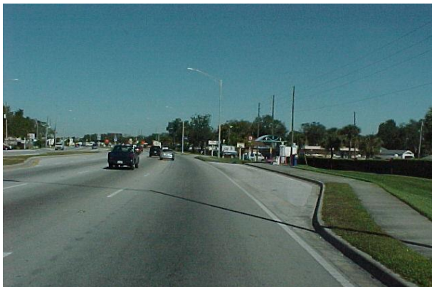
The paved area to the right in this photo is a bus turnout. The pavement in a bus turnout should be evaluated as roadway pavement.
