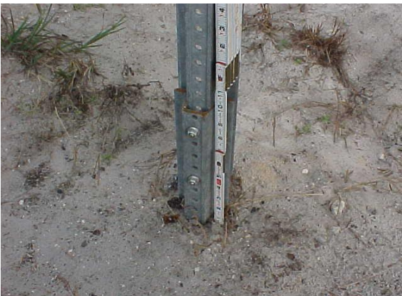
This steel flanged channel post is installed greater than 4 inches above the ground and is a non-standard installation does not meet MRP standards.
