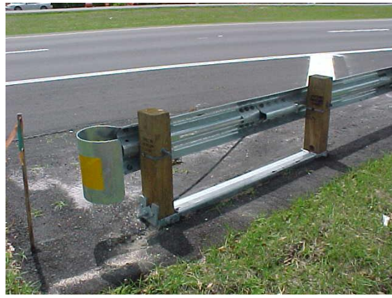
This is an approach end guardrail end section. Check to make sure all connecting hardware is in place.
