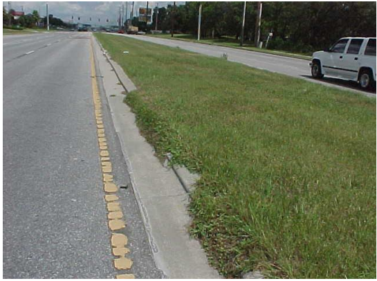
This vegetation is encroaching the curb more than 6 inches for more than 10 feet. This does not meet MRP standards for curb/sidewalk edging.
