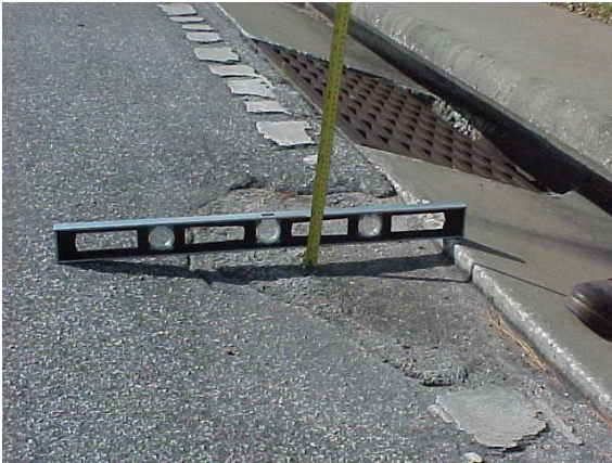
Depression next to a curb inlet.
