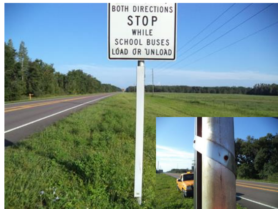
This Retroreflective panel is the correct color but has been riveted into the post. This would not meet maintenance conditions.
