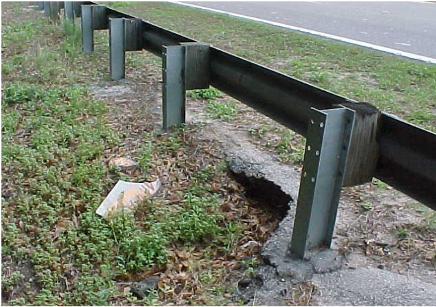
The asphalt under the guardrail has washed out. The guardrail meets desired maintenance conditions; however, unpaved shoulder or front slope would not meet MRP standards.
