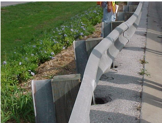
This guardrail has been hit by a vehicle. The posts have been knocked out of alignment and may not function as designed. This guardrail does not meet MRP standards.
