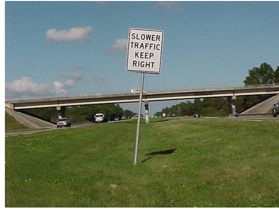
Signs should not lean more than 1 inch per foot.
