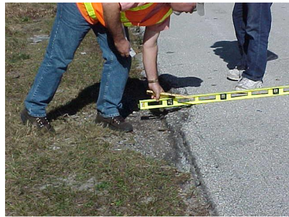
Shoulder drop off greater than 5 inches does not meet MRP Standards.
