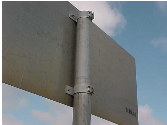
This sign was installed using "C clamps and does not meet MRP standards.
