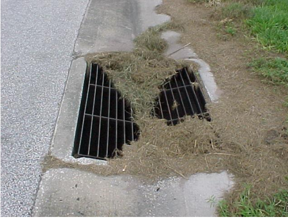
Grass covering inlet grate. Determine the percentage of opening area obstructed. If more than the standard, it would not meet MRP standards.
