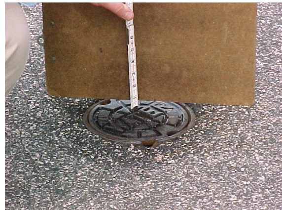
Depression at a water valve in pavement.
