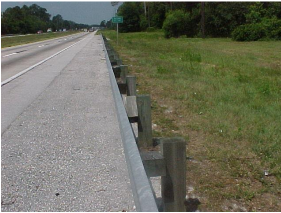
Guardrail offset blocks are not aligned properly. This condition does not meet MRP standards if more than 10% are twisted.
