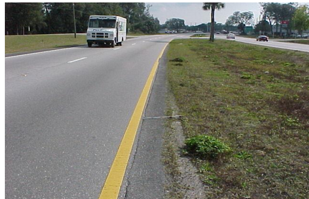
This edge widening is less than 2 feet wide therefore, does not meet MRP standards for paved shoulders (unless specified in the Straight-line Diagrams).
