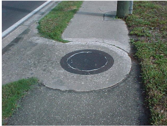
This manhole cover is seated correctly in the design cradle. This meets MRP standards.
