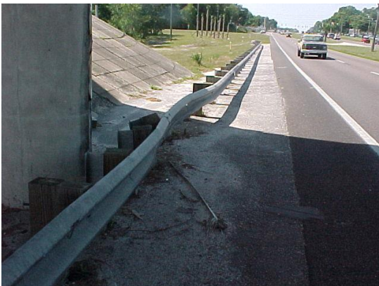
This guardrail has been damaged by a crash. Several posts are damaged. This does not meet MRP standards.
