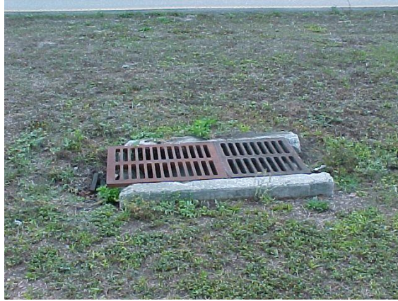
The inlet grate on the left is the wrong size. This would not meet MRP standards.
