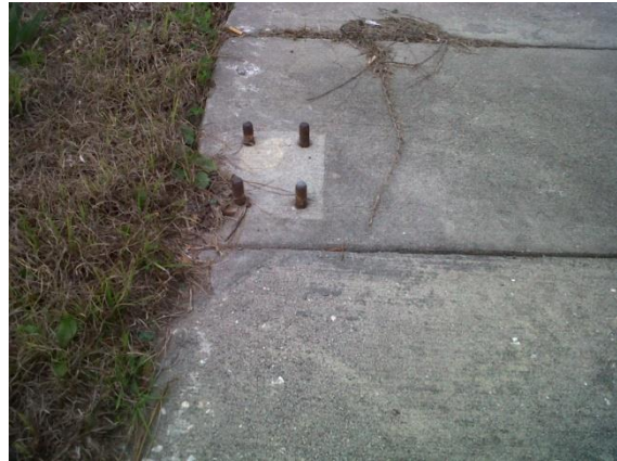
Rigid objects protruding from concrete greater than 1/4 inch in height.
