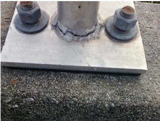
Broken welds will not meet desired maintenance conditions.
