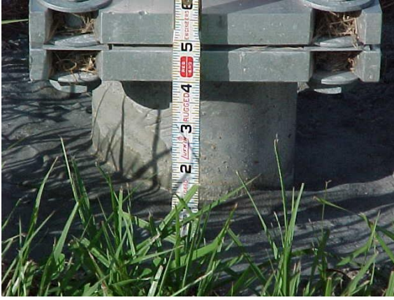
Slip base more than 4 inches above the ground. This does not meet MRP standards.
