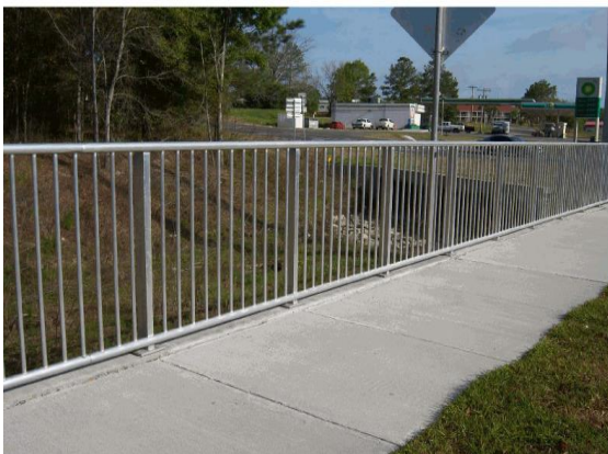
Picket railing protecting drop-off next to sidewalk.
