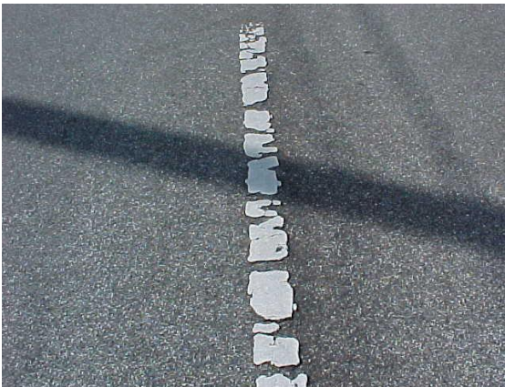
Edge line does not meet MRP standards
