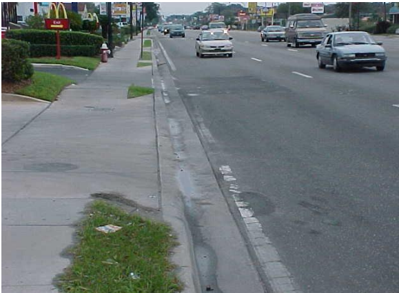
Worn out striping in an urban area does not meet MRP standards.
