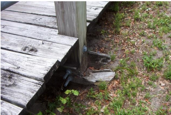
Deterioration of supports.
