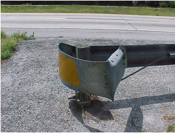
This damaged end section does not meet MRP standards.
