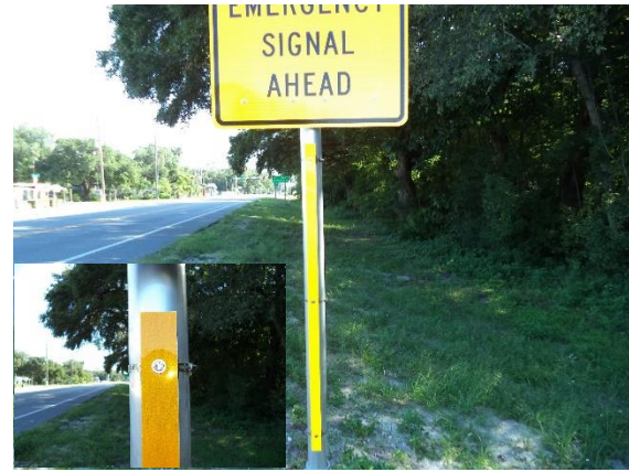
This Retroreflective panel is the correct color and has been mounted to the post correctly. This would meet maintenance conditions.
