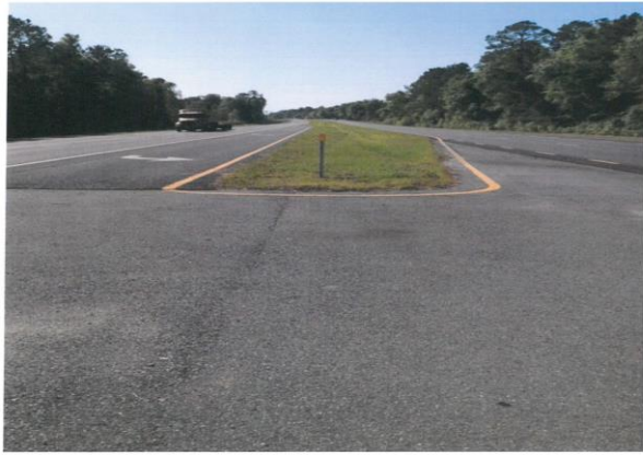
Rate edge raveling at crossovers where pavement without paved shoulders ties into paved shoulders.
