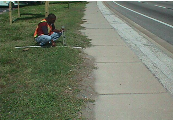
This vegetation encroachment on the sidewalk does not meet MRP standards for curb/sidewalk edging.
