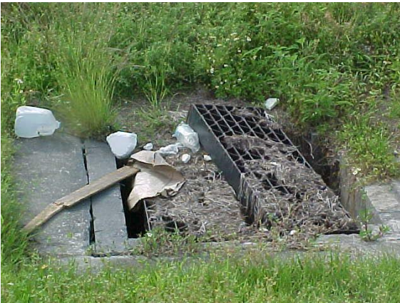
Inlet grate out of cradle. Does not meet MRP standards.
