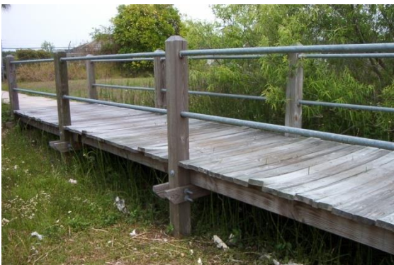
Surface deck boards with misalignments.
