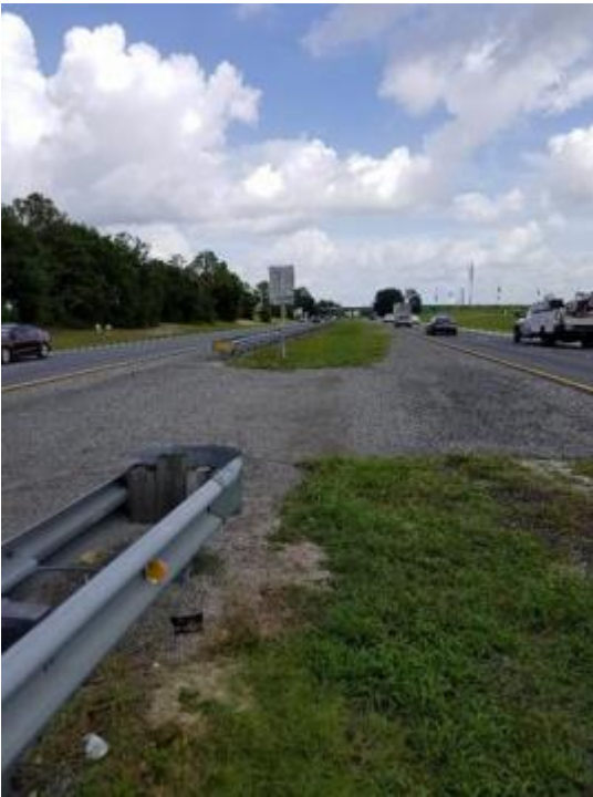
Do not rate edge raveling at crossovers where pavement with paved shoulders are present.
