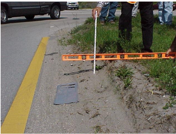
High shoulder 2 inches or more for 25 continuous feet does not meet MRP Standards.
