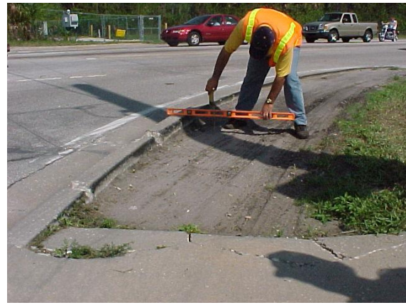
Drop-off behind curb. Since this road has curb & gutter this would be evaluated under curb & sidewalk edging.
