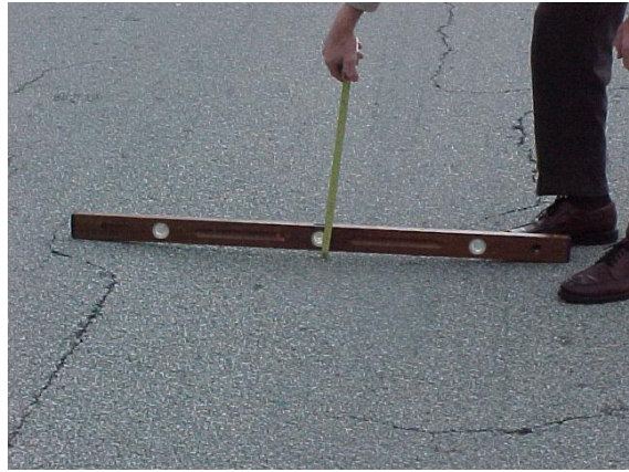
Measuring the depth of a depression.
