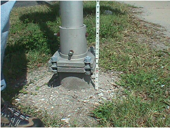
Slip base more than 4 inches above the ground. This does not meet MRP standards.
