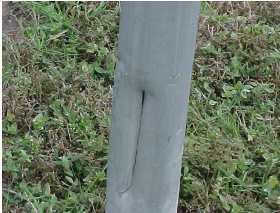
This sign column has been damaged and does not meet desired maintenance conditions.
