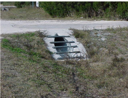
This is a side drain pipe with grates. This meets MRP standards.
