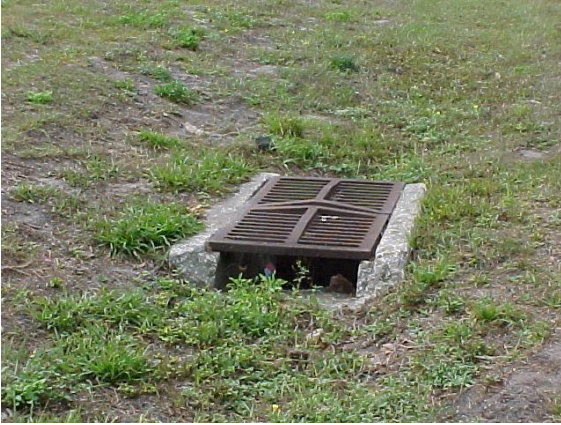
These inlet grates are installed upside-down. This would not meet MRP standards.
