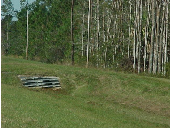
Side drain pipe with grates.
