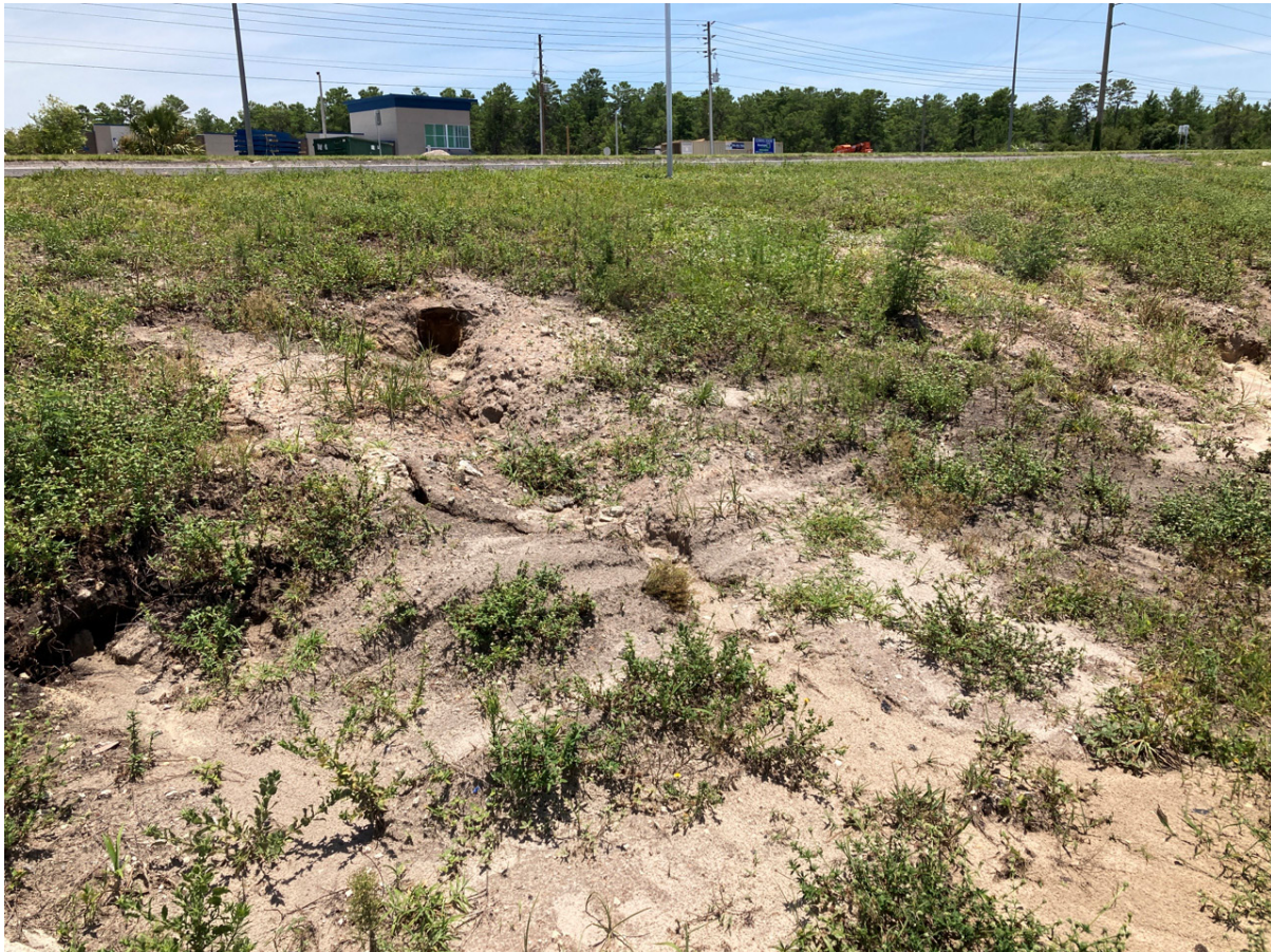
PHOTO 4 LOOKING AT EROSIONAL AREAS EAST OF SKIMMER AT STA 463+10 LT.JPG
