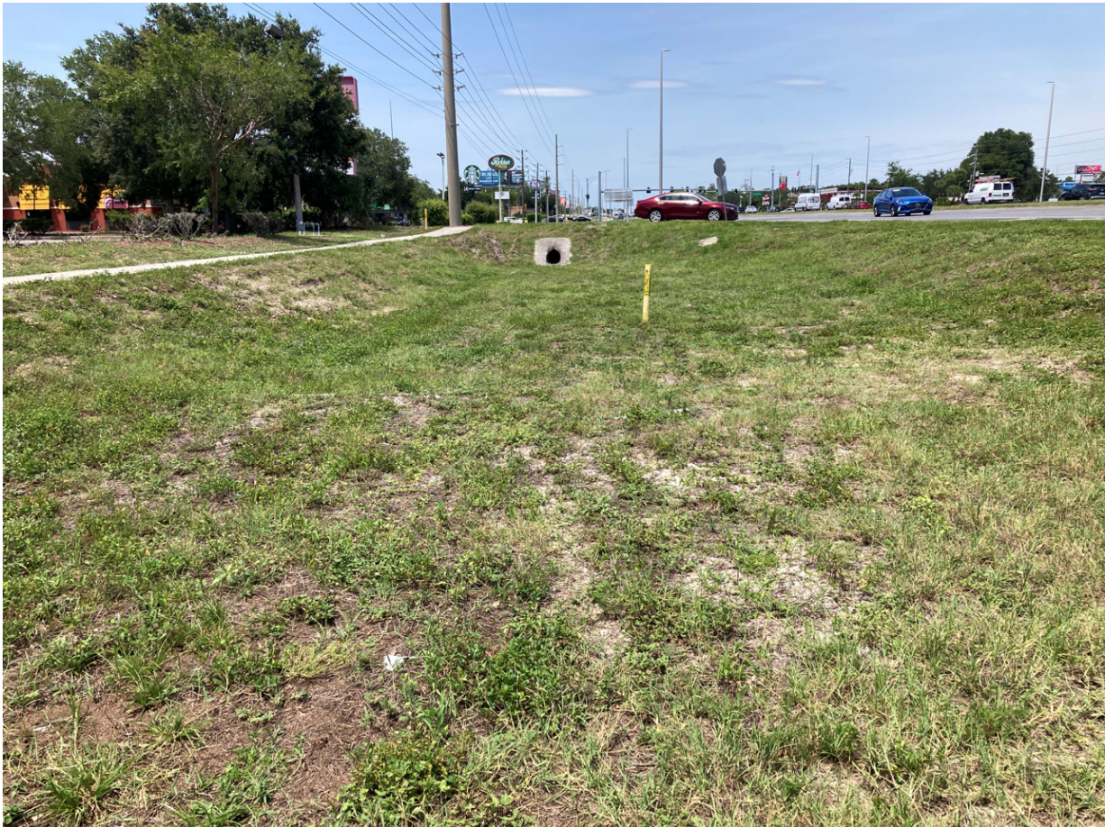
PHOTO 28 LOOKING NORTH AT DB-7 STA 431+80 LT (LOSS OF TREATMENT VOLUME).JPG
