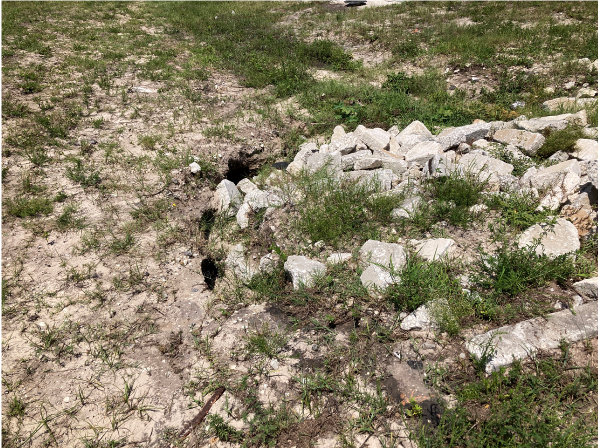
PHOTO 22 LOOKING AT EROSIONAL AREA WHERE WATER IS BYPASSING DB-13 ON WEST ED.JPG
