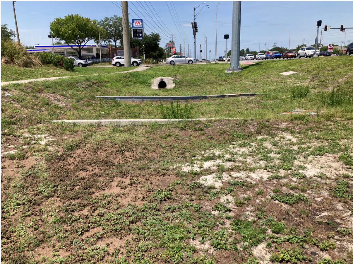
PHOTO 26 LOOKING NORTH AT DB-9 STA 432+80 LT (SEDIMENT ACCUMULATION).JPG
