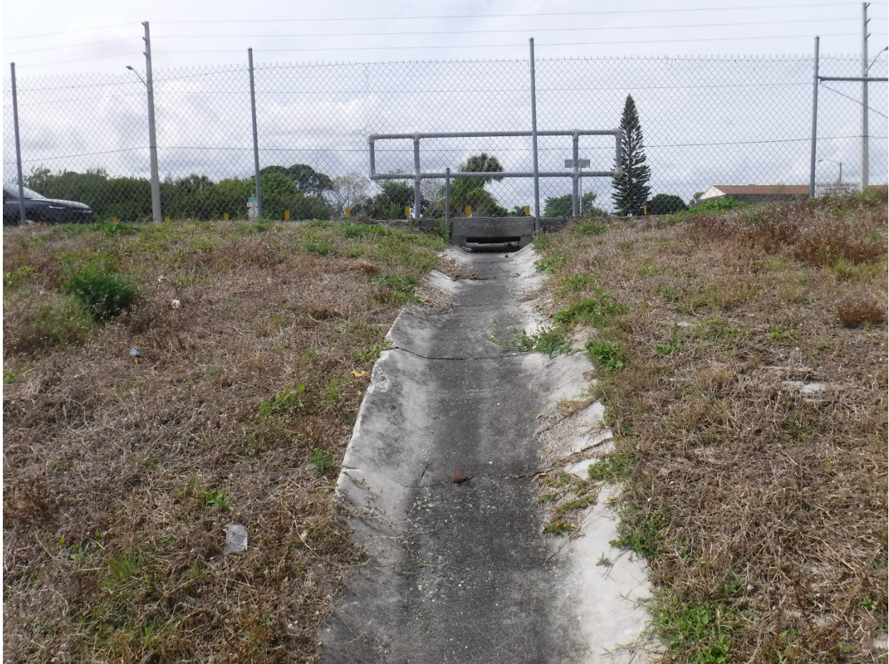
Figure 4-41. Typical Open Conveyance Outfall in Good Condition Return to List of Figures
