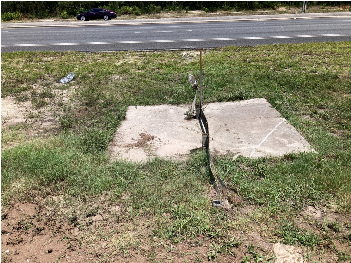
PHOTO 21 LOOKING EAST AT DB-13 SKIMMER (DAMAGED).JPG
