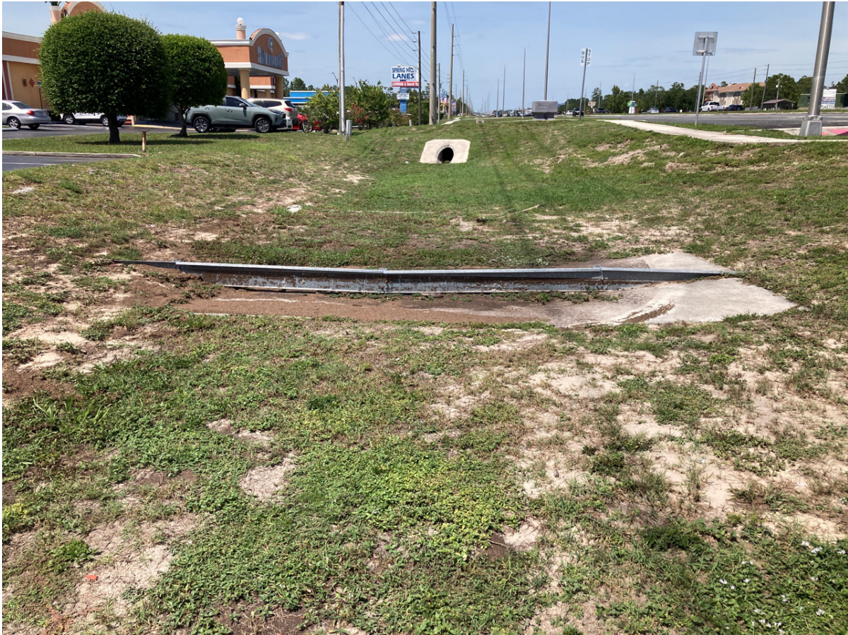
PHOTO 34 LOOKING NORTH AT DB-1 STA 411+80 LT (SEDIMENT ACCUMULATION).JPG
