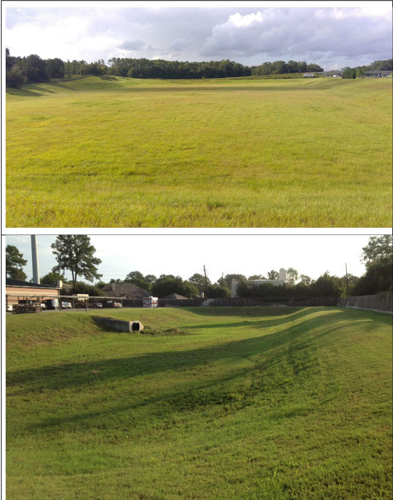
Figure 4-23. Typical Dry Retention Ponds in Good Condition Return to List of Figures
