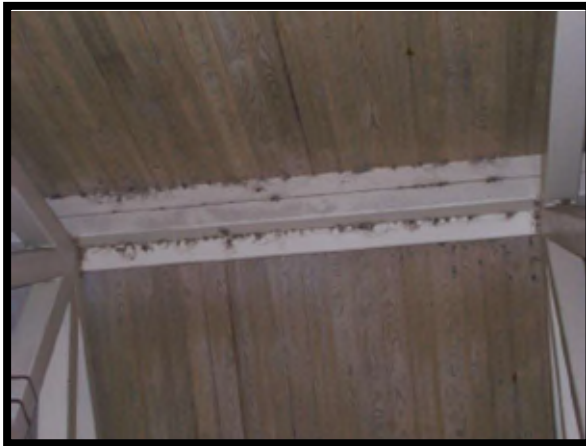
A ceiling with cobwebs would not meet desired maintenance conditions.
