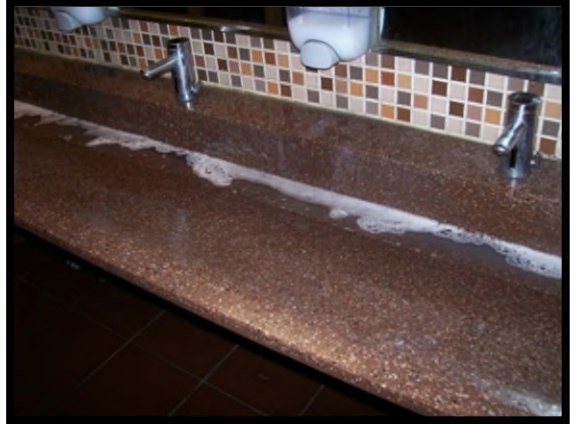
The water is not draining properly and would not meet desired maintenance conditions.
