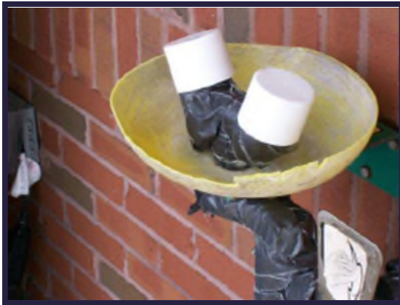
Broken or deteriorating plastic on eyewash station would not meet the desired maintenance conditions.
