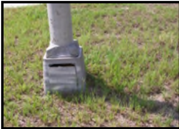
An unsecured access panel would not meet the desired maintenance conditions.
