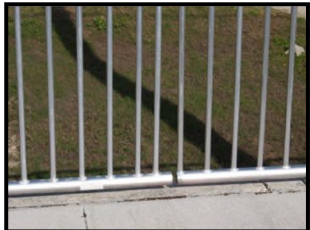
The picket railing is missing a steel sleeve at the expansion joint. This would not meet desired maintenance conditions.
