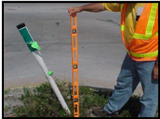
This delineator is leaning more than 1 inch per foot and would not meet desired maintenance conditions.
