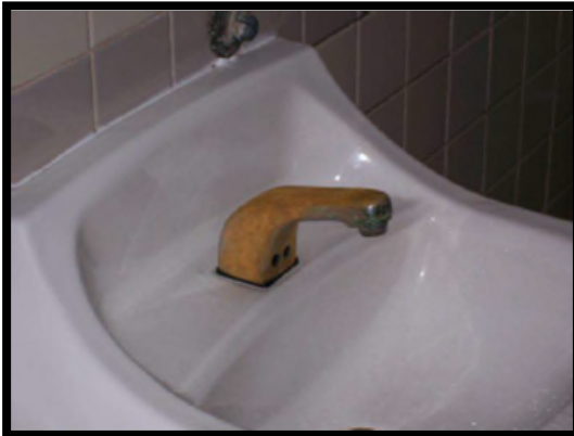
sinks that did not meet criteria. Faucet is corroded and would not meet desired maintenance conditions.
