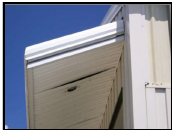
Soffit needs to be repaired and cleaned. This does not meet desired maintenance conditions.
