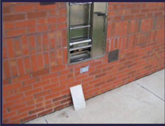
Missing door/covers would not meet the desired maintenance conditions.
