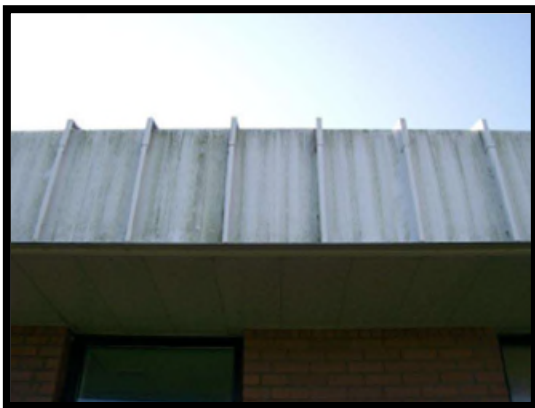
Roof/Fascia has dirt and mildew build-up. This does not meet desired maintenance conditions.
