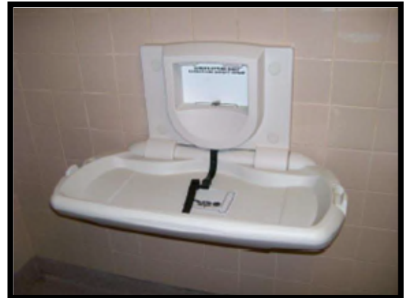
Changing table with straps meets desired maintenance conditions.
