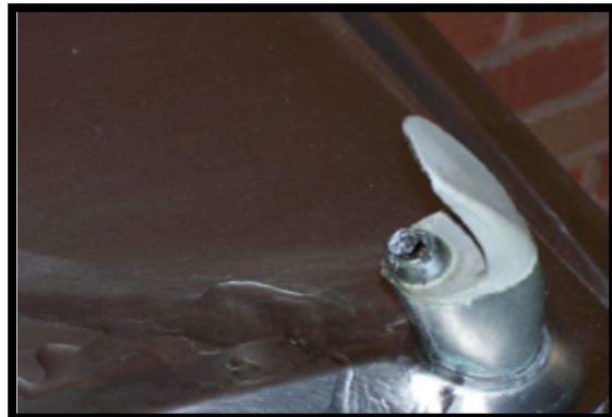
This water fountain will not shut off and would not meet desired maintenance conditions.
