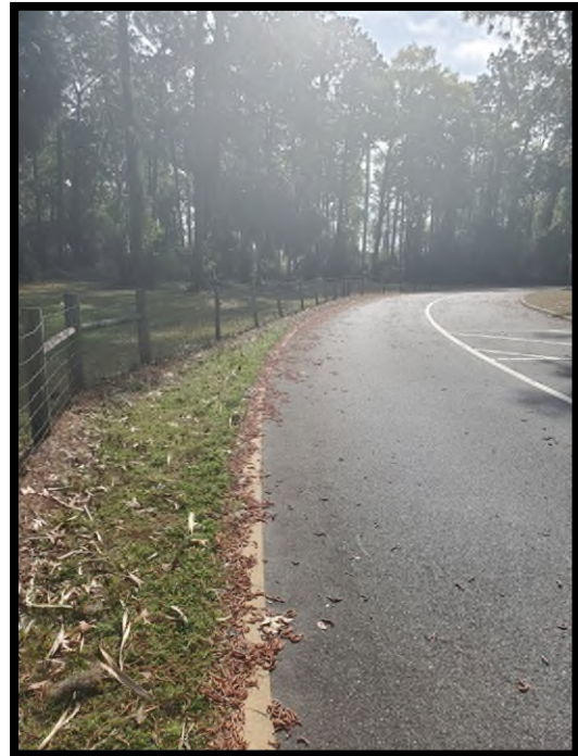
Example of edge line covered with grass, if the striping covered in grass is more than 52 continuous feet in length; this would not meet the desired maintenance conditions.
