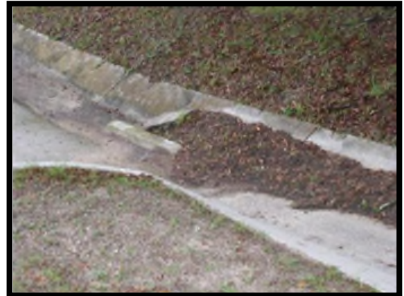
If the buildup in this ditch obstructs the flow of water, it would not meet desired maintenance conditions.
