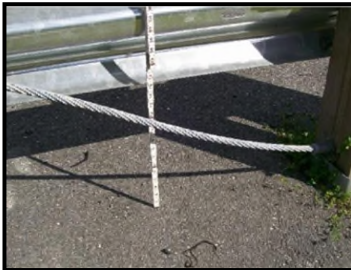
The cable is not taut and may deviate more than 1 inch, this may not meet desired maintenance conditions.
