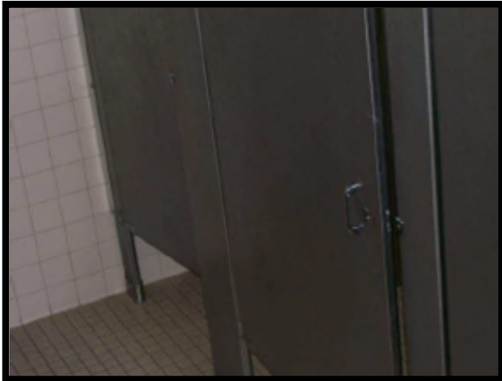
This door has a broken latch and would not meet desired maintenance conditions.
