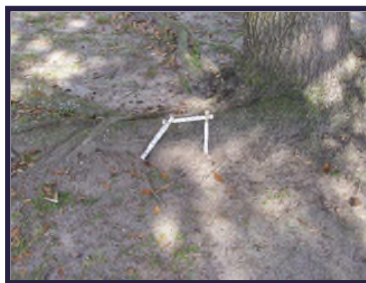
Tree root is greater than 3 inches above natural ground this would not meet the desired maintenance conditions if within the walking area.
