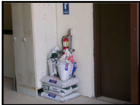
Extinguisher is obstructed and would not meet desired maintenance conditions.
