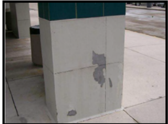
Example of a wall with peeling paint. Depending on the percentage of the walls in this condition, there is a possibility this facility would not meet desired maintenance conditions.
