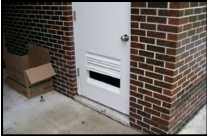
This door has a missing panel and would not meet desired maintenance conditions.
