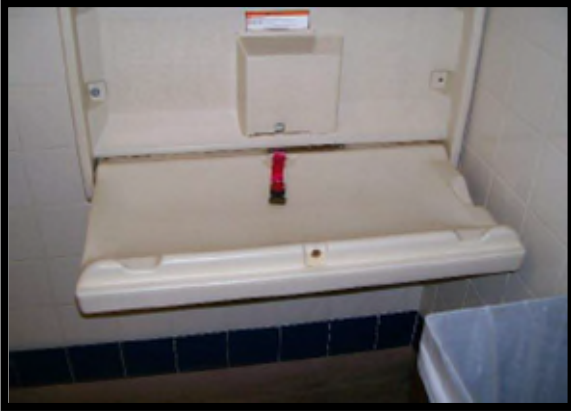
Changing table with missing or broken strap would not meet desired conditions.
