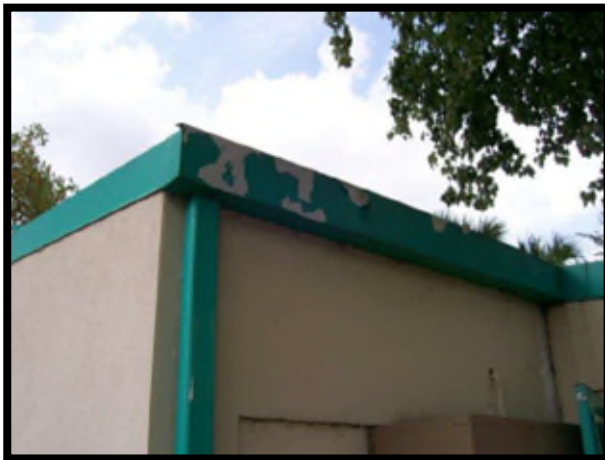
This gutter system should be painted to meet desired maintenance conditions.
