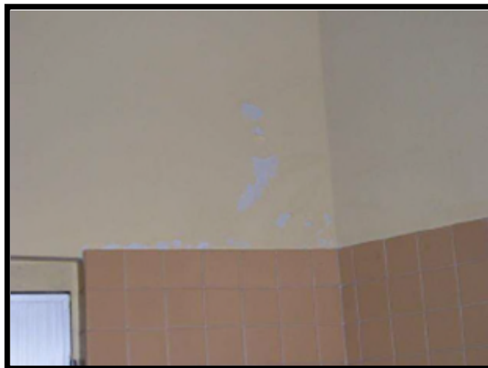
Example of peeling paint on a wall that would not meet desired maintenance conditions.
