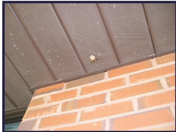
Example of wasp nest. If wasps are present this would be considered active and would not meet the desired maintenance conditions.
