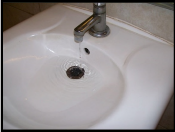
This faucet is leaking and draining slow. This would not meet desired maintenance conditions.
