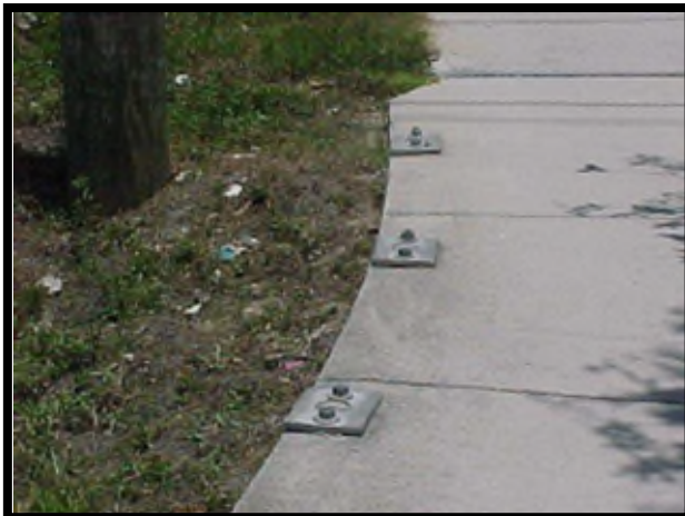
A missing handrail does not meet desired maintenance conditions.
