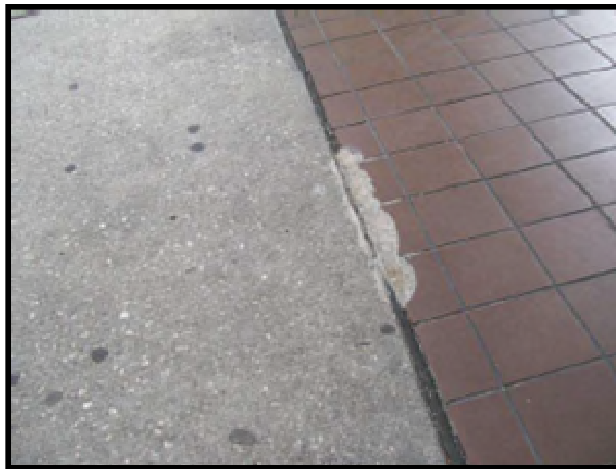
Misaligned/broken tiles could be a trip hazard and does not meet desired maintenance conditions.
