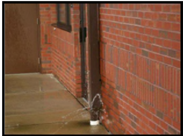
A gutter blocked and leaking does not meet desired maintenance conditions.
