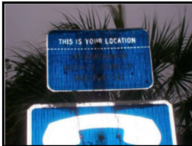
This sign is dirty would not meet the desired maintenance conditions.
