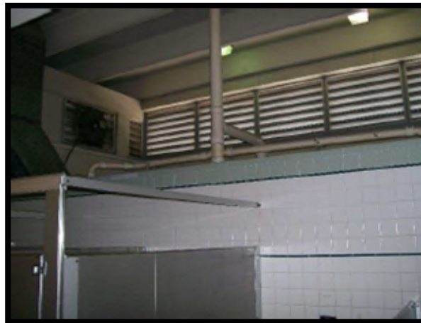
Buildup of dust on top of wall and pipe. This would not meet desired maintenance conditions.
