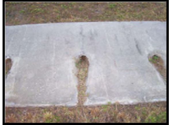
Measure the pipe opening to determine if 90% is unobstructed.
