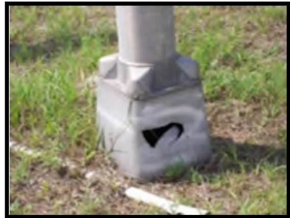
There is damage to the lighting base, and this would not meet desired maintenance conditions.
