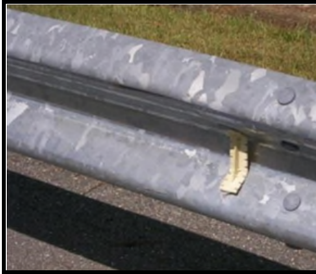
A missing hazard marker reflector may not meet desired maintenance conditions.
