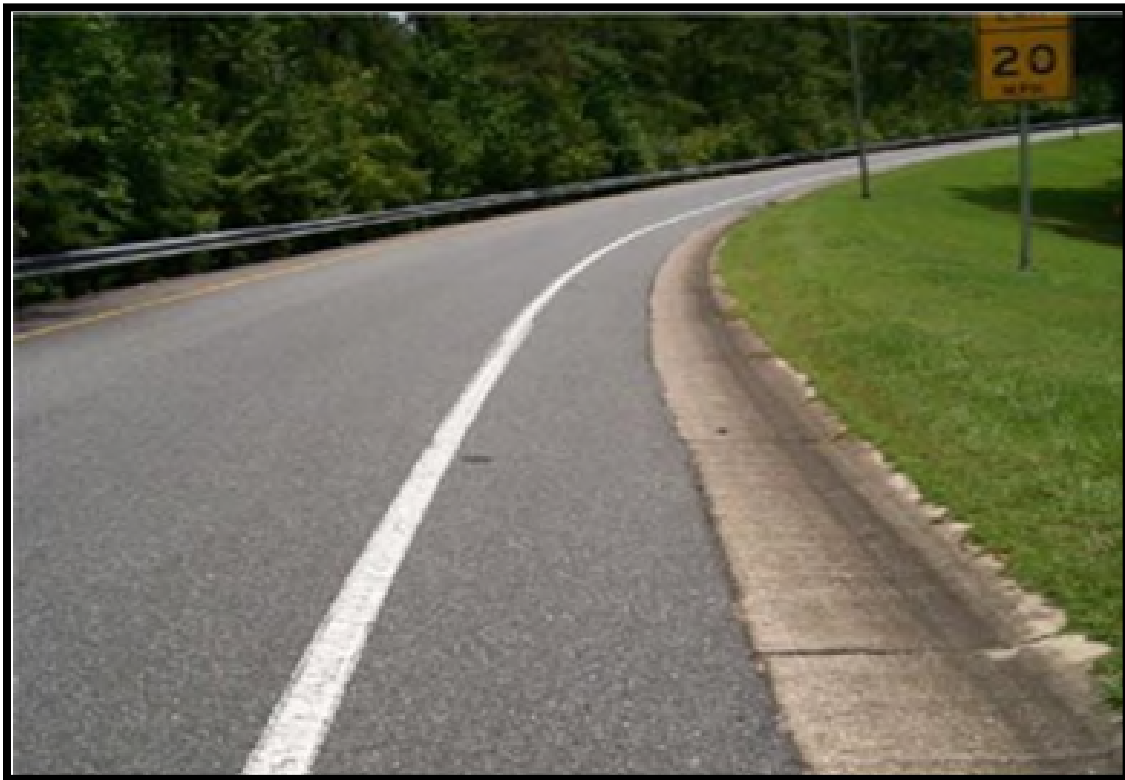
Example of missing RPMs on ramp edge line striping. This does not meet desired maintenance conditions.
