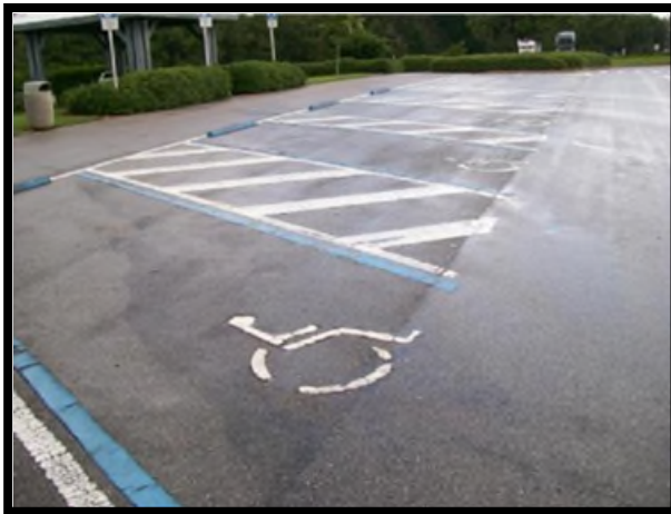
Example of symbols in a parking area that meets desired maintenance conditions.
