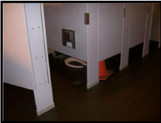
The toilet in this stall is missing and would not meet desired maintenance conditions.
