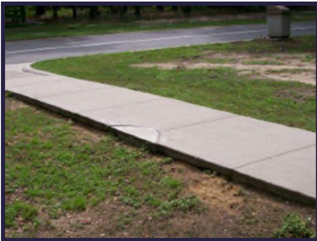
Deviation of soil for more than 2 inches this would not meet desired maintenance conditions.
