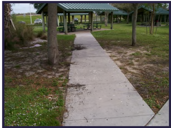
An example of a sidewalk that is not edged and swept. This does not meet desired maintenance conditions.
