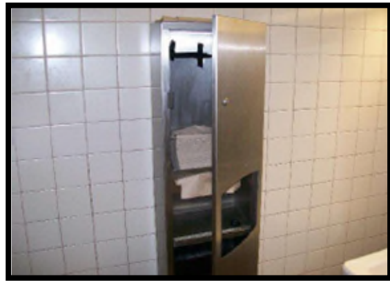
Cabinet door should be secured and function as intended. This would not meet desired maintenance conditions.
