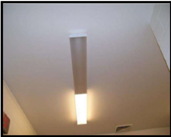
This light is not working and would not meet desired maintenance conditions.
