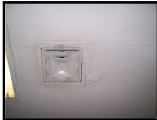
Ceiling with a dirty stained vent with cracked and peeling paint would not meet desired maintenance conditions.
