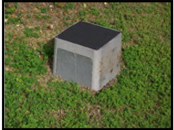
Missing light pole would not meet the desired maintenance conditions.
