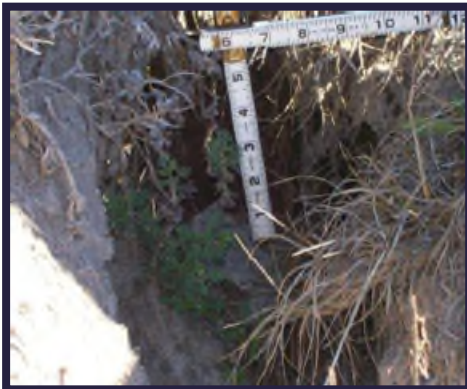
Large hole six (6) inches deep in the common and picnic area grounds this would not meet the desired maintenance conditions.
