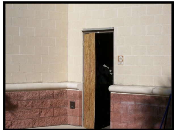
This door is missing the lock, enclosed with cardboard and duct tape. This would not meet desired maintenance conditions.
