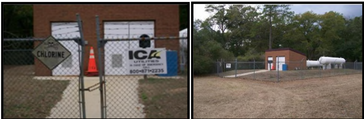
Examples of water treatment facilities with signs in place and secured, meeting the desired maintenance conditions.
