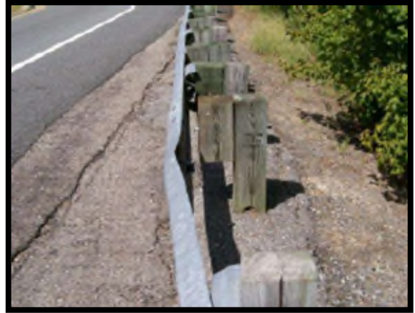
A damaged guardrail that is pulled away from the block, would not meet desired maintenance conditions.
