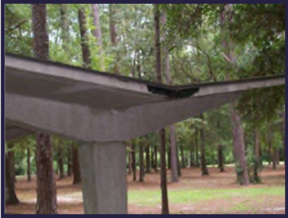
Mildew and peeling paint on this shelter would not meet desired maintenance
