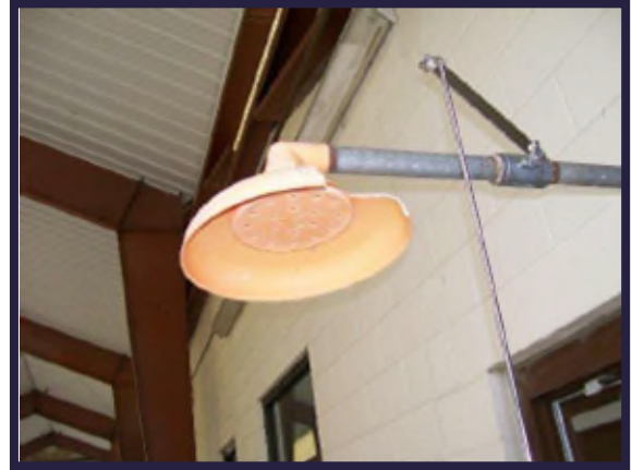
Broken shower head would not meet the desired maintenance conditions.
