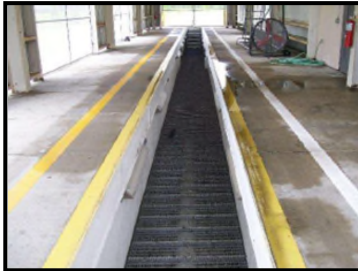
Inspection pit and ventilation system.
