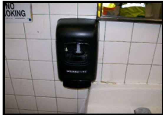
Soap dispenser is missing front cover, soap packet, and would not meet desired maintenance conditions.
