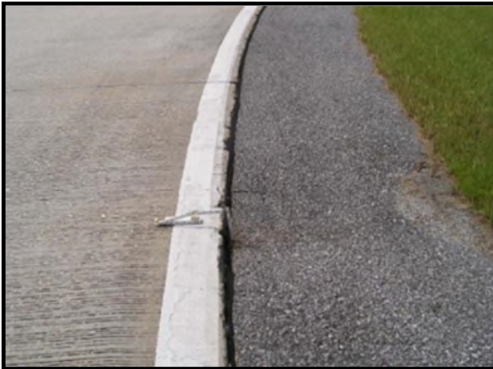
Example of a drop off on the paved shoulder that is greater than 3 inches in depth. If this is continuous for more than 20 feet, it would not meet the desired maintenance conditions.
