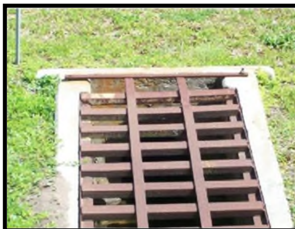
Grate missing hardware, an anchor bolt in the corner, this would not meet desired maintenance conditions.
