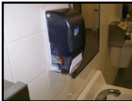
Broken or missing soap dispensers would not meet desired maintenance conditions.
