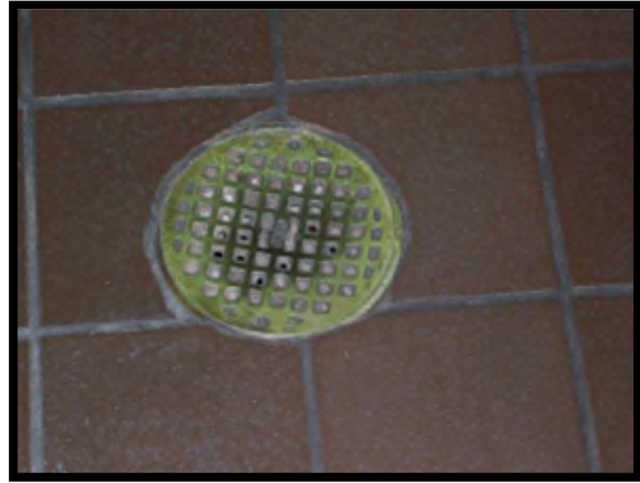
A blocked floor drain would not meet desired maintenance conditions.
