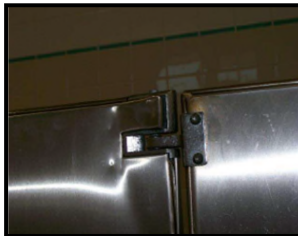
Partition door will not open properly because of damaged hinge and would not meet desired maintenance conditions.
