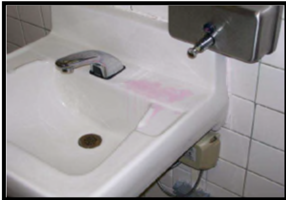
The above soap dispenser has a leak and would not meet desired maintenance conditions.
