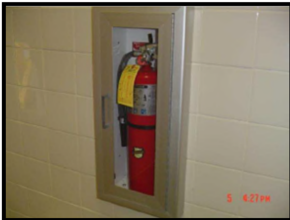
Extinguisher in proper cabinet with inspection sticker available meets desired maintenance conditions.
