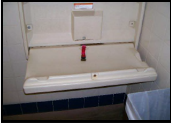
Changing table with missing or broken strap would not meet desired conditions.
