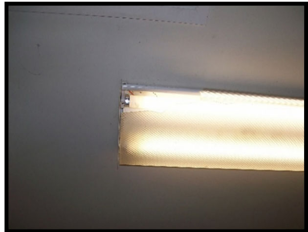
This light has a cracked and broken light cover/diffuser and would not meet desired maintenance conditions.
