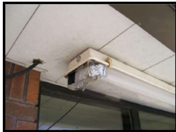
This fixture has a cracked/broken lens and would not meet the desired maintenance conditions.
