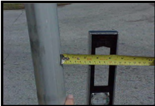
This signpost is leaning more than 1 inch per foot and would not meet the desired maintenance conditions.
