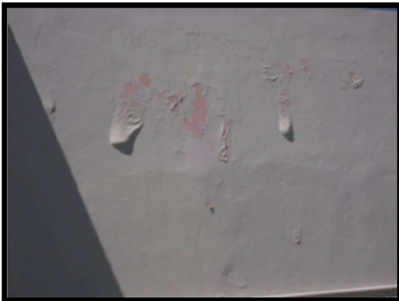
A wall with blistered and peeling paint would not meet desired maintenance conditions.
