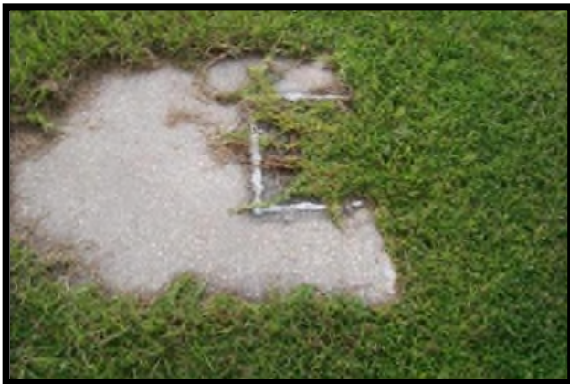
Buildup of grass and dirt in this paved ditch would not meet desired maintenance conditions for miscellaneous drainage.
