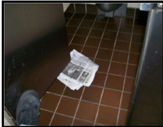
Trash and debris on floor may create a trip hazard and would not meet desired maintenance conditions.
