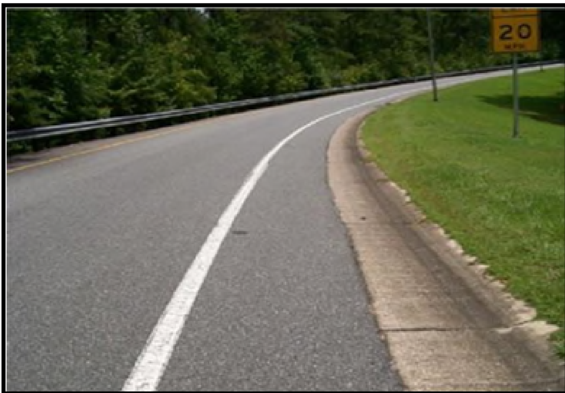
Example of missing RPMs on ramp edge line striping. This does not meet desired maintenance conditions.
