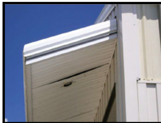
Soffit needs to be repaired and cleaned. This does not meet desired maintenance conditions.
