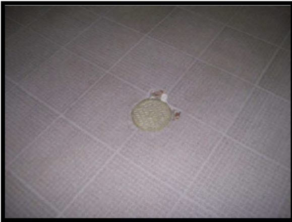
Broken tile greater than \frac{1}{4} inch in depth around floor drain would not meet desired maintenance conditions.
