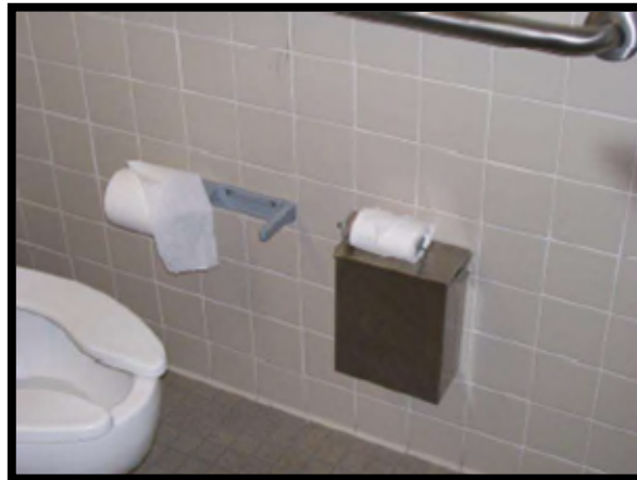
This dispenser is not in working order and would not meet desired maintenance conditions.
