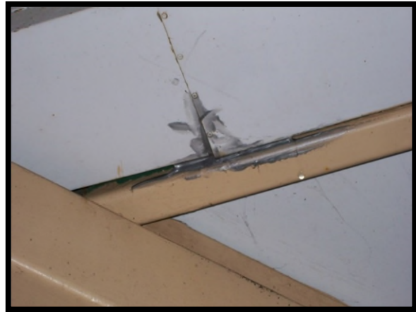
Example of a ceiling where a leak was improperly patched. This would not meet desired maintenance conditions.
