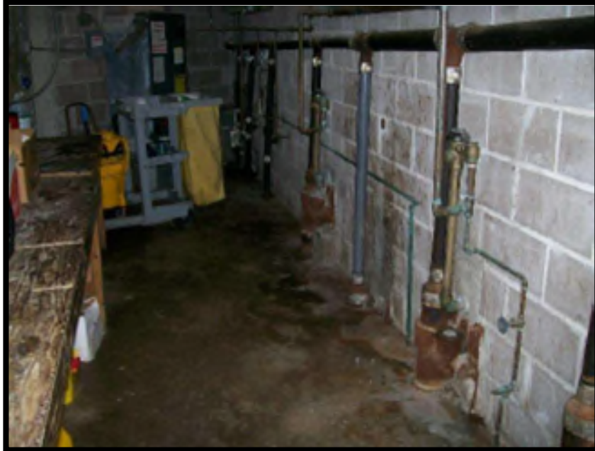
Plumbing stacks leaking, cleaning cart blocking the electrical panel box, this would not meet desired maintenance conditions.
