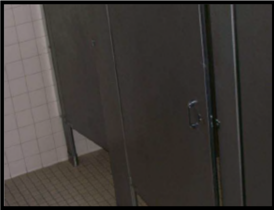
This door has a broken latch and would not meet desired maintenance conditions.
