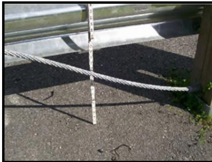
The cable is not taut and may deviate more than 1 inch, this may not meet desired maintenance conditions.
