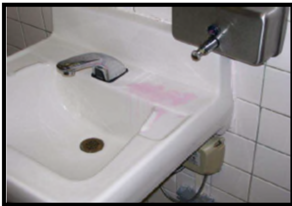
The above soap dispenser has a leak and would not meet desired maintenance conditions.
