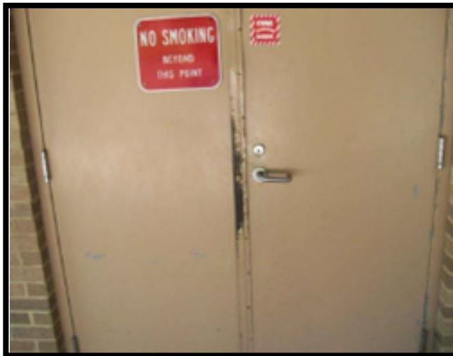
This door is to a restricted area and should remain locked when not in use to meet desired maintenance conditions.
