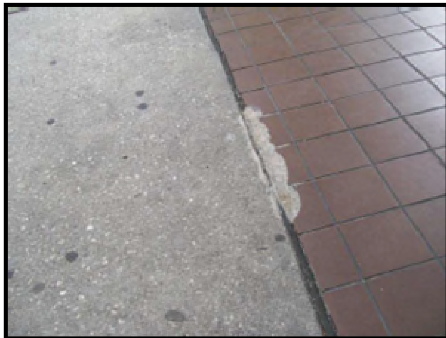
Misaligned/broken tiles could be a trip hazard and does not meet desired maintenance conditions.
