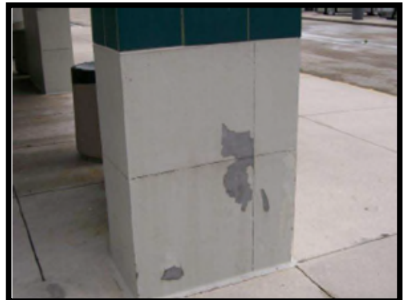
Example of a wall with peeling paint. Depending on the percentage of the walls in this condition, there is a possibility this facility would not meet desired maintenance conditions.
