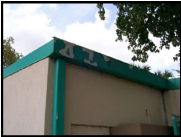
This gutter system should be painted to meet desired maintenance conditions.
