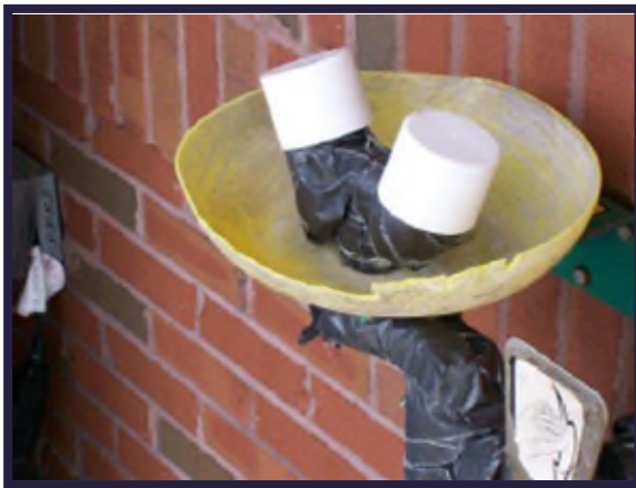
Broken or deteriorating plastic on eyewash station would not meet the desired maintenance conditions.
