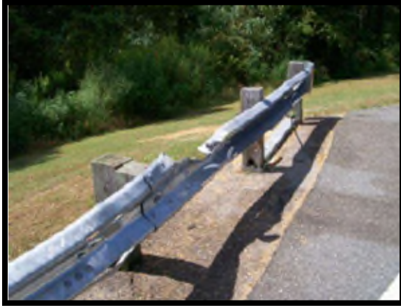
A damaged guardrail would not meet desired maintenance conditions.
