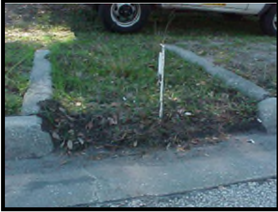
Edge drains are rated as miscellaneous drainage and 90% should be unobstructed with a hardware cloth in place to meet desired maintenance
