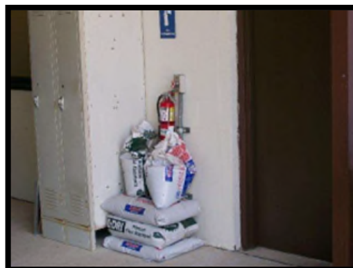
Materials stacked in front of fire extinguisher would not meet desired maintenance conditions.
