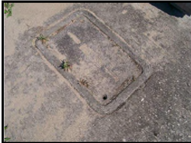
Cover lids are to be properly secured with bolts if lid is designed to have bolts to meet desired maintenance conditions.
