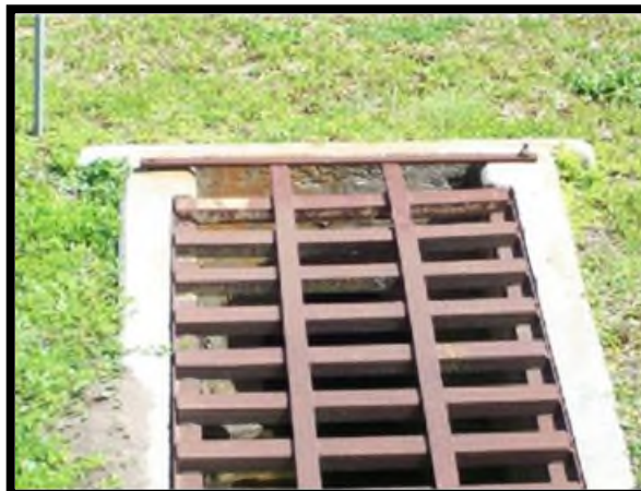
Grate missing hardware, an anchor bolt in the corner, this would not meet desired maintenance conditions.
