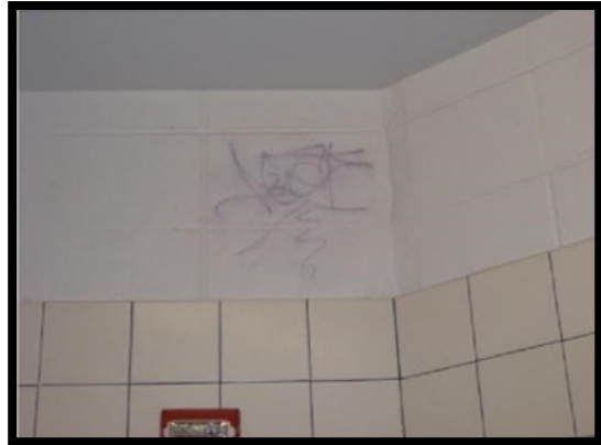
Graffiti on walls would not meet desired maintenance conditions.
