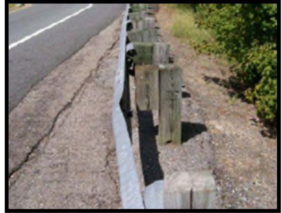
A damaged guardrail that is pulled away from the block, would not meet desired maintenance conditions.
