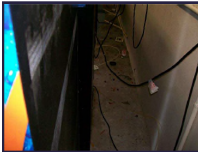
Behind the vending machines should be clean. This does not meet desired maintenance conditions.
