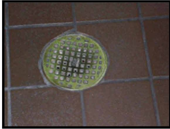
A blocked floor drain would not meet desired maintenance conditions.
