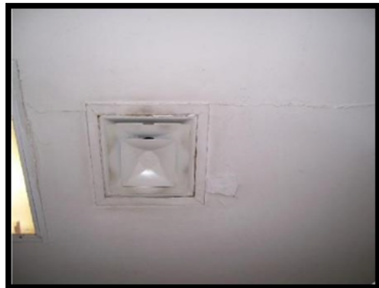
Ceiling with a dirty stained vent with cracked and peeling paint would not meet desired maintenance conditions.
