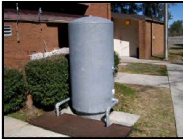
Water supply/treatment tank meets the desired maintenance conditions.
