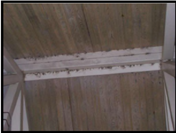
A ceiling with cobwebs would not meet desired maintenance conditions.
