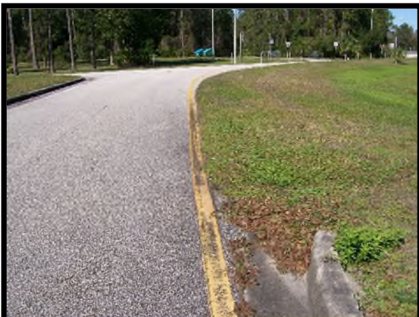
Example of striping that would not meet the desired maintenance conditions.
