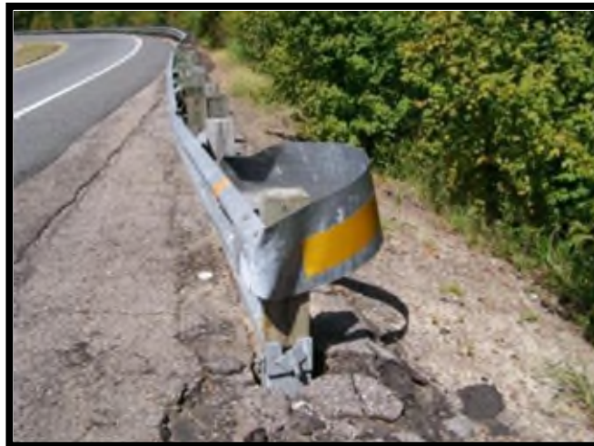
A damaged end section would not meet desired maintenance conditions.
