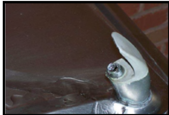
This water fountain will not shut off and would not meet desired maintenance conditions.
