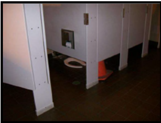
The toilet in this stall is missing and would not meet desired maintenance conditions.
