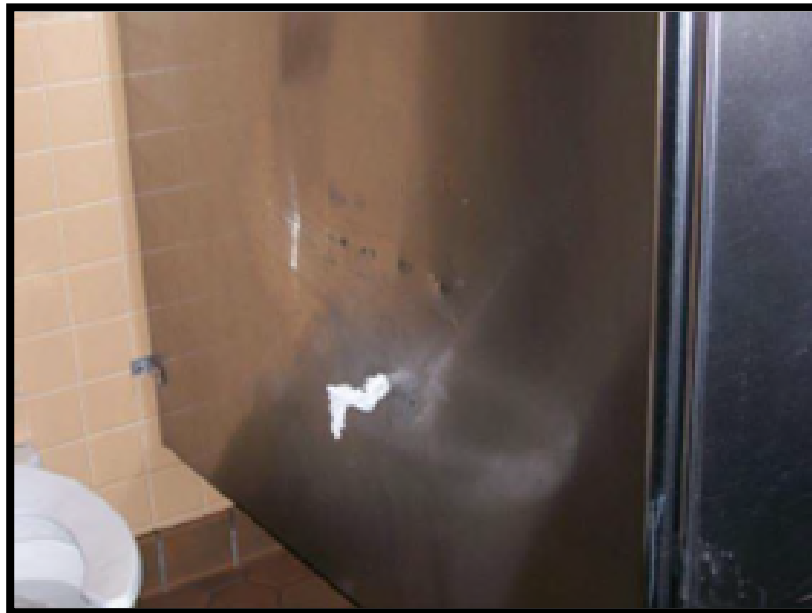
The partition surface has holes, rough edges, and would not meet desired maintenance conditions.
