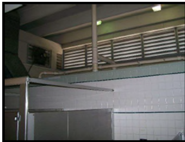
Buildup of dust on top of wall and pipe. This would not meet desired maintenance conditions.
