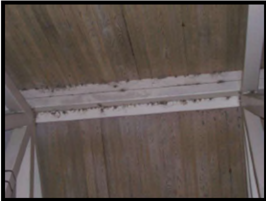
Cobwebs on ceiling would not meet desired maintenance conditions.
