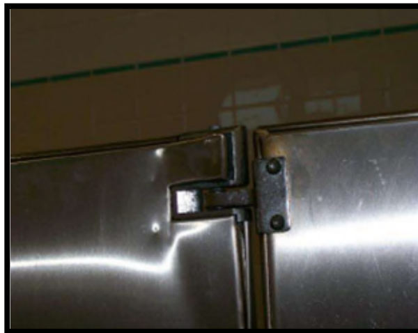
Partition door will not open properly because of damaged hinge and would not meet desired maintenance conditions.
