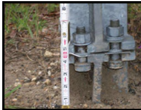
The slip base on this sign is more than 4 inches above grade and would not meet desired maintenance conditions.
