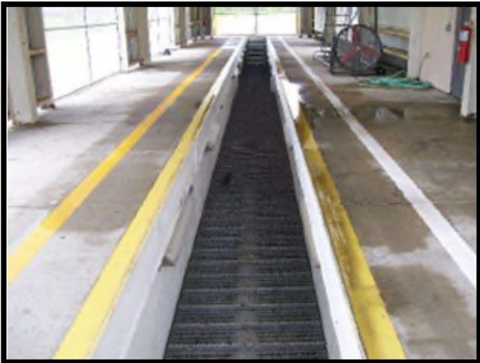
Inspection pit and ventilation system.
