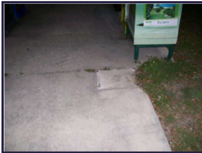
Receptacle has been removed but the anchor bolts left in place create a trip hazard. This would not meet desired maintenance conditions.
