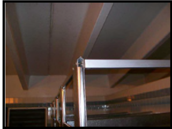
The frame is missing a trim end cap from the partition would not meet desired maintenance conditions.
