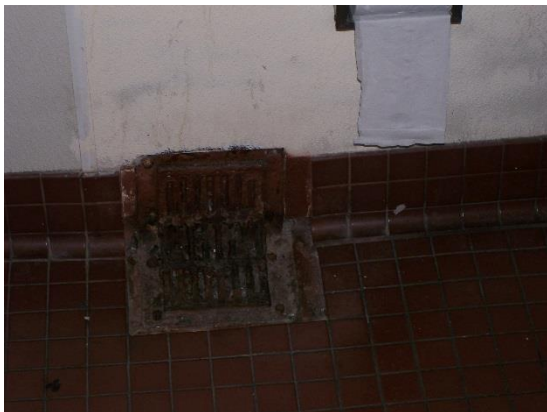
Rusted damaged floor drain this would not meet desired maintenance conditions.
