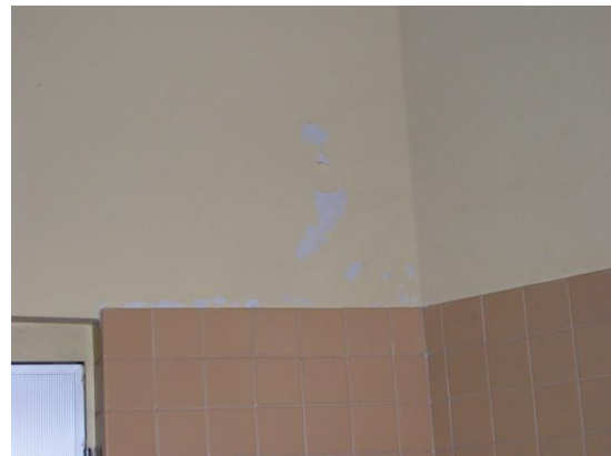
Example of peeling paint on wall.
