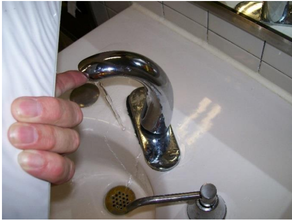
Loose damaged faucet would not meet desired maintenance conditions.
