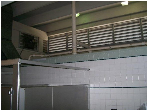
Build-up of dust on top of wall and pipe this would not meet desired maintenance conditions.
