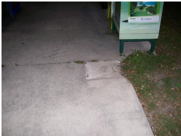
Receptacle has been removed, but anchor bolts left in place create a tripping hazard. This would not meet desired maintenance conditions.
