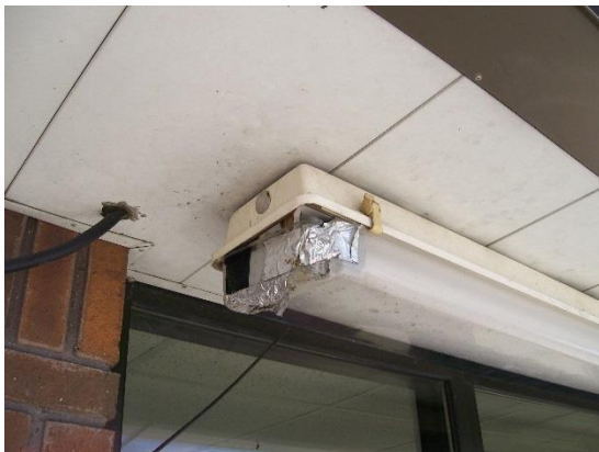
This fixture with a cracked/broken lens would not meet desired conditions.
