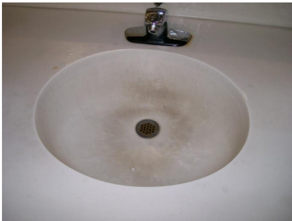
This basin is stained and would not meet desired maintenance conditions.
