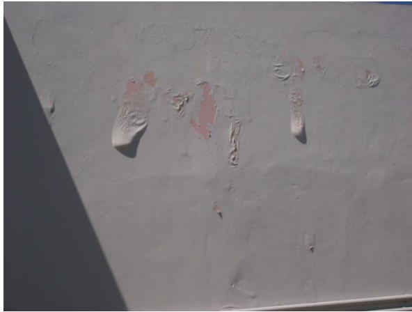
Wall with blistered and peeling paint, this possibly would not meet desired maintenance.
