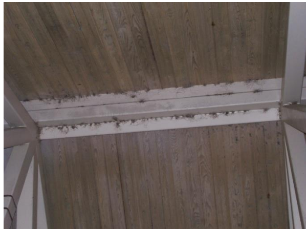
Ceiling with cobwebs requires cleaning.
