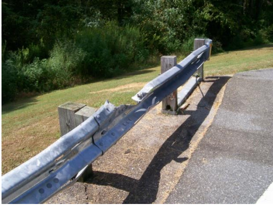
Damaged guardrail, this would not meet desired maintenance conditions.
