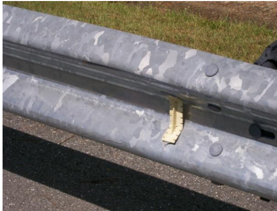
Missing hazard markers reflectors, this may not meet desired maintenance conditions.
