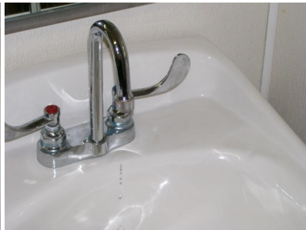
This faucet is leaking and would not meet desired maintenance conditions.
