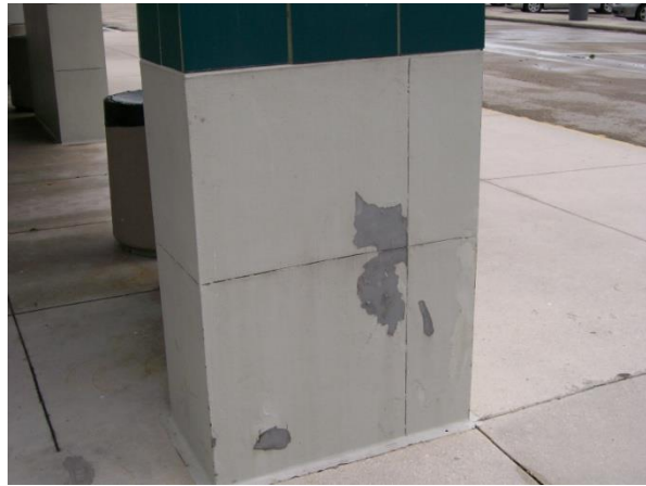
Wall with peeling paint, this might not meet desired maintenance conditions.
