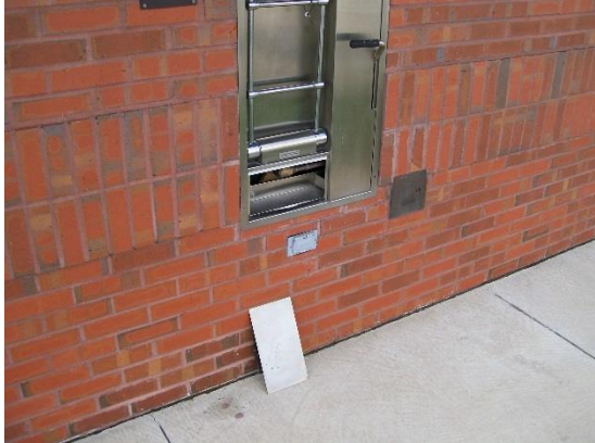
Missing door/covers would not meet desired maintenance conditions
