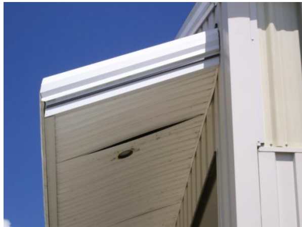
Soffit need to be repaired and cleaned.
