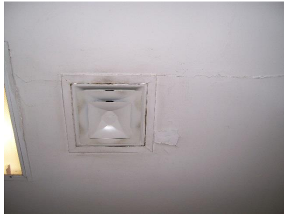
Ceiling with a dirty, stained vent with cracked and peeling paint would not meet desired conditions.
