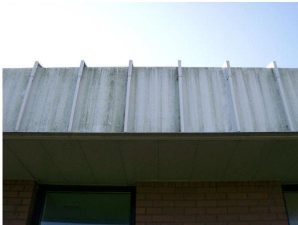
Roof/Fascia has dirt and mildew build-up.
