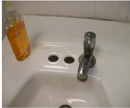
These holes should be covered or plugged and would not meet desired maintenance conditions.
