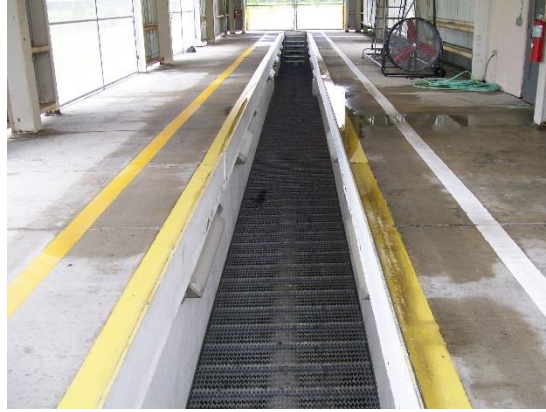
Inspection pit and ventilation system.
