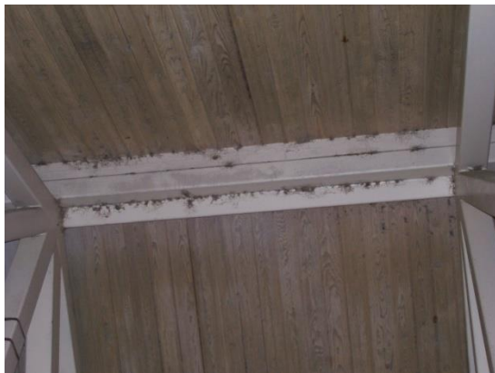
Example of cobwebs on ceiling.
