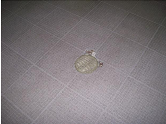
Broken tile greater than ¼ inch in depth around floor drain, this would not meet desired maintenance conditions.
