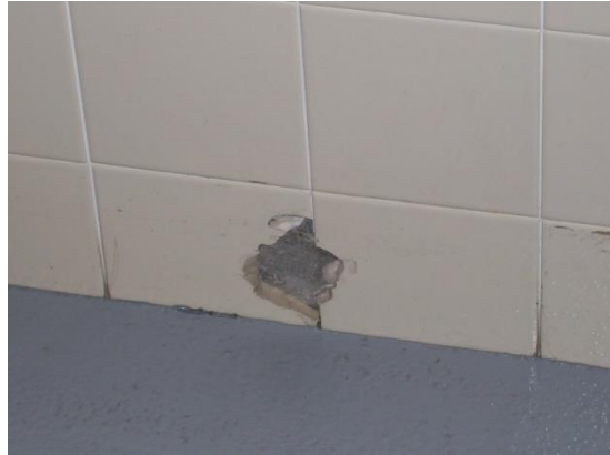
Example of broken tile on wall. No sharp edges on tile.
