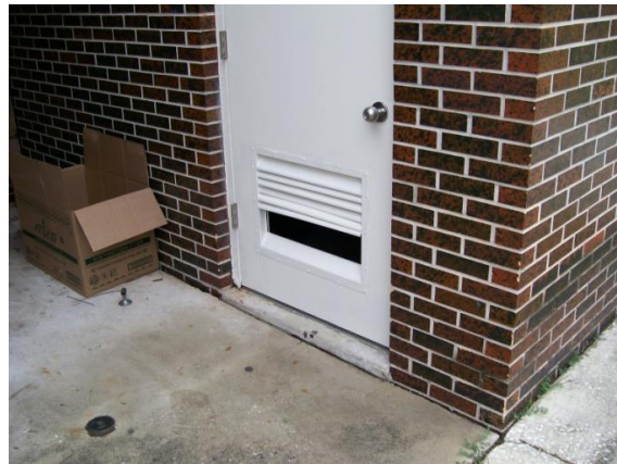
This door would not meet desired maintenance conditions.
