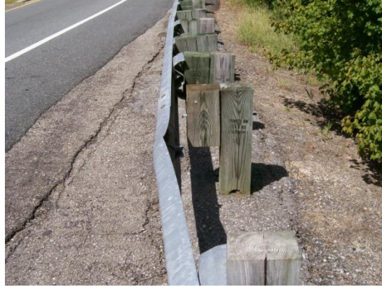
Damaged guardrail that is pulled away from the block, this would not meet desired maintenance conditions.
