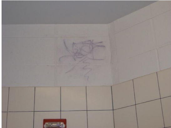
Example of graffiti on walls.
