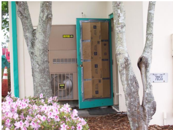
This door is missing the lock and would not meet the desired maintenance conditions.
