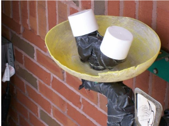
Broken or deteriorating plastic on eyewash station would not meet desired maintenance conditions.
