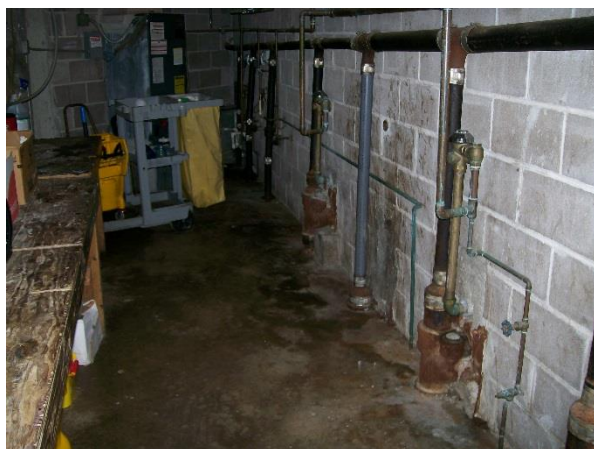
Plumbing stacks leaking also cleaning cart blocking the electrical panel box this would not meet desired maintenance conditions.
