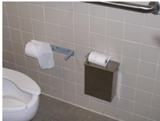
This dispenser is not in working order and would not meet desired maintenance conditions.
