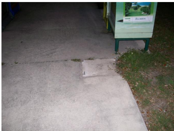
Receptacle has been removed, but anchor bolts left in place create a tripping hazard. This would not meet desired maintenance conditions.
