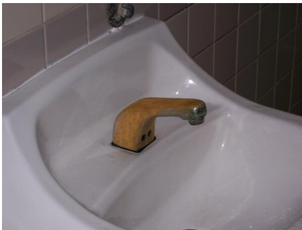
Faucet is corroded, and would not meet desired maintenance conditions.
