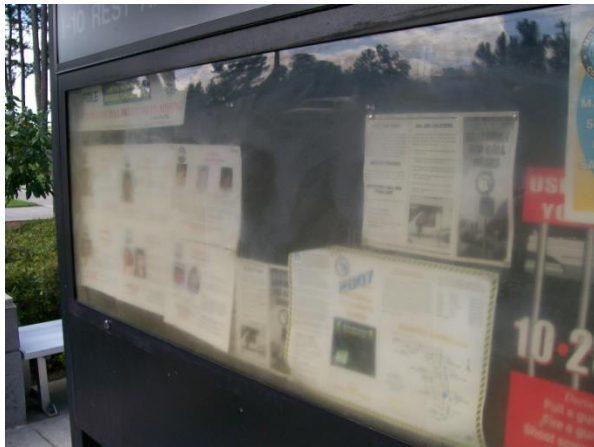
Bulletin board glass is fogged and/or scratched; this would not meet desired maintenance conditions.
