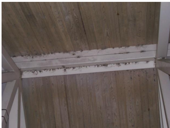
Example of cobwebs on ceiling.
