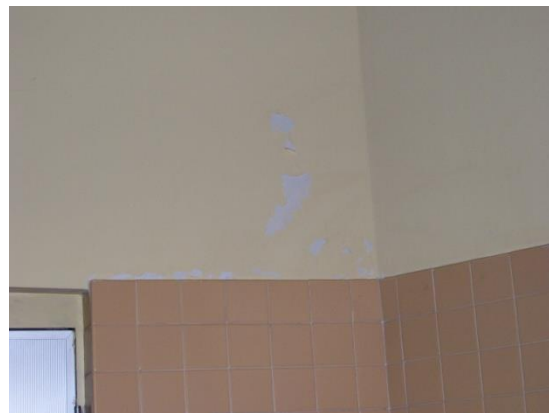
Example of peeling paint on wall.
