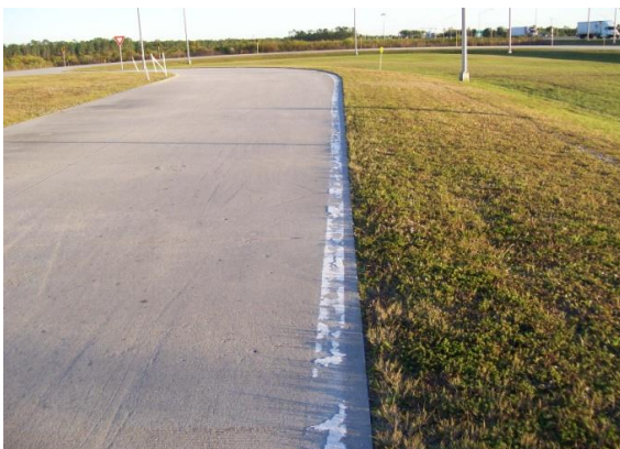
Example of striping that would not meet desired maintenance conditions.
