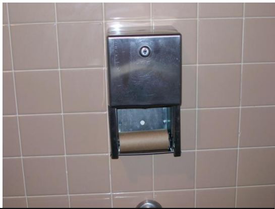
This dispenser is out of paper and would not meet desired maintenance conditions.
