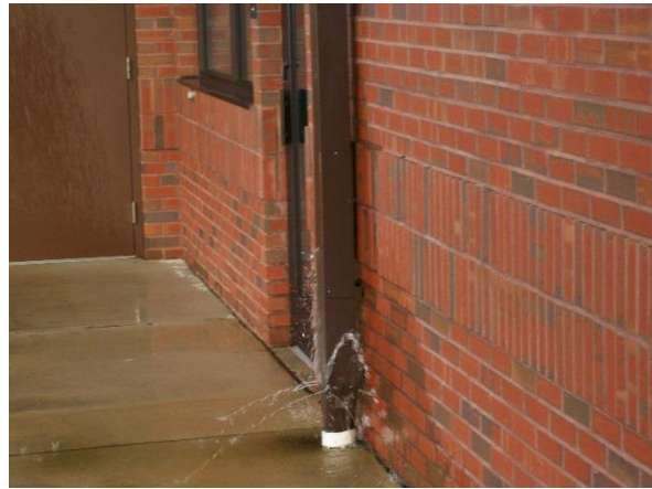
Gutter blocked and leaking this would not meet desired conditions.
