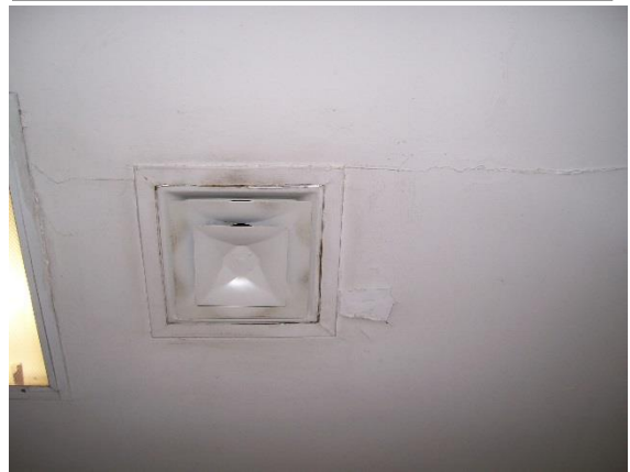
Ceiling with a dirty, stained vent with cracked and peeling paint would not meet desired conditions.
