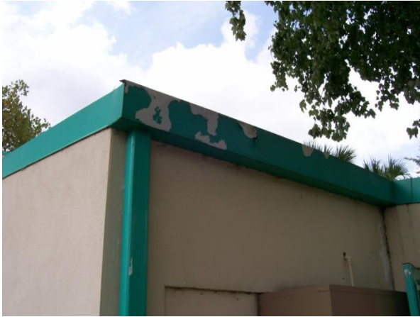
This gutter should be painted.
