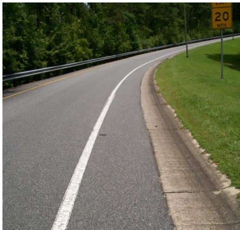
Example of missing RPMs on ramp edge line striping.
