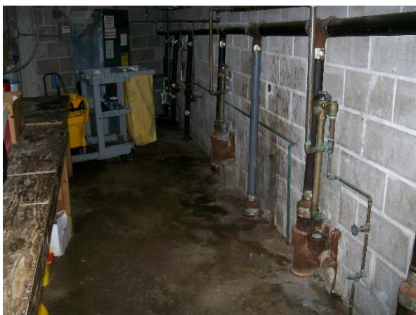
Plumbing stacks leaking also cleaning cart blocking the electrical panel box this would not meet desired maintenance conditions.
