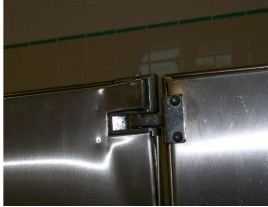
Partition door will not open properly because of damaged hinge
