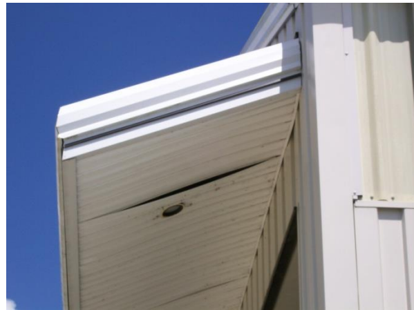
Soffit need to be repaired and cleaned.
