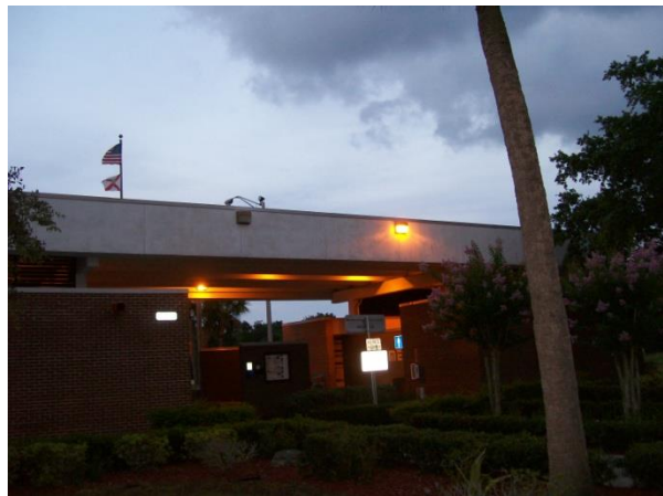
Example of building light not working. The lights under the roof will be included as foyer lighting.
