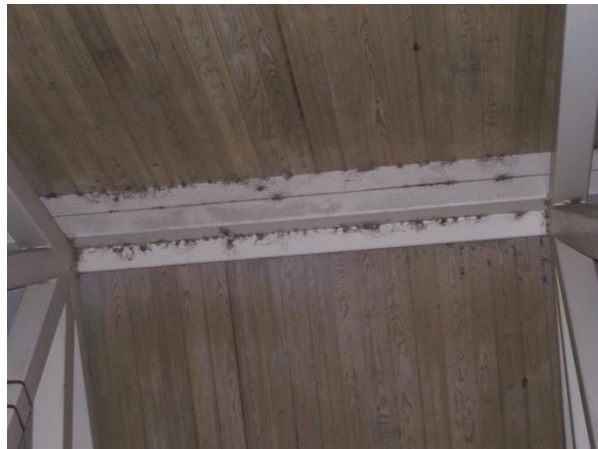
Ceiling with cobwebs requires cleaning.
