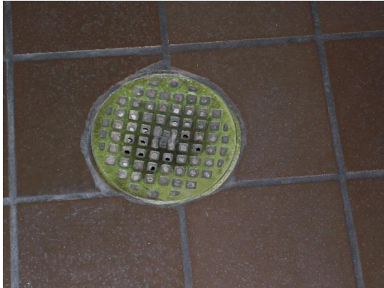
Blocked floor drain would not meet desired maintenance conditions.
