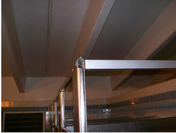
Missing trim end cap from partition would not meet desired conditions.
