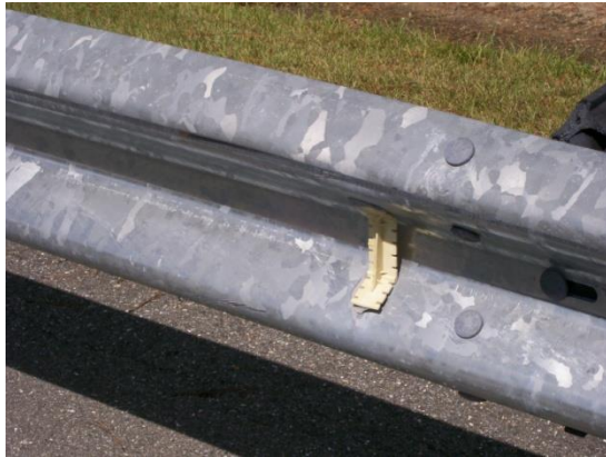
Missing hazard markers reflectors, this may not meet desired maintenance conditions.
