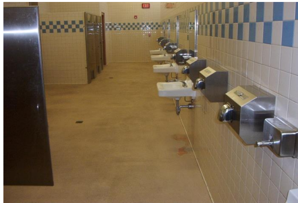
Test each hand dryer ensure they meet desired maintenance conditions.
