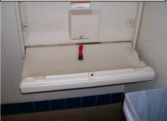
Changing table with missing or broken strap would not meet desired conditions
