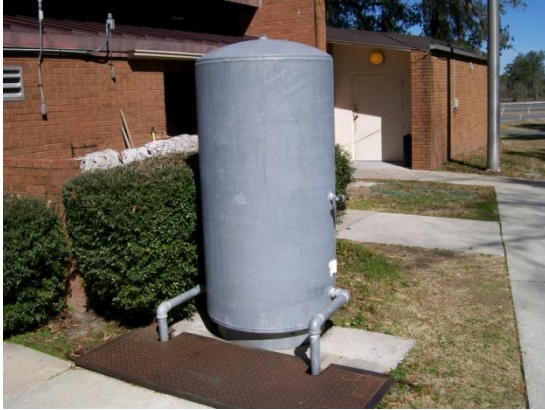
Photo of water supply/treatment.
