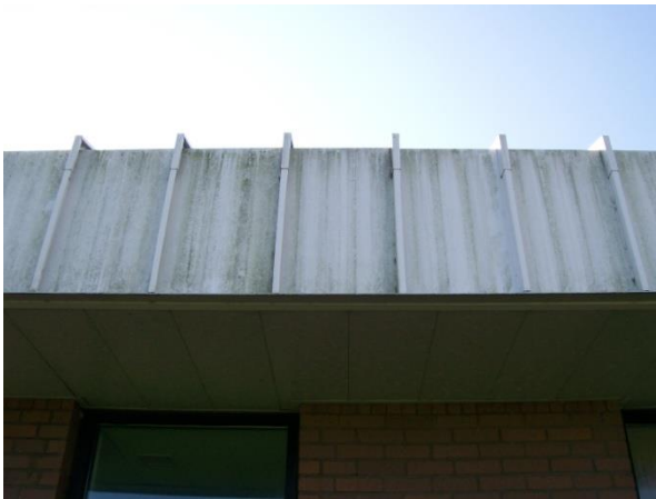
Roof/Fascia has dirt and mildew build-up.
