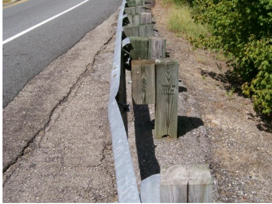
Damaged guardrail that is pulled away from the block, this would not meet desired maintenance conditions.
