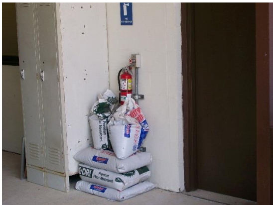
Materials stacked in front of fire extinguisher would not meet desired maintenance conditions
