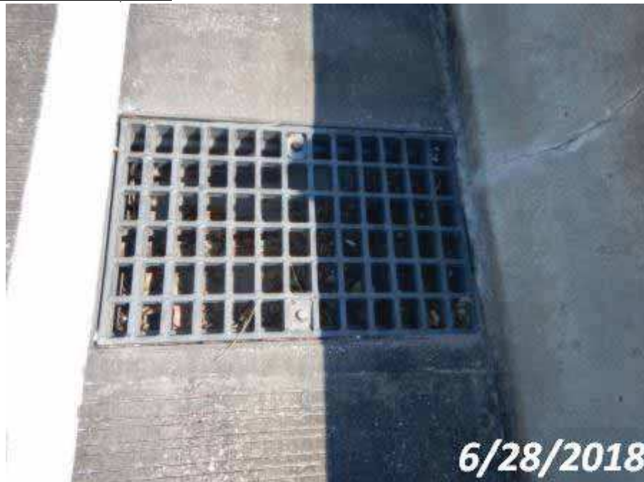
Photo 8398-S01 (Unit 0: Drainage System - Other)
