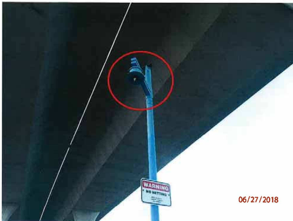
Photo 5: Structural Notes: Showing missing luminaries assembly at post 13.
