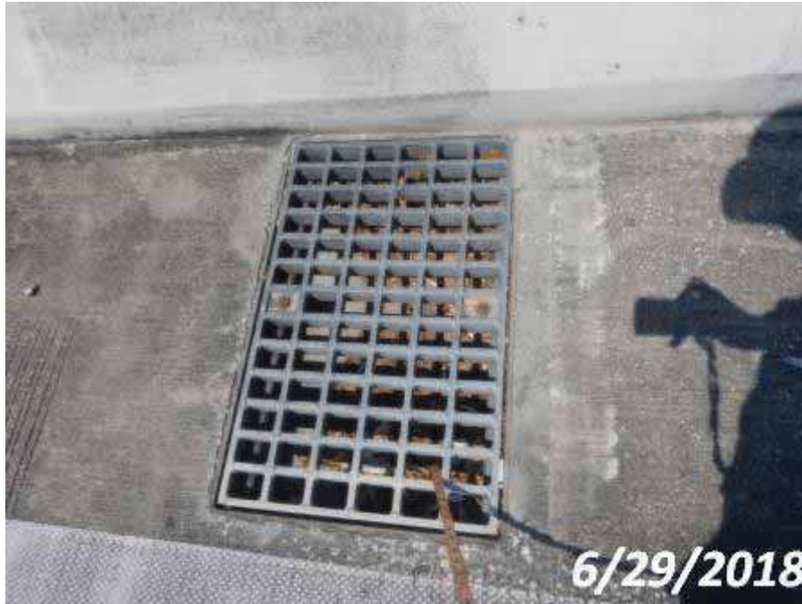
Photo 8398-S01 (Unit 0: Drainage System - Other)
