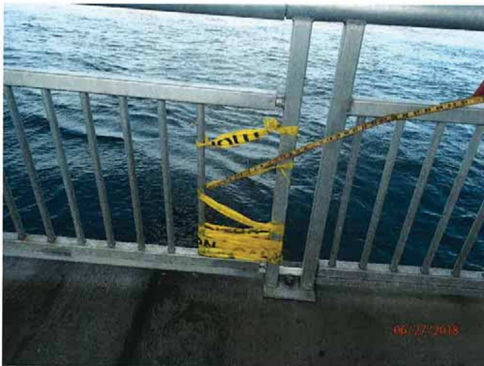
Photo 2: Structure Notes: Showing right rail missing Pickett.
