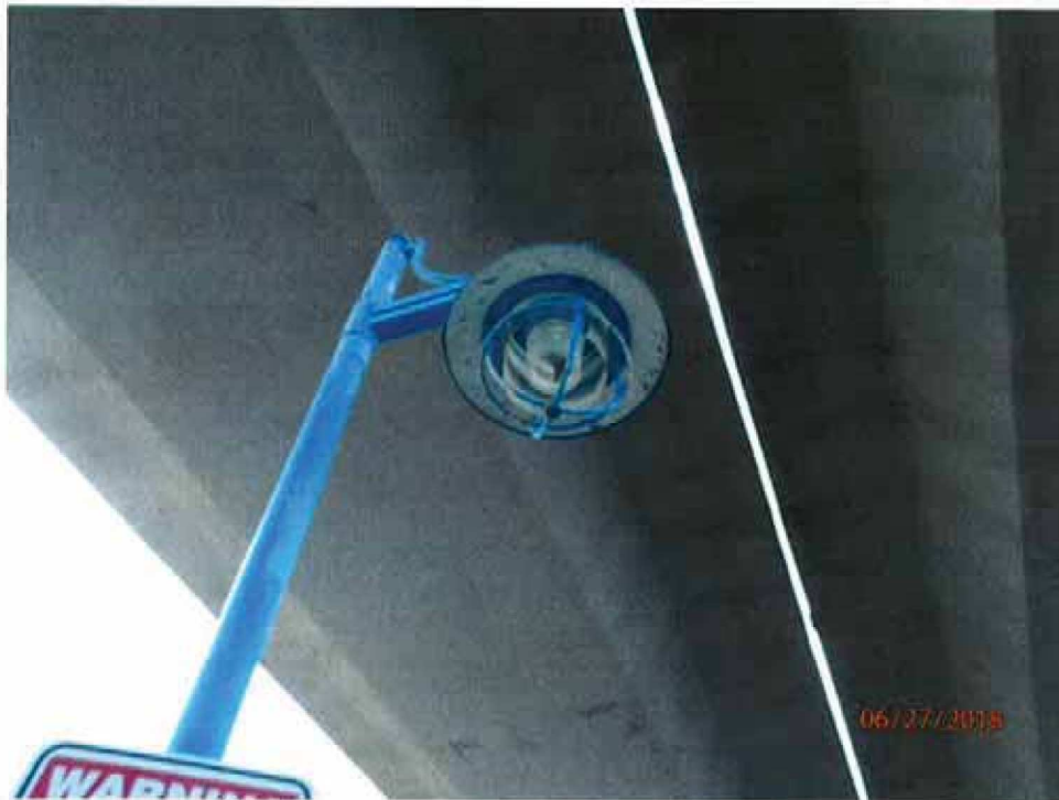
Photo 4: Structure Notes: Showing broken/missing lens at light post 5.
