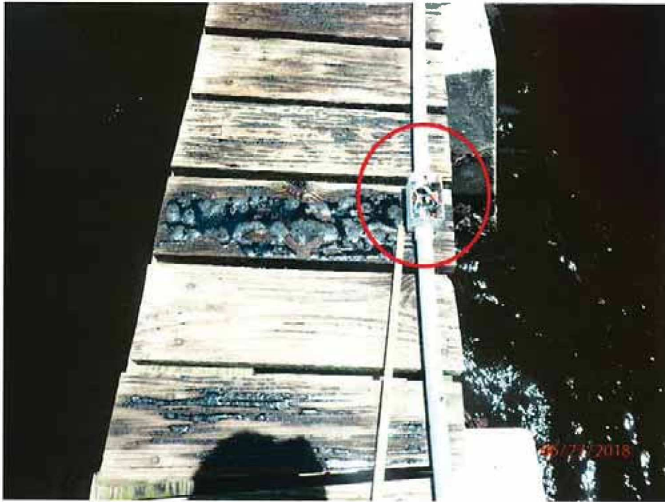
Photo 1: Element 8387: Showing south fender section 3 missing J-Box cover.
