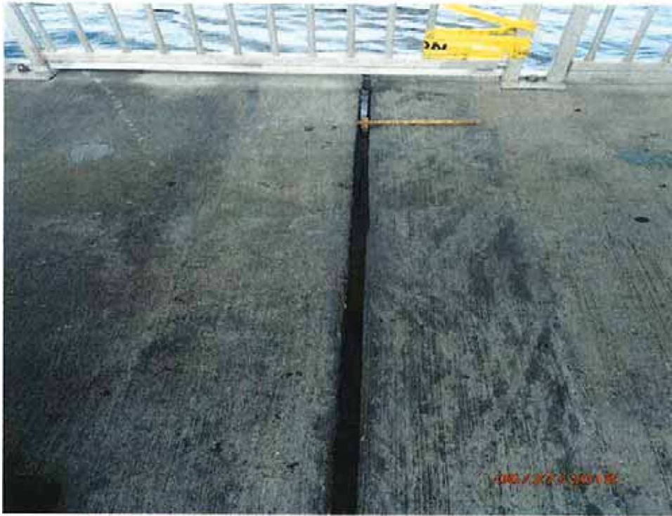
Photo 3: Structure Notes: Showing typical joint condition at fishing piers.
