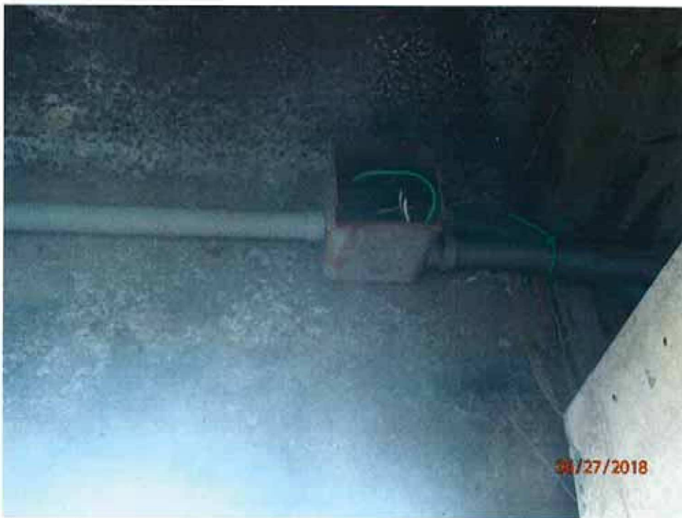
Photo 6: Structural Notes: Showing exposed wires at J-Box covers.
