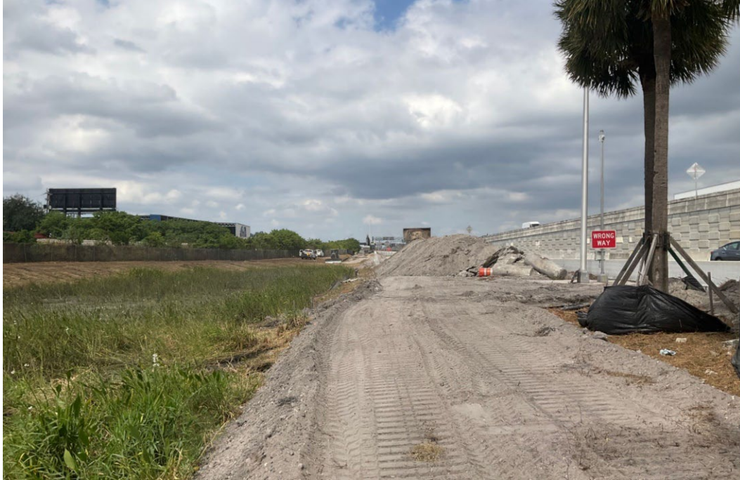
Figure 4. Northern half of the APE at intersection of Griffin Road and S.R. 9, facing north showing active construction zone.
