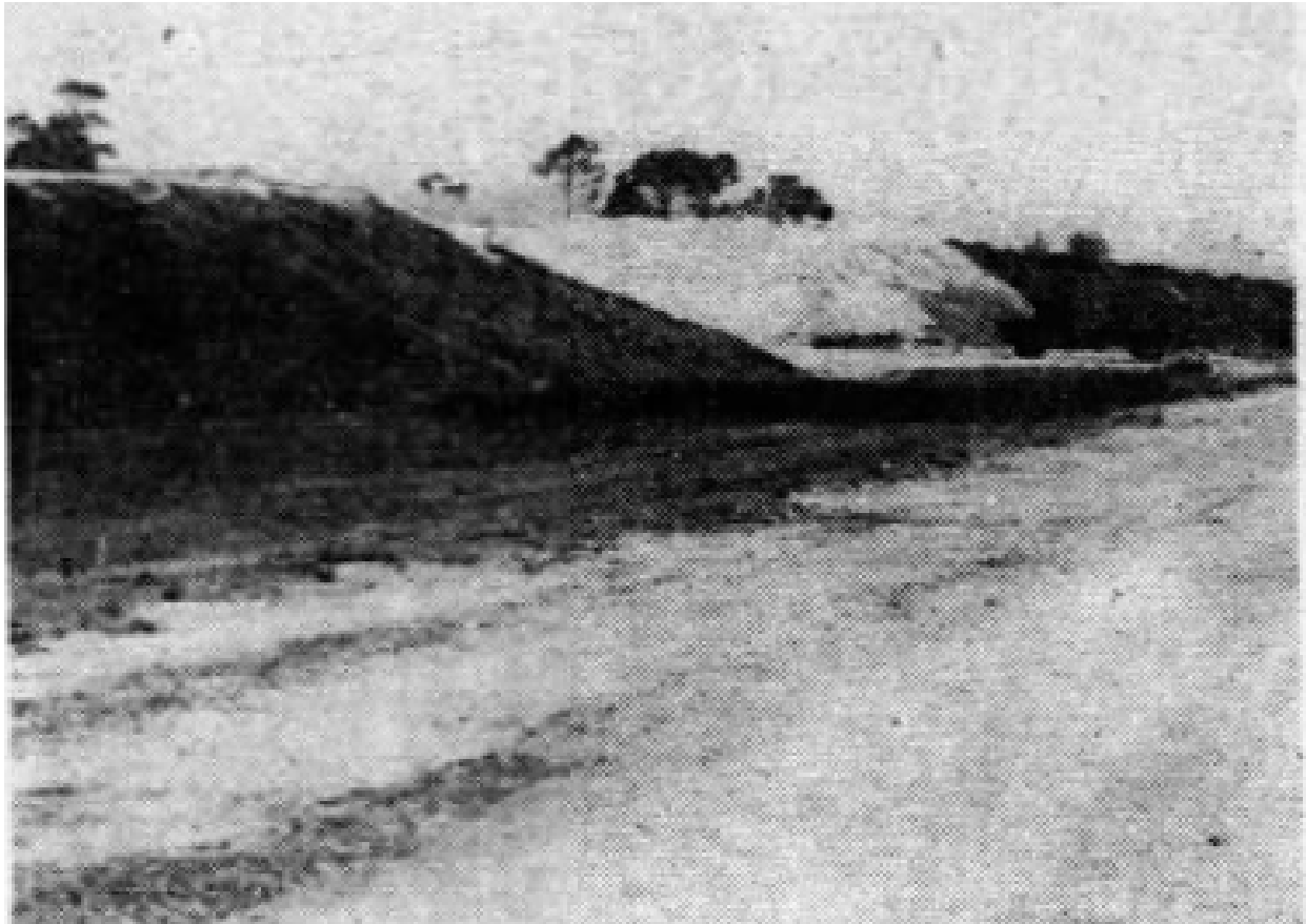
Figure 9. Excerpt from the Miami News showing construction of the S.R. 9 overpass over Hollywood Boulevard (near center of APE) (Miami News, 27 April 1952a:17).
