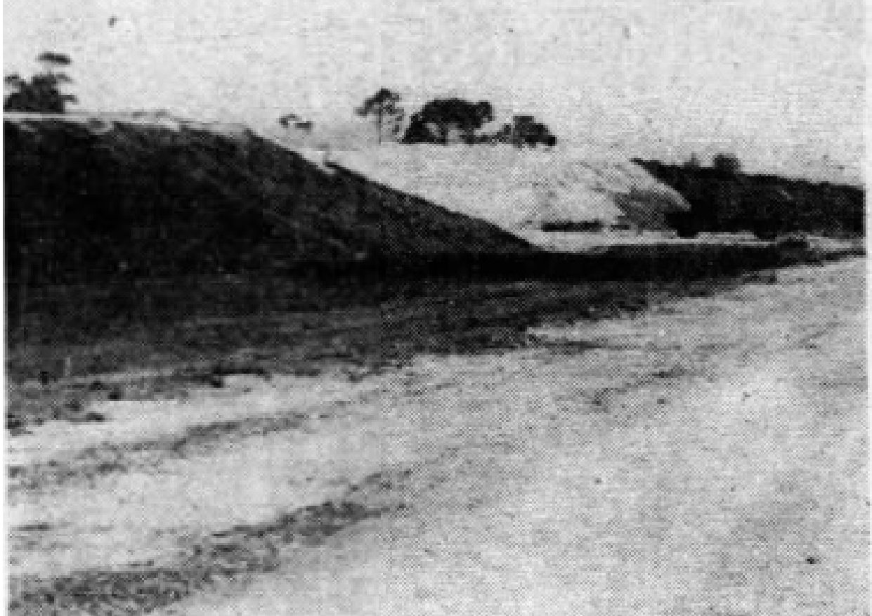
Figure 8. Excerpt from the Miami News showing construction of the S.R. 9 overpass over Hollywood Boulevard (Miami News, 27 April 1952a:17).
