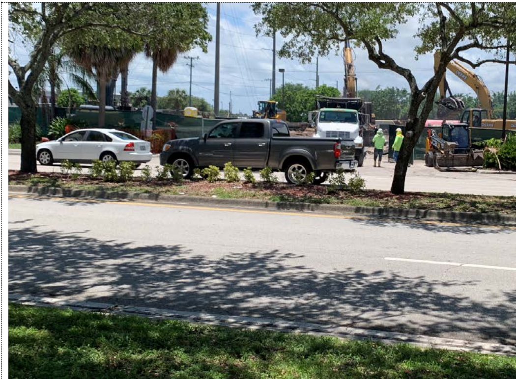
Photo 8 – View of Racetrac #459 site, 905 W. Woolbright Rd., facing north, showing ongoing construction activities.
