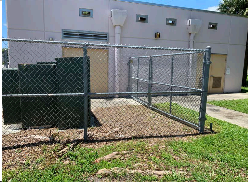
Photo 5 – View of generator and associated tank located in the rear of Forest Park school building.
