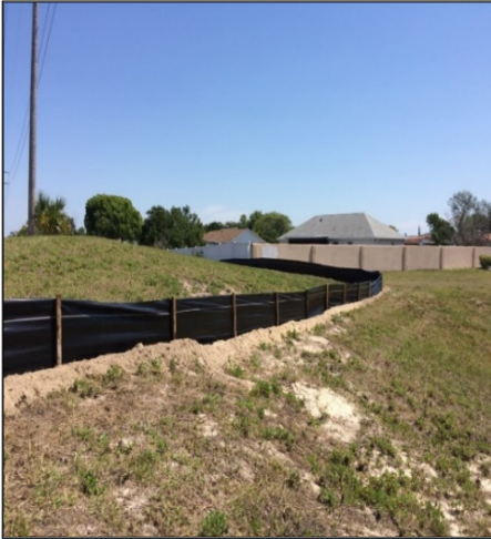
Plate 9: Correctly installed exclusionary silt fence.
