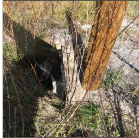
Plate 10: Incorrectly installed exclusionary silt fence with open gap.
