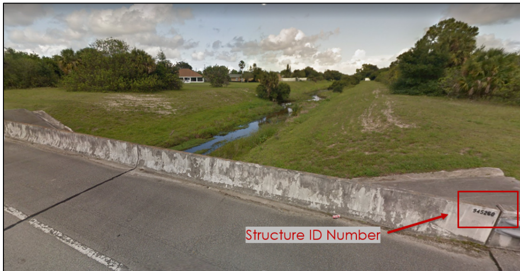
FIGURE 8 –Bridge ID Number Example; # 945260, District Four, Port St. Lucie Blvd., St. Lucie County
