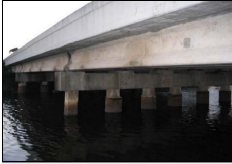
PHOTO 20 - Access Issue - Low Continuous concrete multibeam bridge over water.
