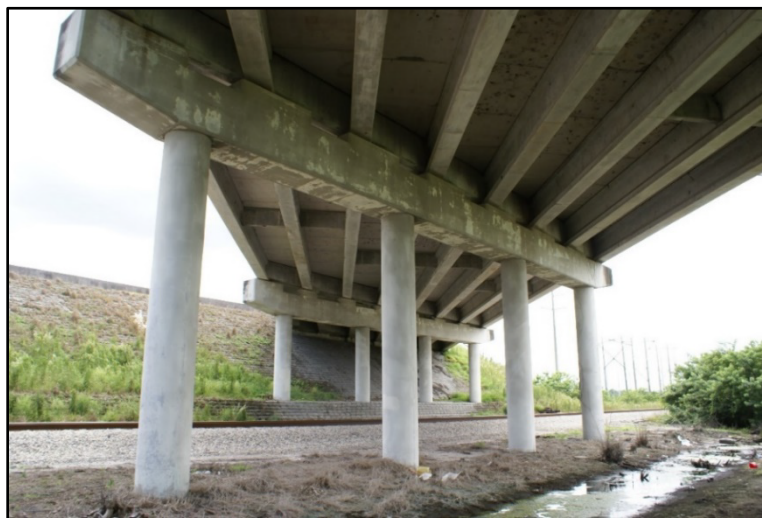
PHOTO 22 – Bat Exclusion (2019), Fly By Night , on I-95 Bridge over the FEC rail line and CR 709, Martin County, District Four.
