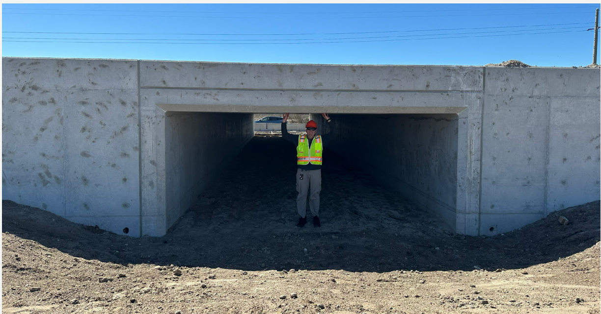
Completed 16-foot x 6.5-foot wildlife crossing on SR 82 near proposed Corkscrew Groves.
