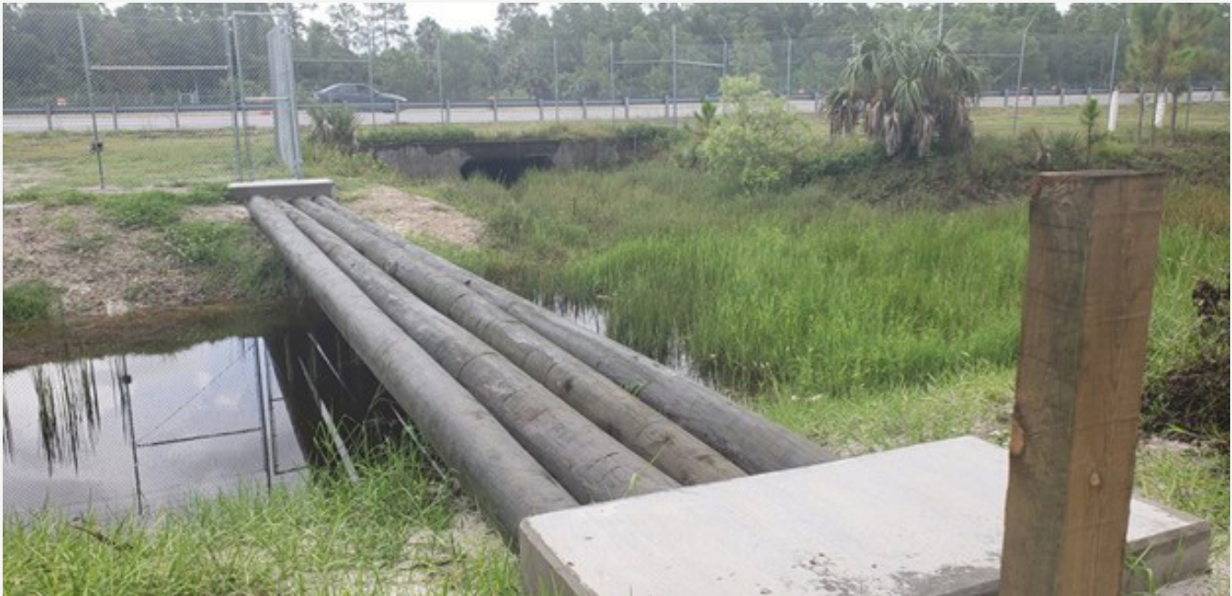
One of three new timber bridges on the south side of I-75/Alligator Alley.
