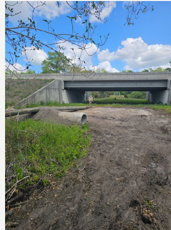
Culvert under wooden pile bridge walkway added to SR 29 Pistol Pond Crossing.
