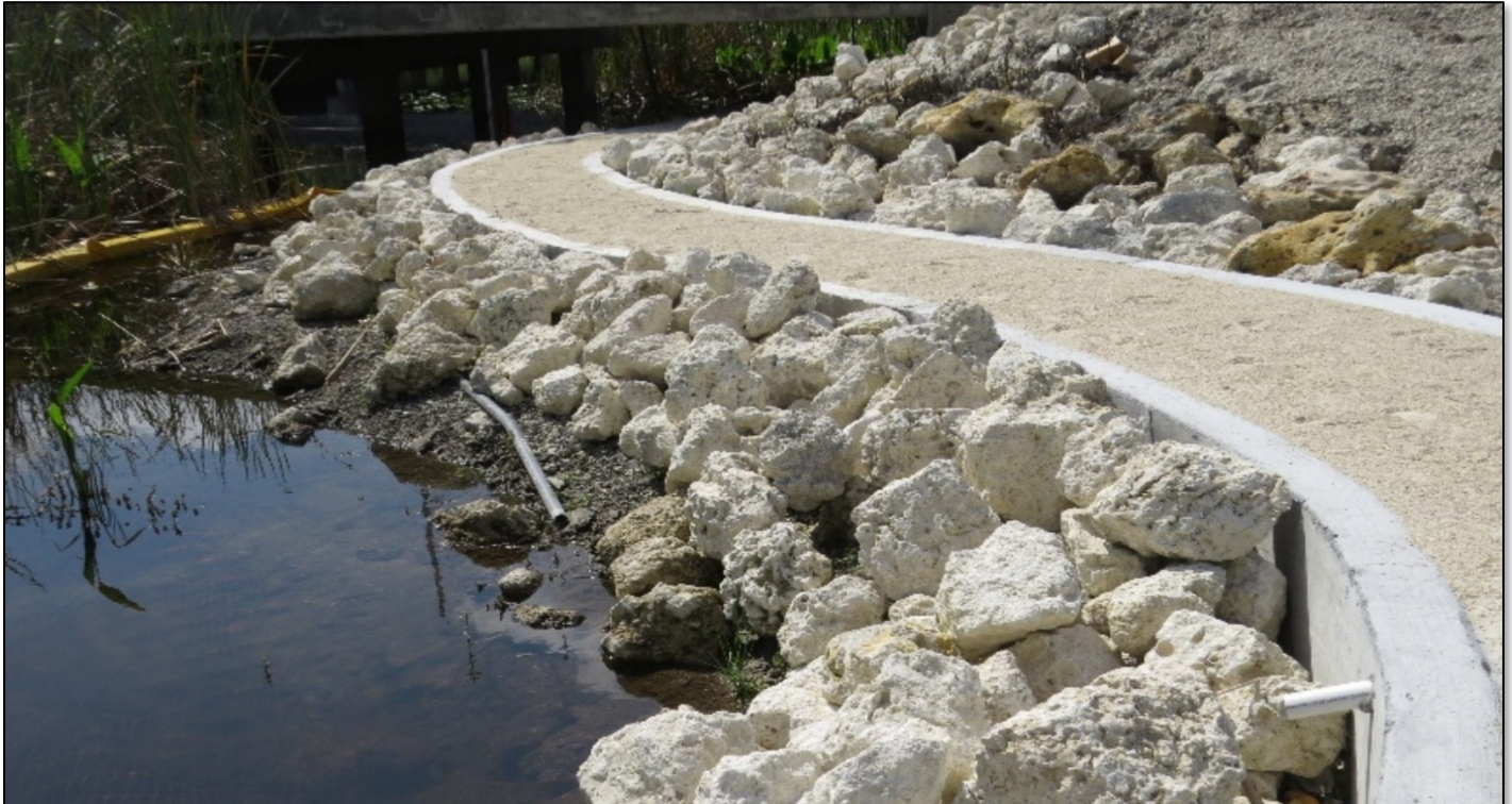
Figure 16 Example of a Crossing Retrofit: A dry shelf with a pathway to transition between end of dry shelf and natural ground at Harold Strand, I-75 Alligator Alley, Collier County, D1 (FPID 444008-2). PVC pipe in right foreground is a drainage feature for the walking surface.
