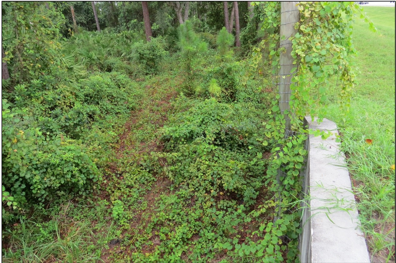
Figure 63 View of the landing area behind concrete barrier wall and wildlife fence for a jump out, I-4, Volusia County, D5 (FPID 408464-1). In this photograph, the roadway side is on the right and the off-site side is on the left.
