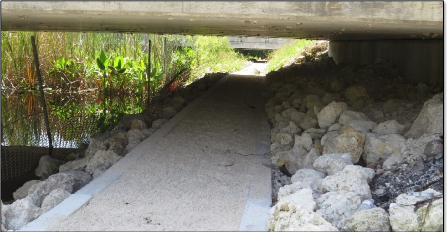
Figure 15 Dry shelf retrofit of a crossing at Harold Strand, I-75 Alligator Alley, Collier County, D1 (FPID 444008-2). The concrete retaining edges retain the natural walking surface.
