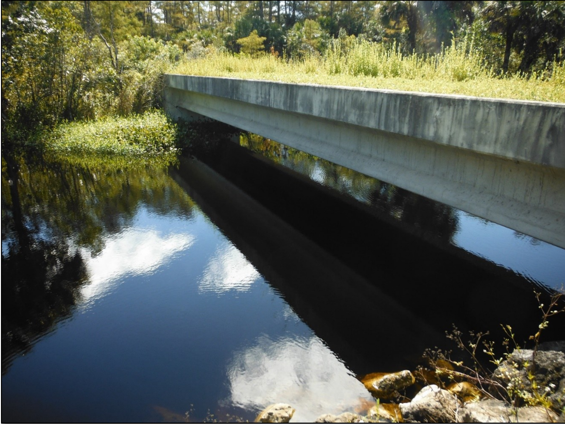
Figure 37 Concrete FIB structure with natural walking surface, SR 29, Collier County, D1 (FPID 407940-1).
