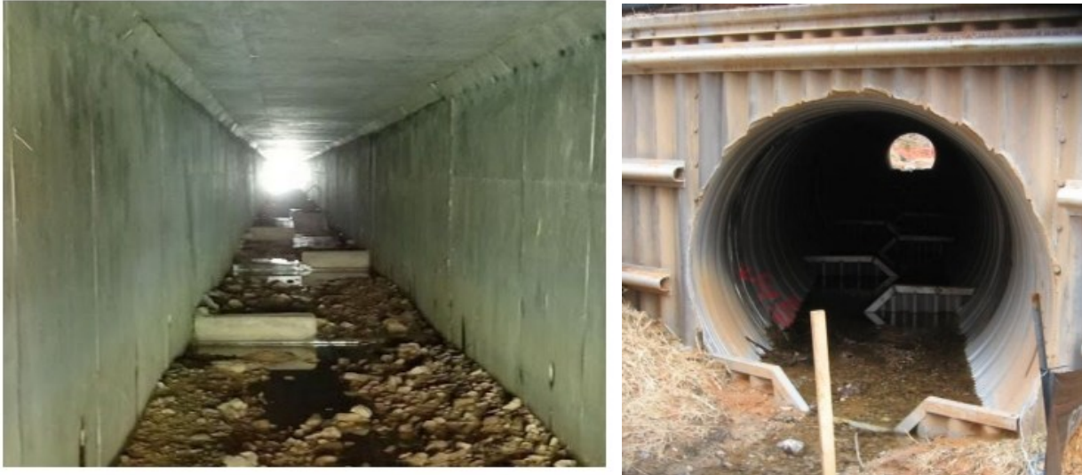
Figure 33 Culverts with baffles.
