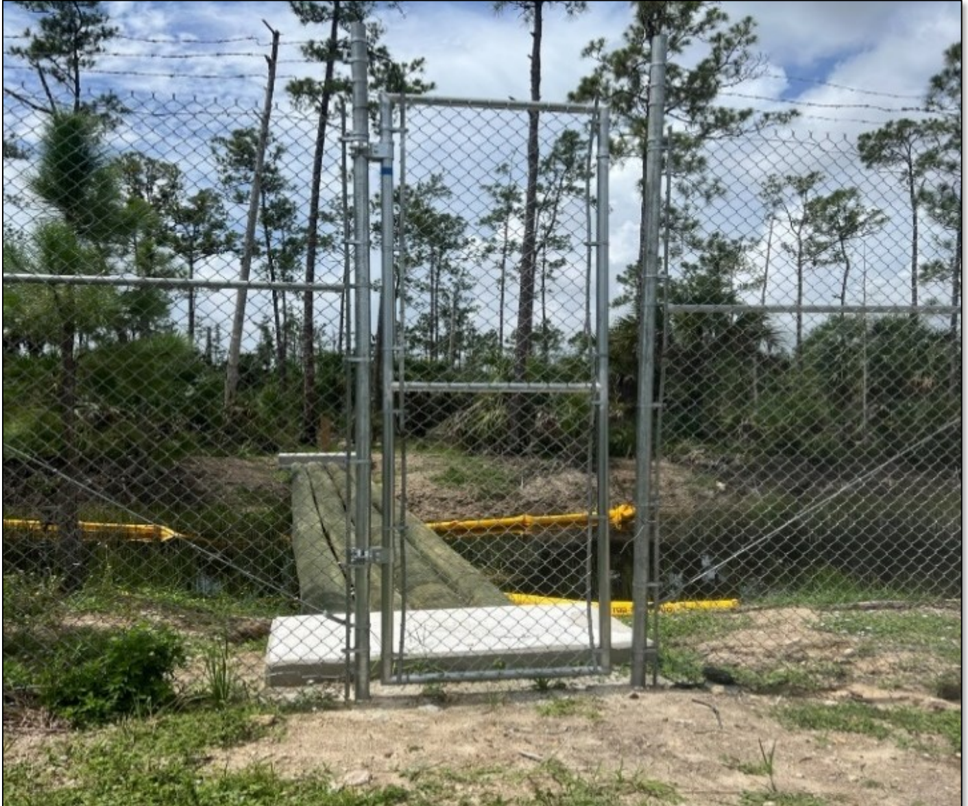
Figure 57 Three-foot-wide swing gate for maintenance and monitoring, I-75 Alligator Alley, Collier County D1 (FPID 405882-3).
