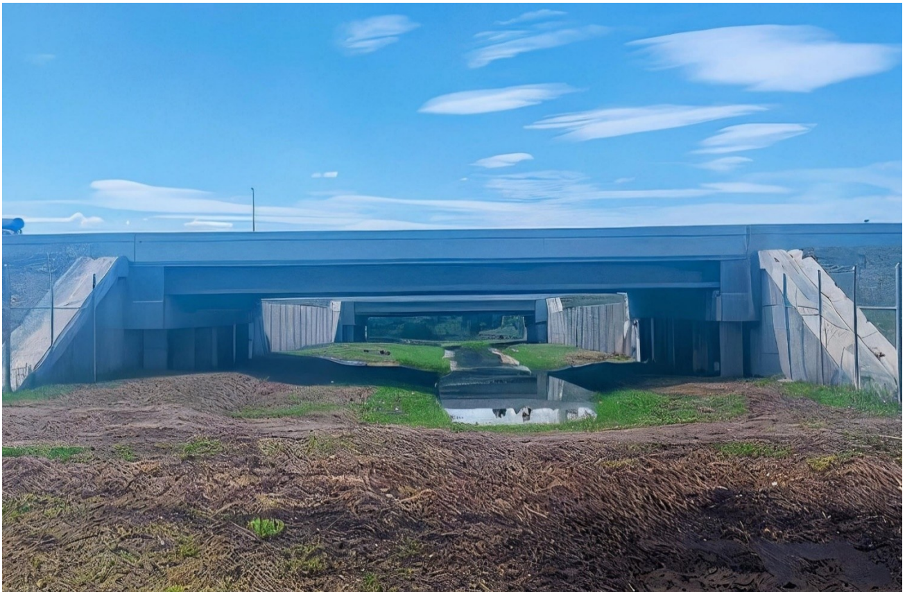
Figure 10 A wildlife crossing under I-4 east of SR 557 interchange, Polk County, D1 (FPID 201215-3). Dry crossing is provided along both sides with an aquatic feature in the center for wetland-dependent species.
