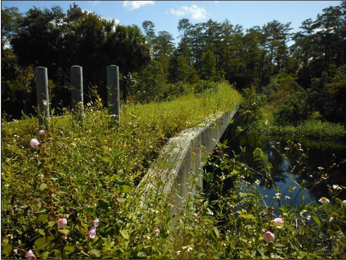
Figure 36 Concrete FIB structure with natural walking surface and bollards, SR 29, Collier County, D1 (FPID 407940-1).
