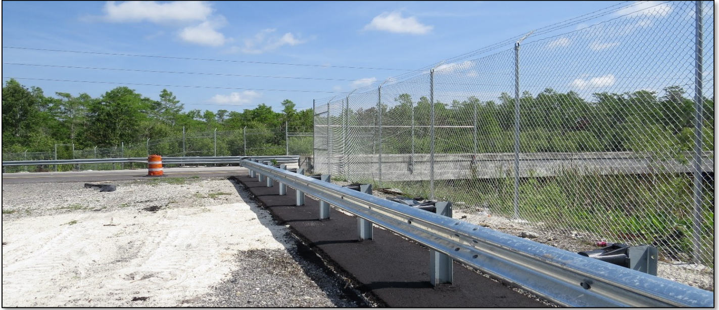
Figure 53 View within the median of a ten-foot chain link wildlife fence attached to a bridge on I-75 Alligator Alley, Collier County, D1 (FPID 405882-3).
