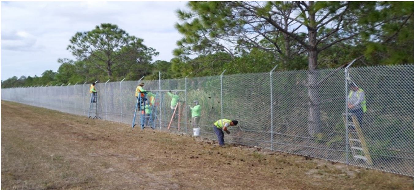
PHOTO -FDOT's 10-foot fencing along I-75/Alligator Alley
