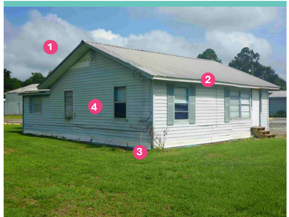
A Frame Vernacular Style Residence at 5271 Glover Lane (Santa Rosa County) constructed in 1957 (8SR2672)
