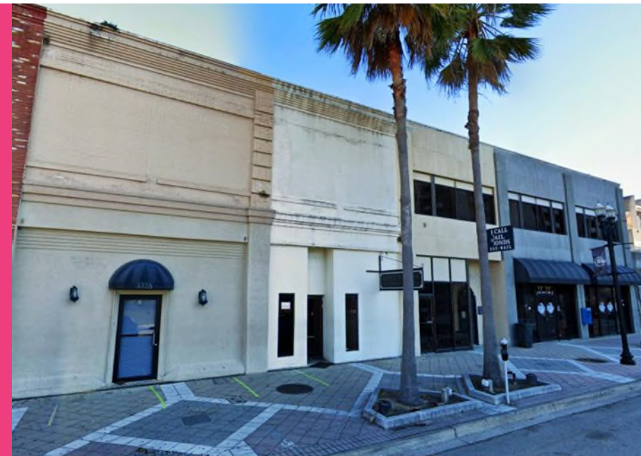
An examples of alterations to pre-war (1909) commercial buildings at 333 E. Bay Street (Duval County). Alterations include replacement of windows and doors and alterations to the openings for the windows and doors.
