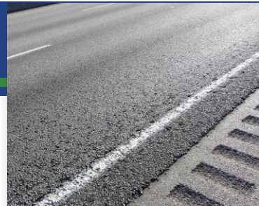
Too Lean - Raveling
