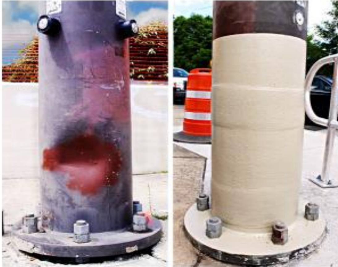
This utility pole (left) was damaged in a collision, but it was successfully repaired (right).
