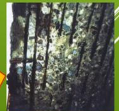
Bottom side of the bridge After 20-year life]
