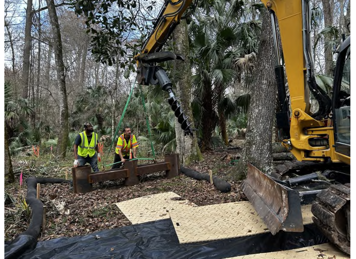
Test pile installation at 8MR1878. Note: geofabric and mats used to help mitigate site disturbance from heavy machinery.
