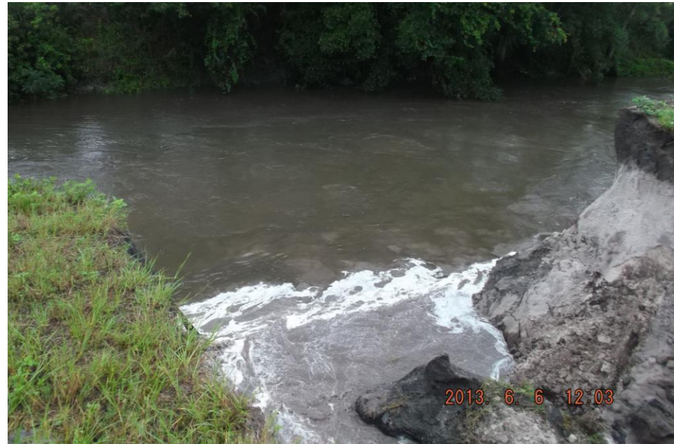
Existing Condition: Erosion
