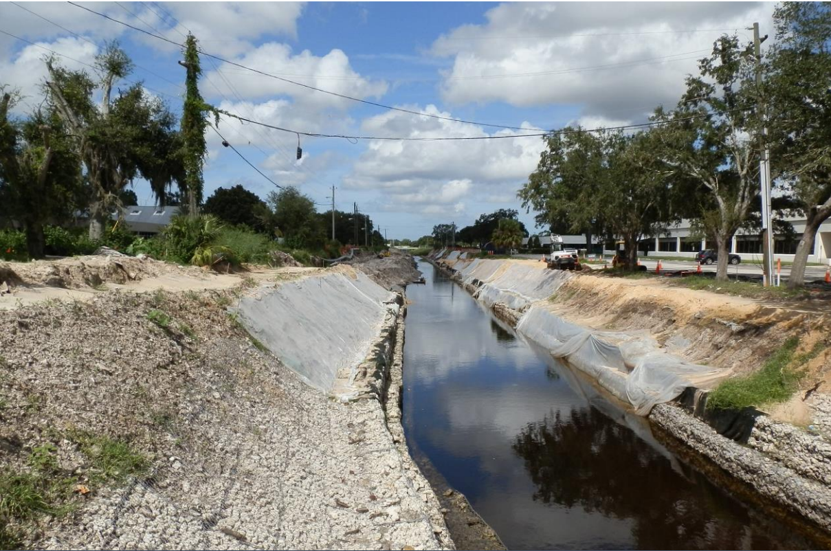
Constructability – Trees in Conflict with Clearing and Grading Work
