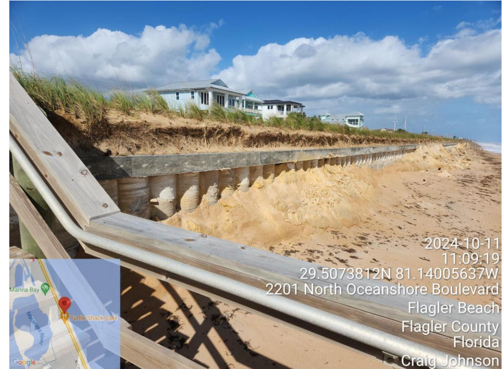
Existing secant wall in Flagler Beach after Hurricane Milton
