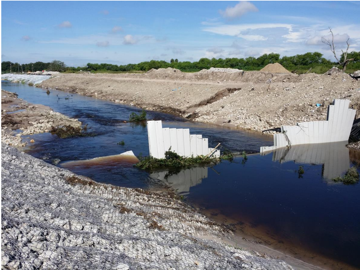
Temporary Drainage – Broken Sheet Pile
