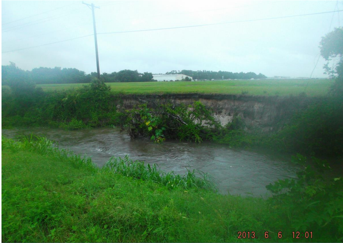
Existing Condition: Erosion uprooted tree fell into Henry Canal
