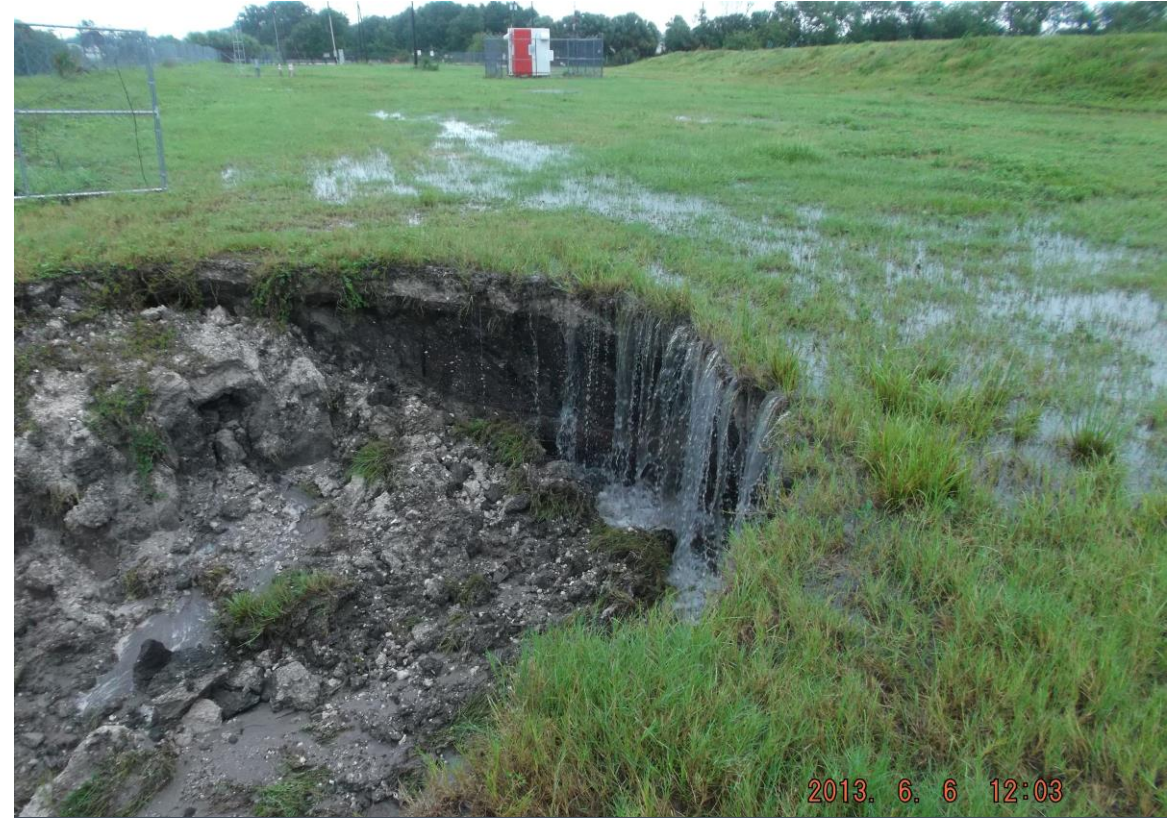
Existing Condition: Erosion caused by sheet flow from rain event
