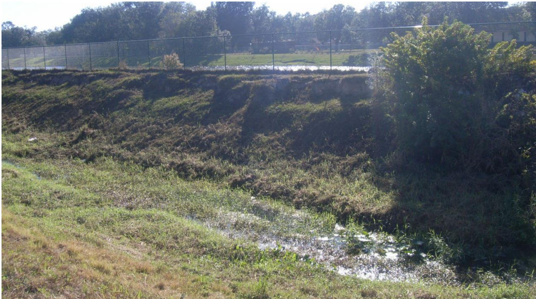
Existing Condition: Erosion at top of bank, sediment in channel bottom
