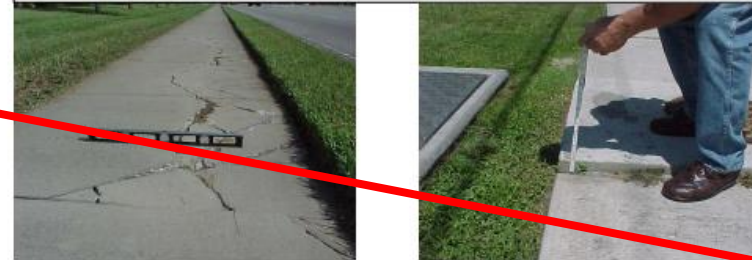
Sidewalk cracking. Measure each horizontal crack greater than \frac{1}{2} inch
