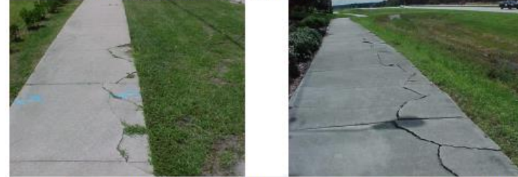
Sidewalk cracking. Measure each horizontal crack greater than \frac{1}{2} inch wide. For MRP purposes, each linear foot of horizontal crack greater than \frac{1}{2} inch equals 1 sq. ft. of crack area. Vertical misalignments greater than \frac{1}{4} inch equals 1 sq. ft. of crack area.
