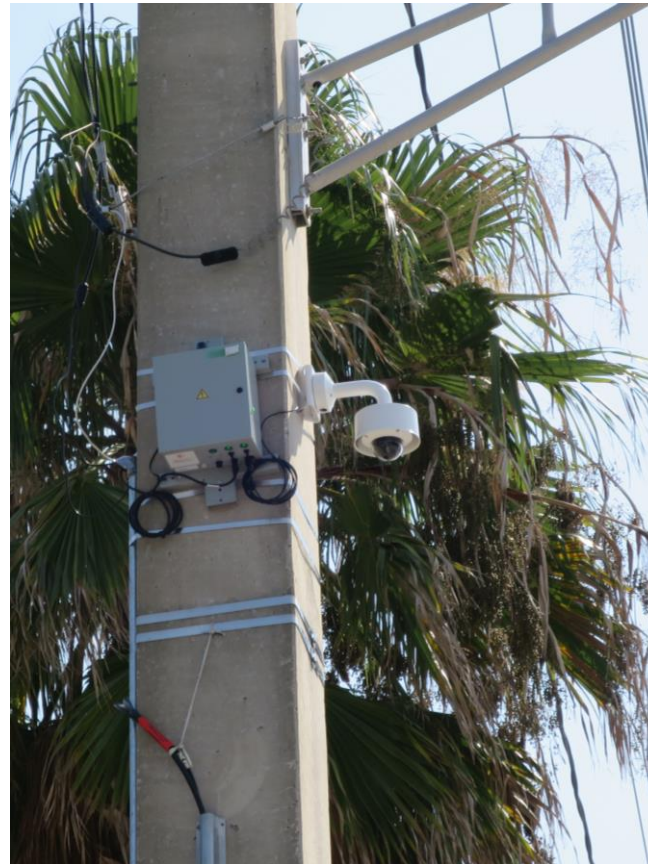
Hardwire, utility pole
