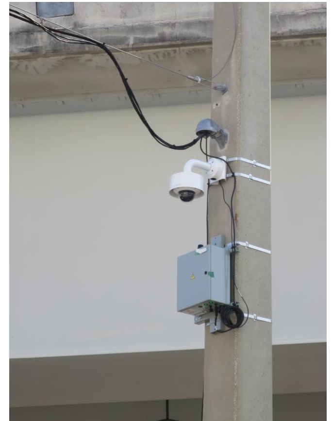
Hardwire, traffic pole
