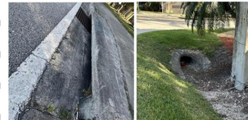
Figure 2-6 Existing Drainage Issues
