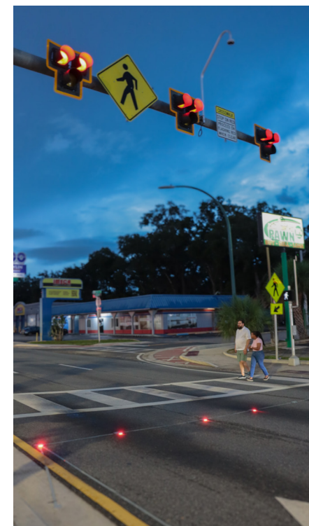
In-pavement warning lights
