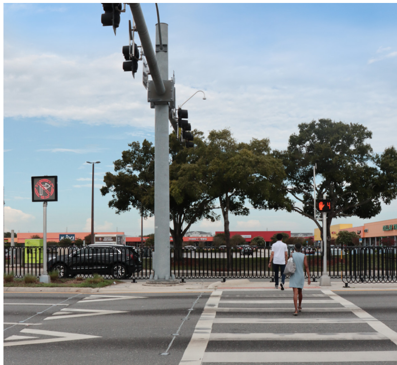
Side street No Right Turn blank-out signs when PHBs activated
